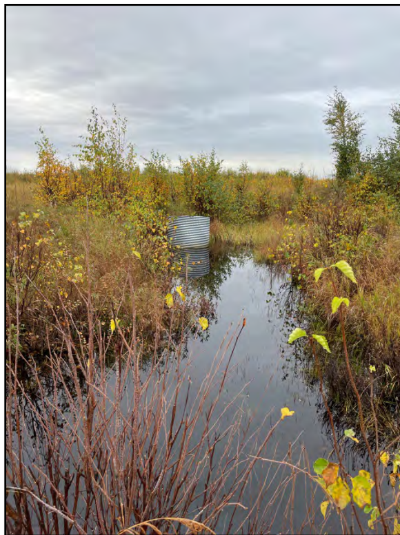
Photograph 2: Drainage channel and large upright culvert near center of Project area, view south
