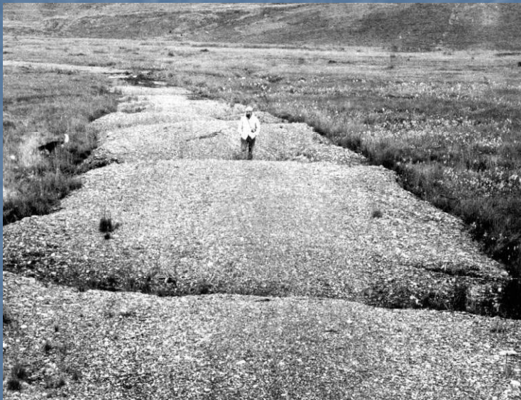
August 1958 – Gravel road near Umiat, showing severe differential subsidence caused by thawing of ice-wedge polygons in permafrost. (Figure 25, U.S. Geological Survey Professional paper 678 – Ferrians, Kachadoorian, and Greene, 1969)
