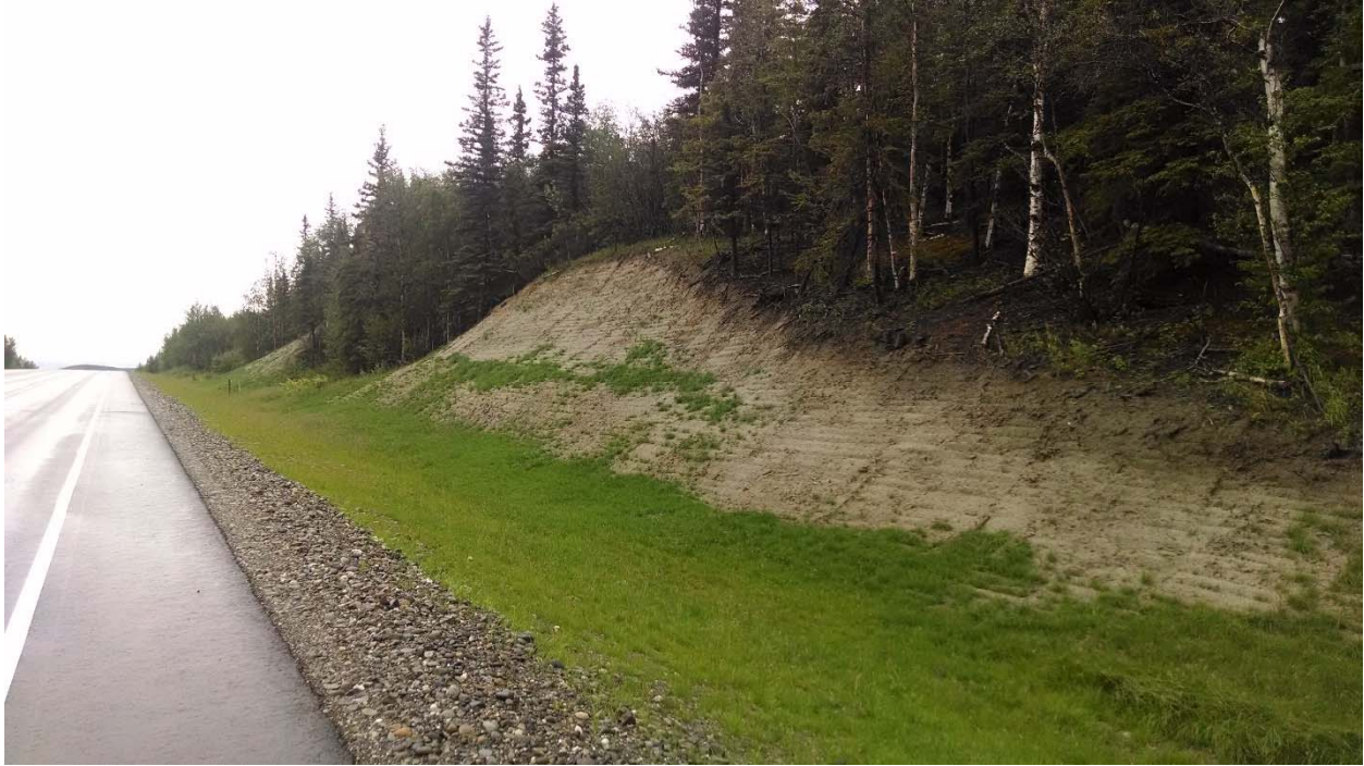
Figure 2-7: Class C soil slope: New soil cut is performing well and is not unstable at this time. Add to database only if instability develops. Parks Hwy MP 257.2
