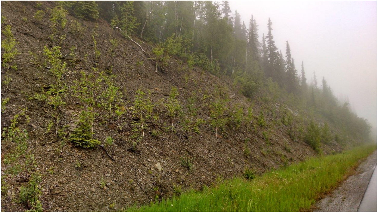
Figure 2-5: Class B rock slope. The slope is relatively well vegetated, indicating a low level of activity, but the ditch is narrow in comparison to the slope height. Parks Hwy MP 338.7.
