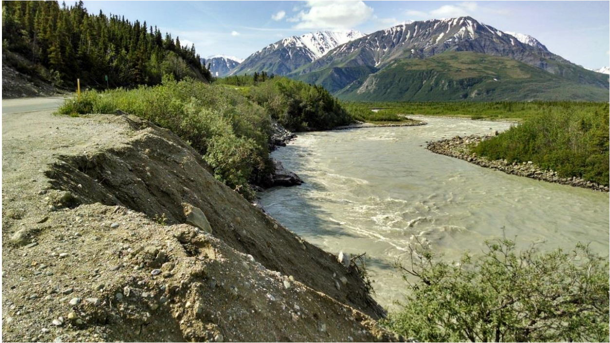
Figure 2-7: Class A slope. Alluvial material comprising the shoulder of roadway is actively being eroded by river action. Armor stone is visible in the distance along portions of the side slope. Richardson Hwy MP 226.
