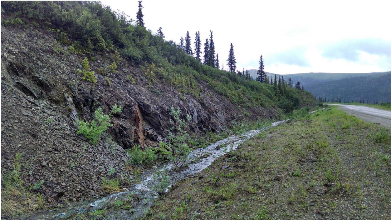
Figure 2-2: Class B rock slope. The slope does not pose a safety concern, but the consequence of rockfall events blocking the ditch and culverts, leading to sheet flow over the road, warrants inclusion into the database. Steese Hwy MP 86.5.
