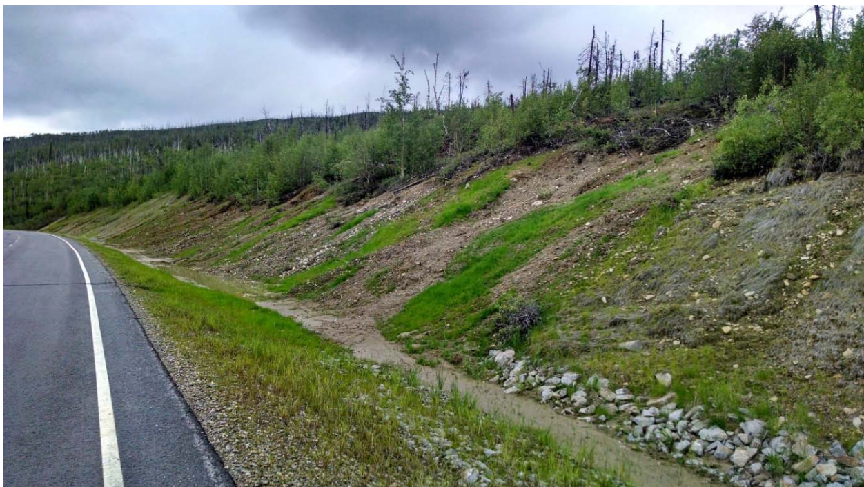
Figure 2-6: Class B soil slope. Short soil cut exhibiting thawing permafrost. Site poses minimal safety risks, but appears to require ongoing minor maintenance attention to maintain the roadside ditch. Steese Hwy MP 68.4.
