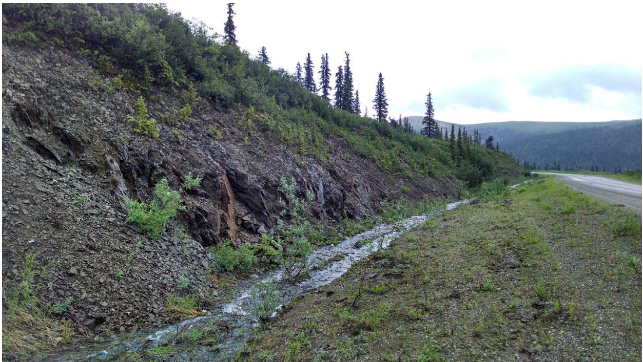
Figure 2-4: Class B rock slope. The slope does not pose a safety concern, but the consequence of rockfall events blocking the ditch and culverts, leading to sheet flow over the road, warrants inclusion into the database. Steese Hwy MP 86.5.
