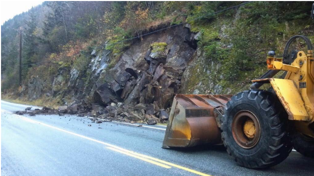
Figure 2-1: Class A rock slope due to adverse geologic character, activity levels, and insufficient ditch catchment. Klondike Hwy MP 3.9.
