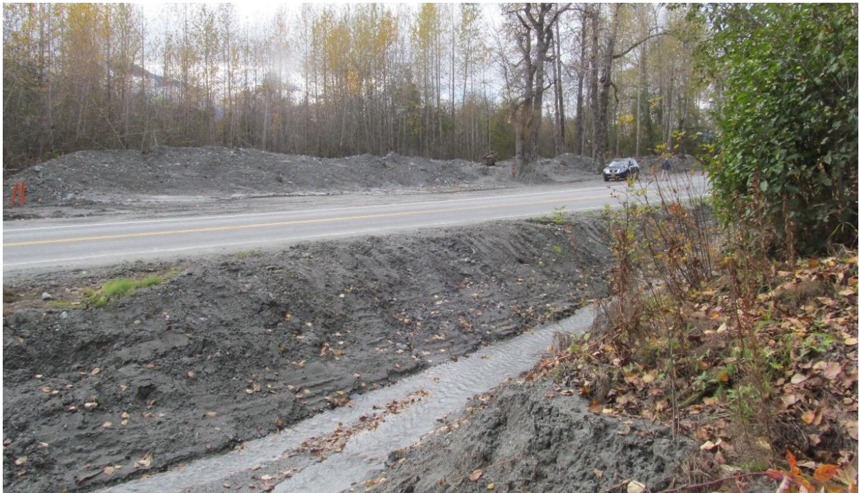
Figure 2-6: Class A slope. Debris flow deposits cleared from roadway. Emergency maintenance frequently required to restore use of the roadway. Haines Hwy MP 19.5.
