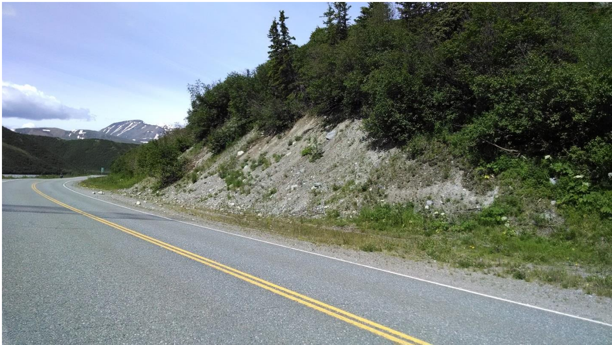
Figure 2-2: Class A slope due to active rock deposition into the ditch, shoulder, and/or travel lane. Road curvature and moderate decision sight distance also contributes to the overall risk. Richardson Hwy MP 209.9.
