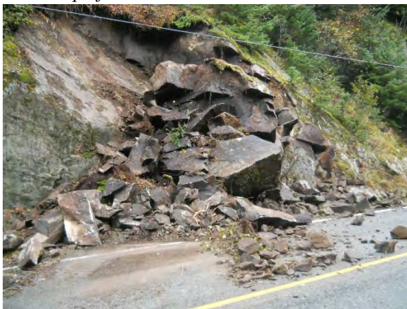
Rock slope failure near MP 2.27
