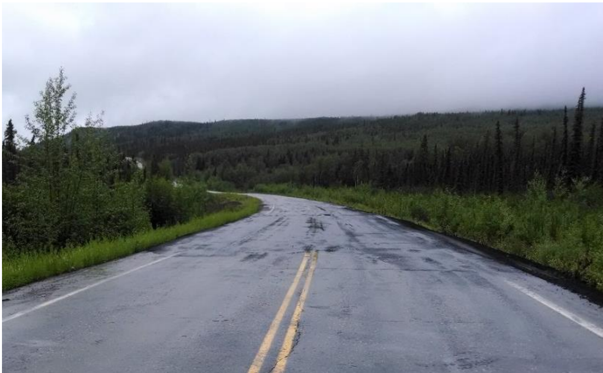
Figure 2-4: Class A soil embankment. Full width roadway patch, with roadway exhibiting wavy, uneven pavement surface associated with continuing thaw-unstable deformation. Elliott Hwy MP 66.4.
