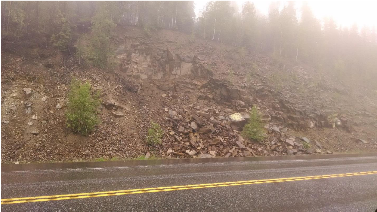
Figure 2-3: Class A slope. The rockfall activity and unmitigated geologic structure require a detailed rating even though a relatively large ditch is present. Parks Highway, MP 344.9.
