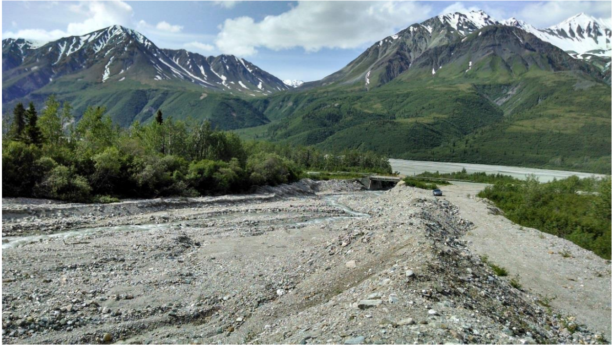
Figure 2-5: Class A slope. Debris flow with containment berms. Regular maintenance required to maintain road. Whistler Ck., Richardson Hwy MP 223.
