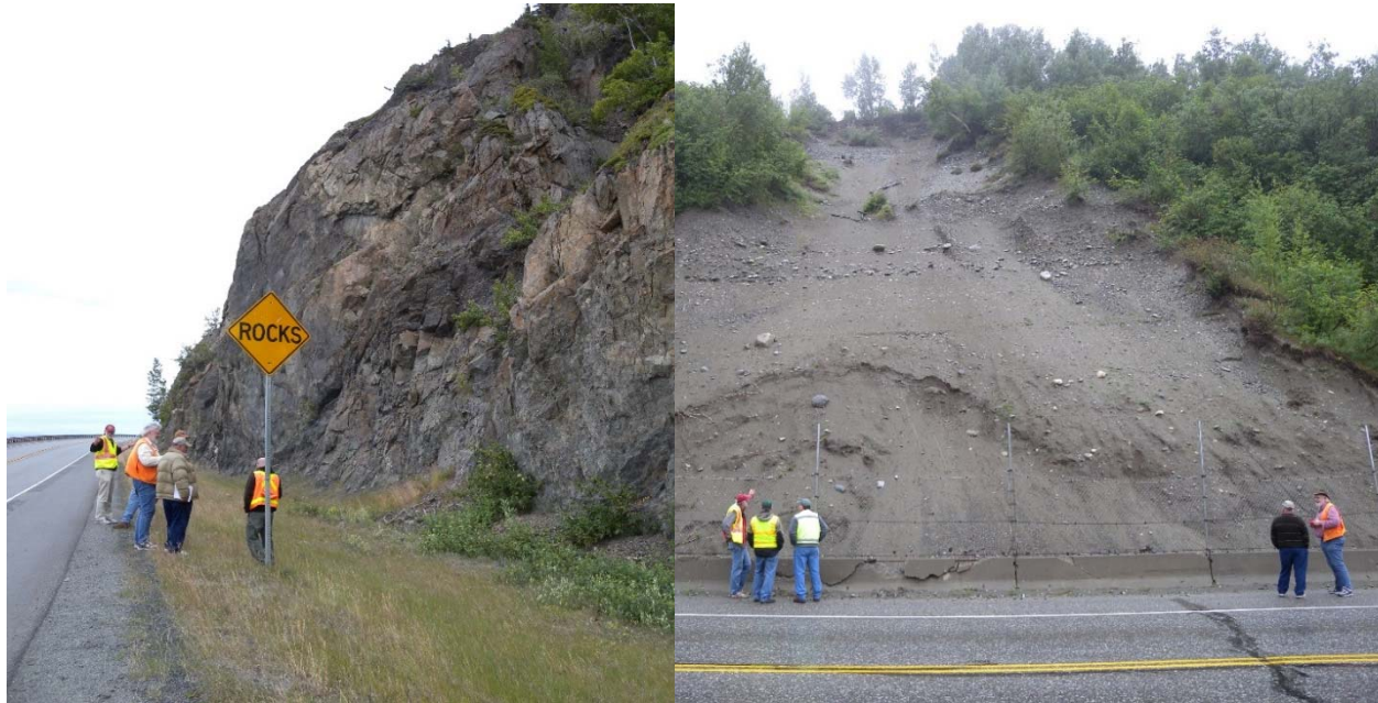
Figure 3-1: Evaluation of rock cuts (Seward Highway shown), soil slopes, and past mitigation work (Glenn Highway shown) during field training and assessment of Phase II rating criteria.
