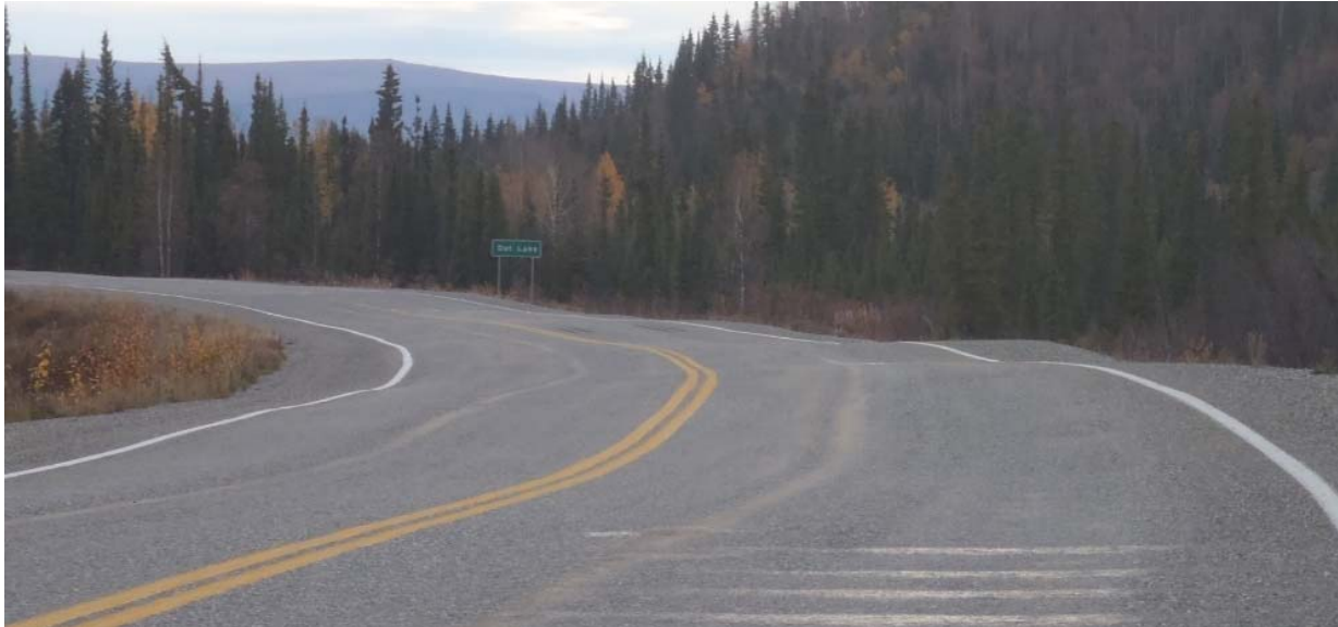
Figure 2-5: Class A soil embankment. Roadway surface exhibiting thaw-unstable settlement with an uneven pavement surface. Alaska Hwy MP 1361.9.
