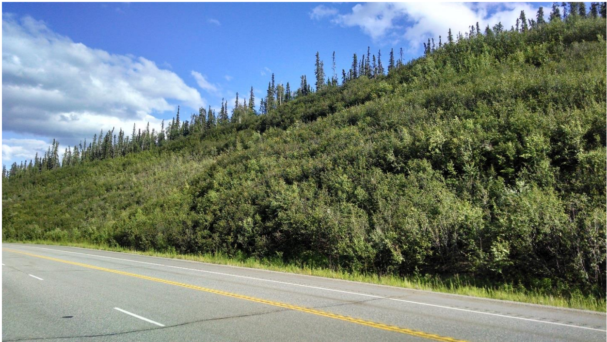
Figure 2-6: Class C rock slope. Typically, such a tall and long cut would be an "A" or "B" slope, but the heavy vegetation indicates exceptionally low activity and high stability. Parks Hwy MP 339.6.
