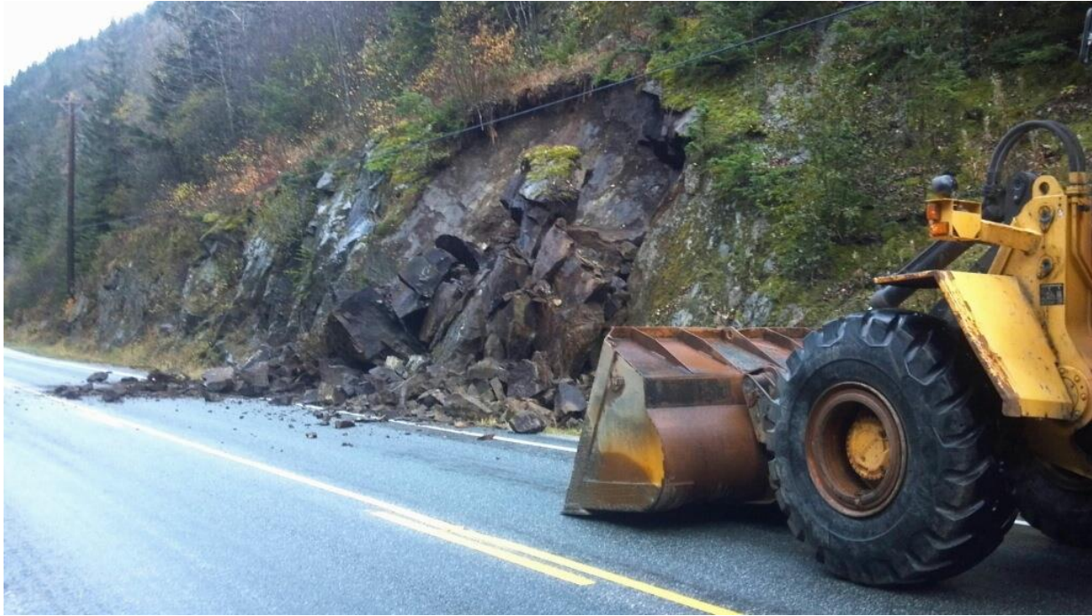
Figure 2-1: Class A rock slope due to adverse geologic character, activity levels, and insufficient ditch catchment. Klondike Hwy MP 3.9.
