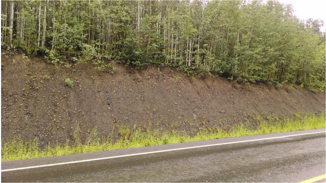
Figure 2-9: Class B soil cut. Relatively small ditch and semi-active raveling/erosion will necessitate occasional ditch maintenance with a low possibility of a soil slump reaching the roadway. Elliott Hwy MP 64.3.
