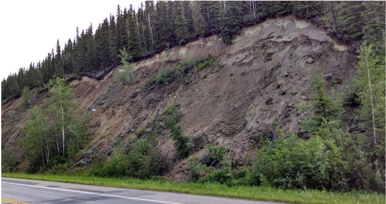
Figure 2-1: Class A soil slope. Slope height and active sloughing warrants a detailed rating. Richardson Hwy MP 328.7.
