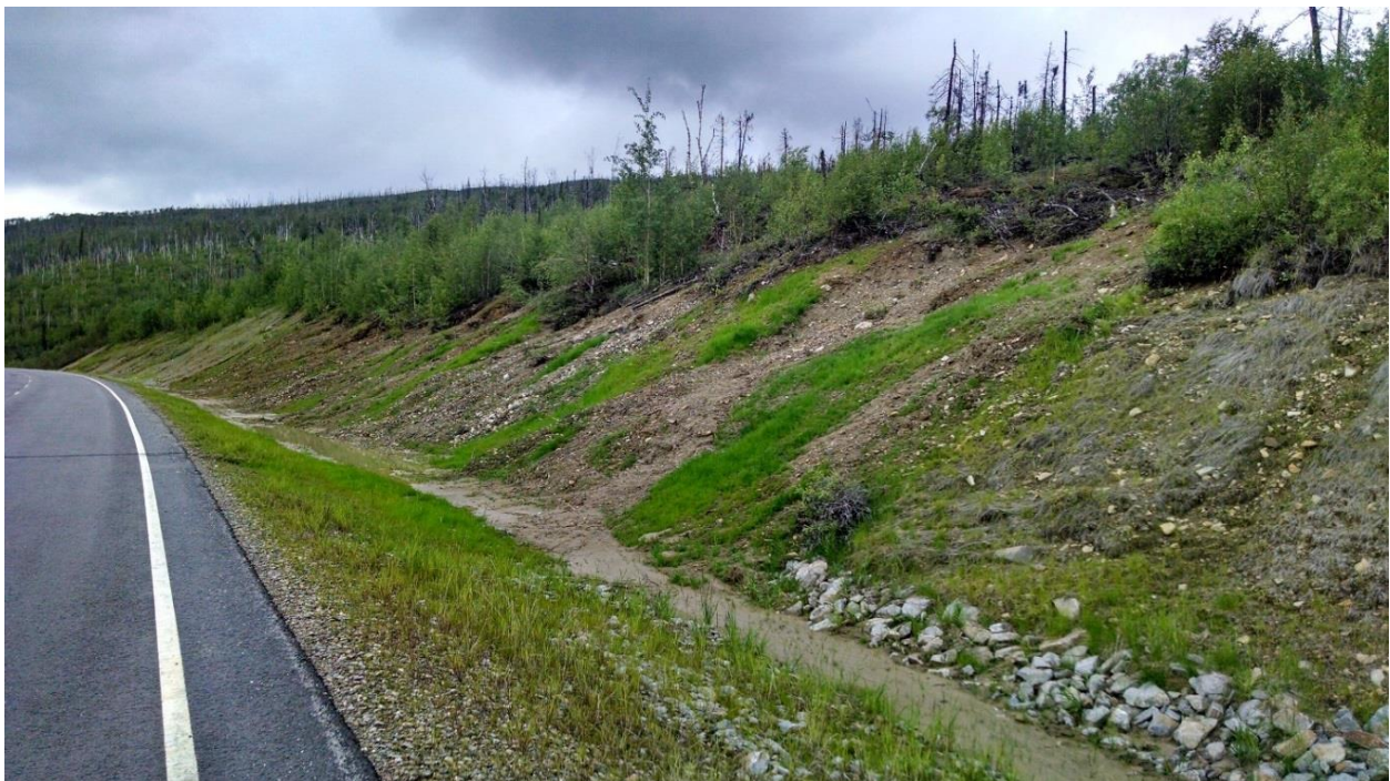
Figure 2-8: Class B soil slope. Short soil cut exhibiting thawing permafrost. Site poses minimal safety risks, but appears to require ongoing minor maintenance attention to maintain the roadside ditch. Steese Hwy MP 68.4.
