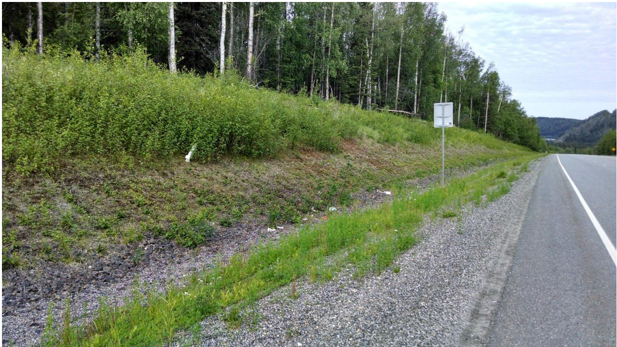
Figure 2-12: Class C soil slope: This slope is performing well and does not show signs of instability. A mossy vegetative mat that has developed across the slope also indicates stability. Richardson Hwy MP 310.3.
