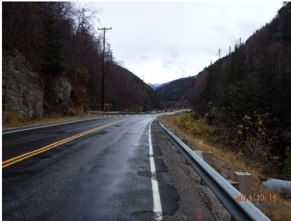
Photographs of embankment distress at MP 2.77
