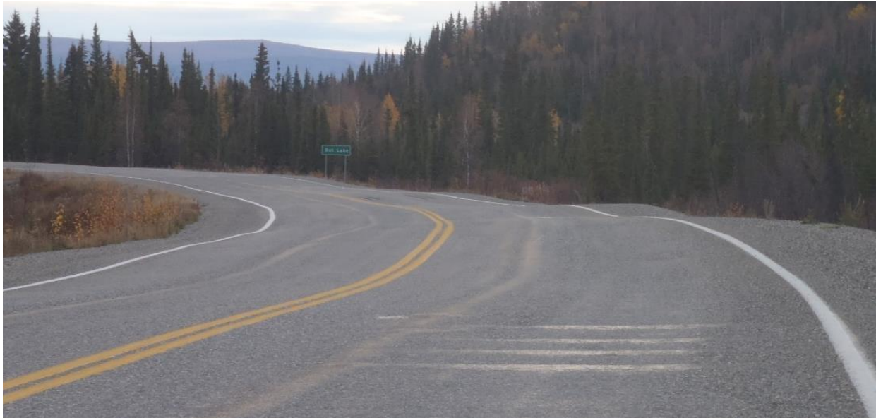
Figure 2-3: Class A soil embankment. Roadway surface exhibiting thaw-unstable settlement with an uneven pavement surface. Alaska Hwy MP 1361.9.
