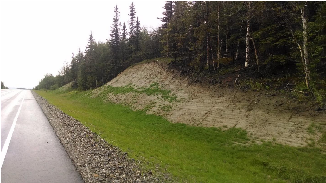
Figure 2-10: Class C soil slope: New soil cut is performing well and is not unstable at this time. Do not include in database unless instability develops. Parks Hwy MP 257.2
