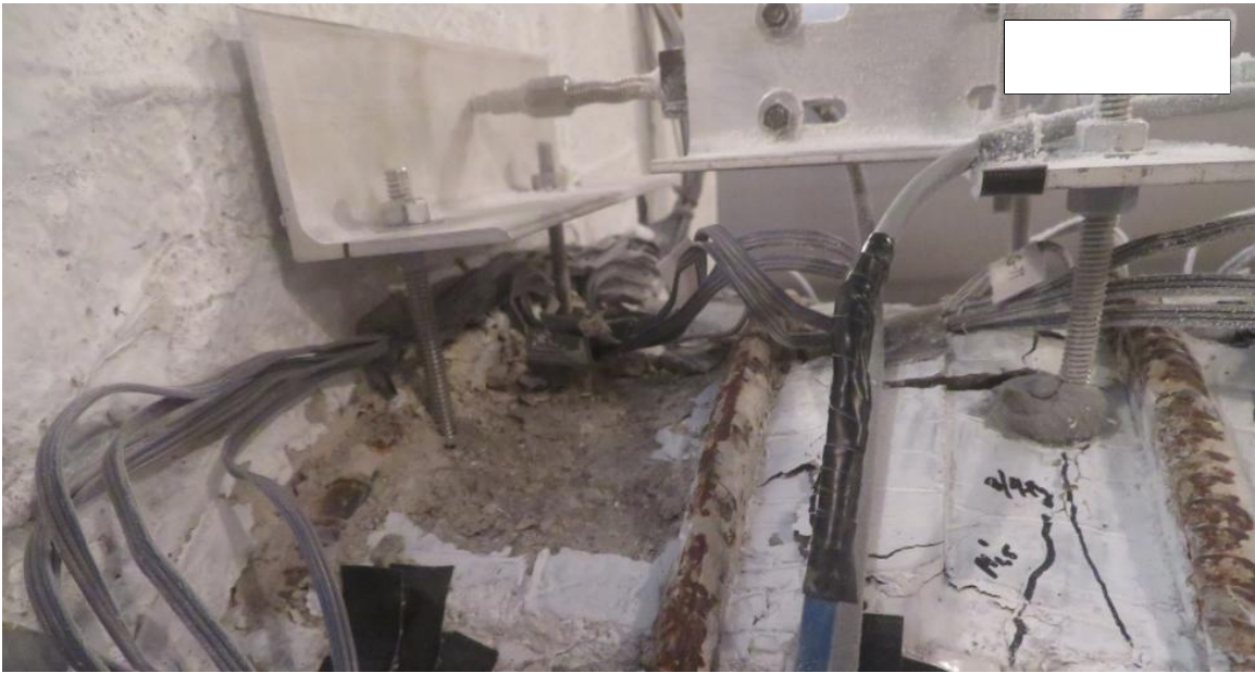
Figure 5-116 First pulling cycle of \mu 4 : Concrete crushing near the base of the column
