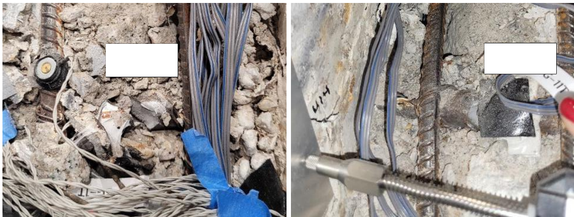
Figure 5-50 First cycle of \mu_6 (pushing): fracture of top bars 1T and 3T
