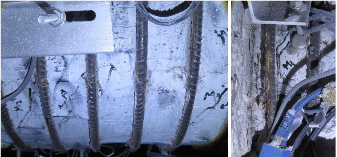
Figure 5-62 First cycle of \mu_3 (pushing). Some hairline shear cracks were observed along the column, and expansion of cracks at the base of the columns
