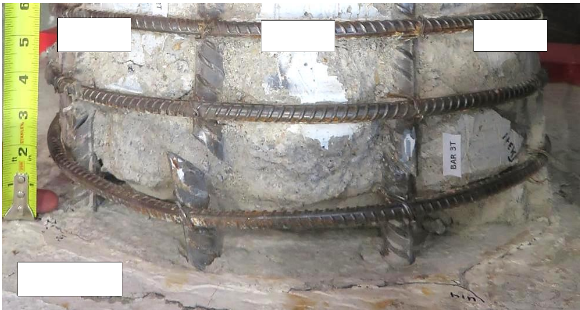
Figure 5-51 Damage at the top of the column along the plastic hinge: Fracture of bars 1T, 2T, and 3T, and concrete core crushing.
