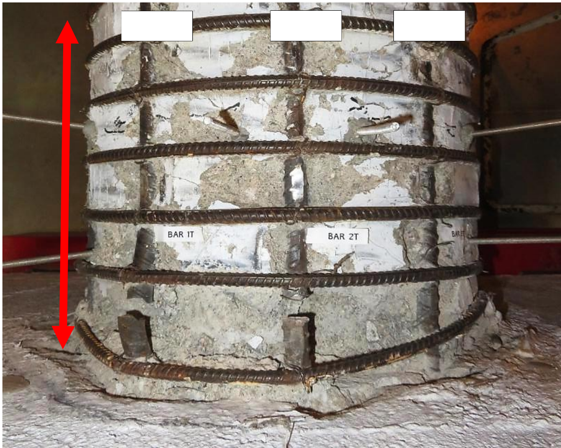
Figure 5-68 Damage at the top of the column along the plastic hinge: Fracture of bars 1T and 2T, and concrete core crushing.
