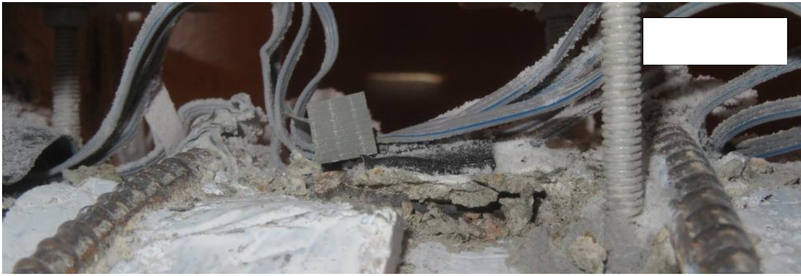
Figure 5-97 Third pulling cycle of \mu 4 : Significant concrete crushing around the longitudinal top extreme bar, 2T
