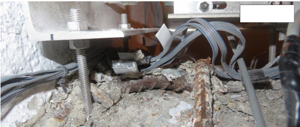
Figure 5-117 Third pulling cycle of \mu 4 : Buckling of top extreme bar 2T
