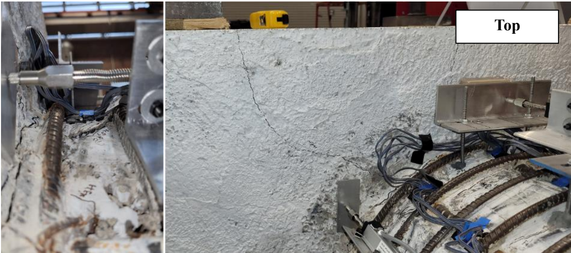
Figure 5-27 First cycle \mu_3 (pushing): Extension of cracks at the base of the column and in the footing.
