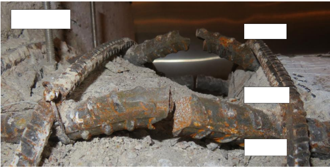
Figure 5-103 Brittle fracture surface of top bars (1T, 2T, and 3T)
