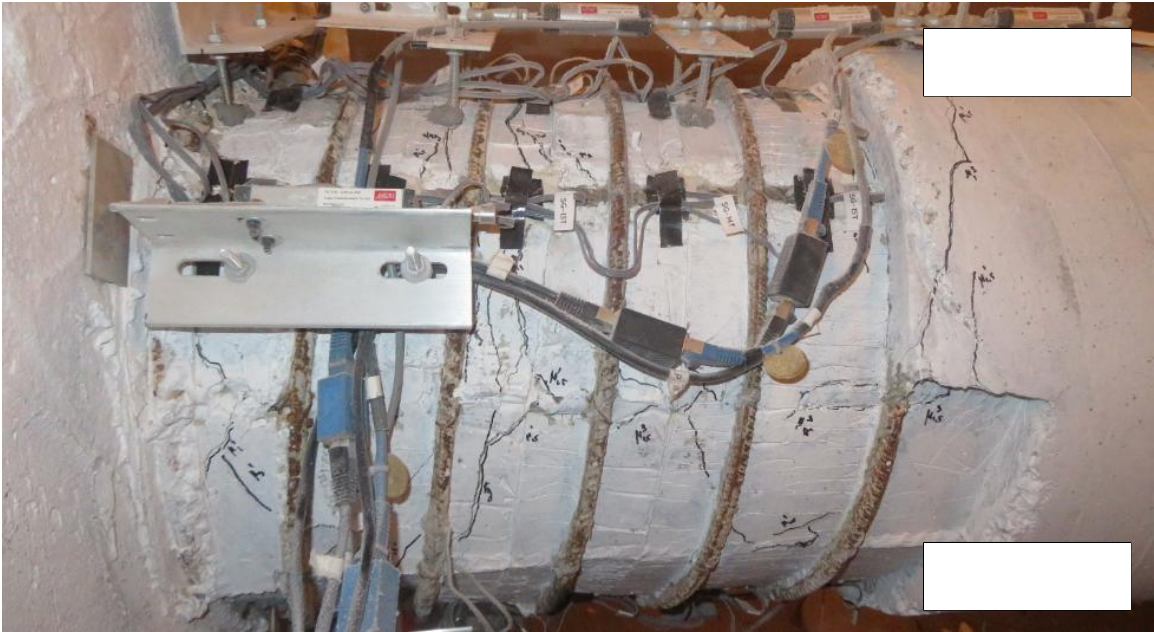
Figure 5-114 Third pushing cycle of \mu 1.5 : Extension of cracks and formation of some shear cracks
