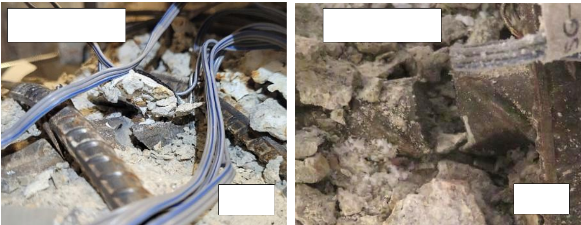
Figure 5-140 Fracture of the top extreme bar in the QST columns, tested at room and low temperatures.
