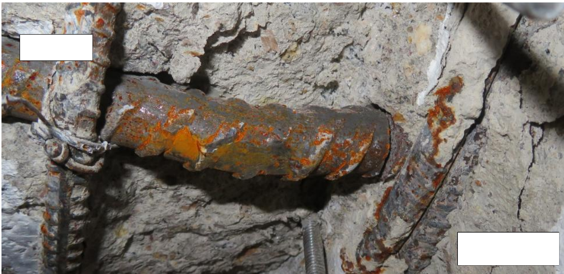
Figure 5-105 Fracture of bar 2B near the base of the column
