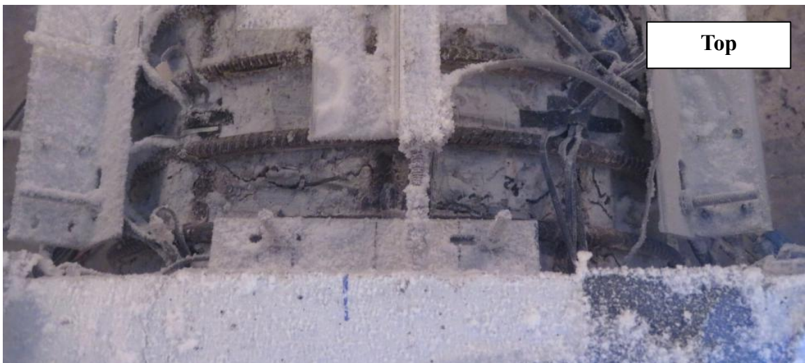
Figure 5-80 Third cycle of \mu_3 (pushing) widening of the perimetral cracks near the base of the column
