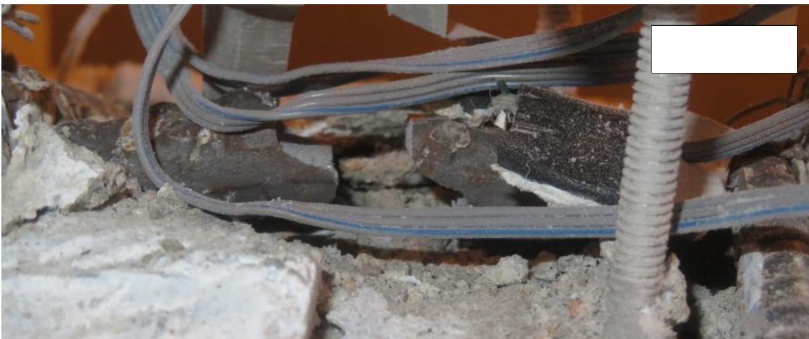
Figure 5-99 Second pushing cycle of \mu 5 : Bar fracture of top extreme bar, 2T
