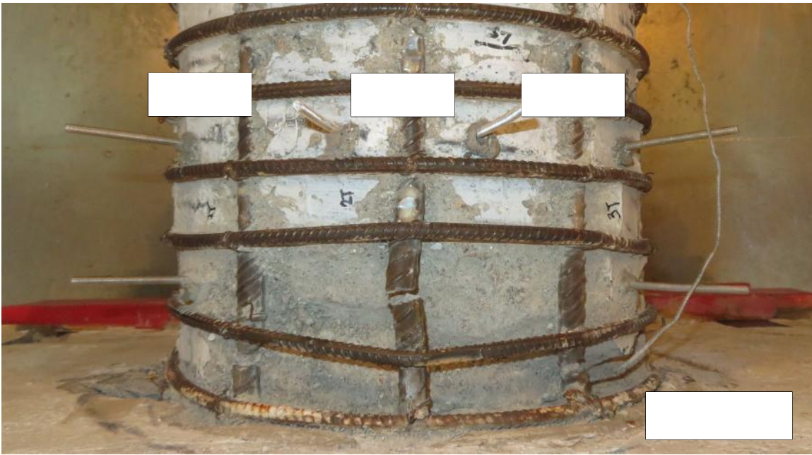
Figure 5-85 Damage at the top of the column along the plastic hinge: Fracture of bars 1T, 2T, and 3T, and concrete core crushing
