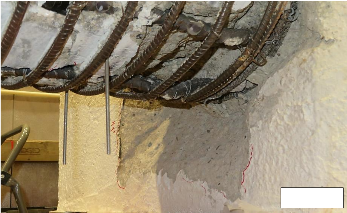
Figure 5-35 Damage at the bottom of the column: Fracture of bar 2B, concrete core crushing, and footing concrete breakout due to stress concentrations on footing support.
