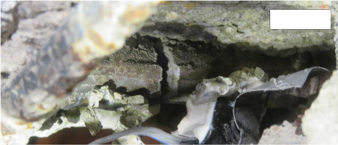
Figure 5-118 First pulling cycle of \mu 5 : Bar fracture of bottom extreme bar 2B
