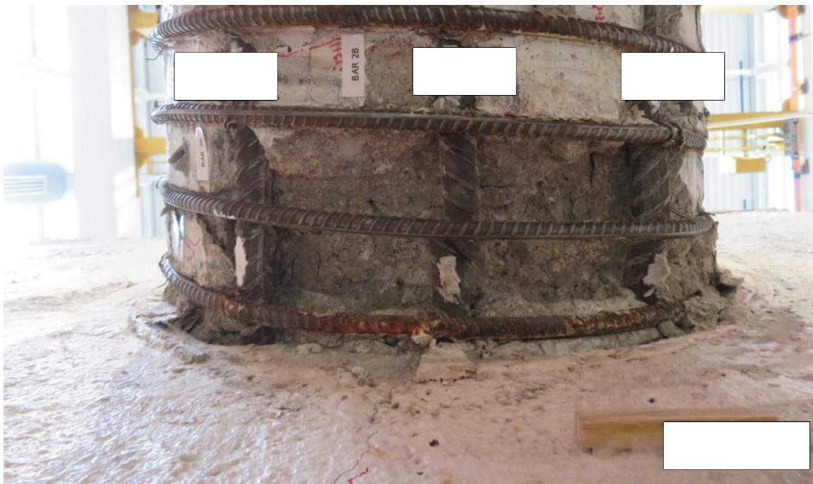
Figure 5-52 Damage at the bottom of the column: Fracture of bar 2B, concrete core crushing.
