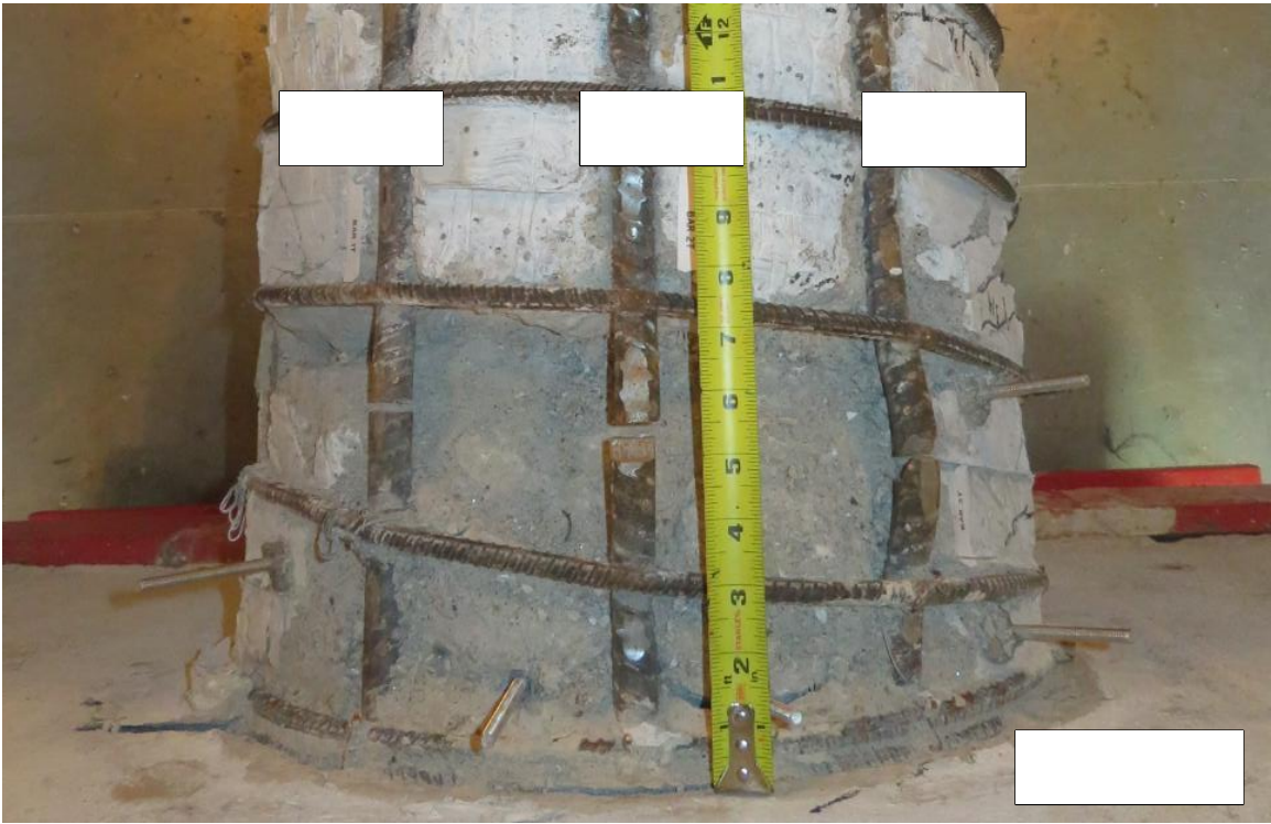
Figure 5-102 Damage at the top of the column along the plastic hinge: Fracture of bars 1T, 2T, and 3T, and concrete core crushing
