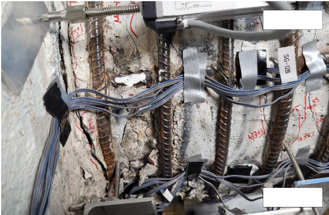
Figure 5-47 Third cycle of \mu_4 (pulling): Cracks are widening at the base of the footing.
