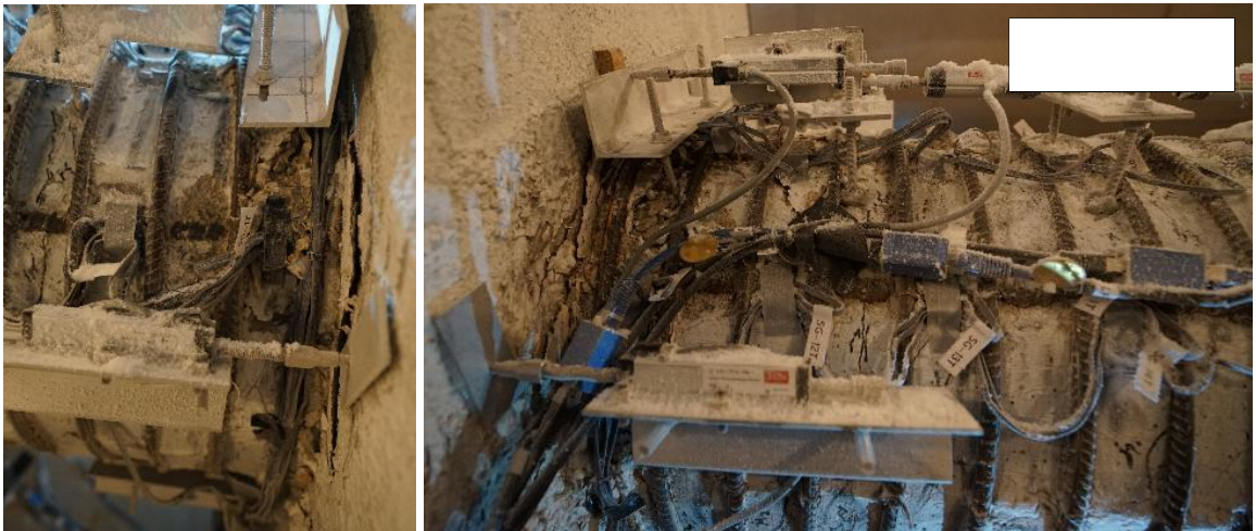
Figure 5-64 First cycle of \mu_5 (pushing). Concrete damage around the longitudinal bars, damage observed in the footing, and thickening of cracks along the plastic hinge length
