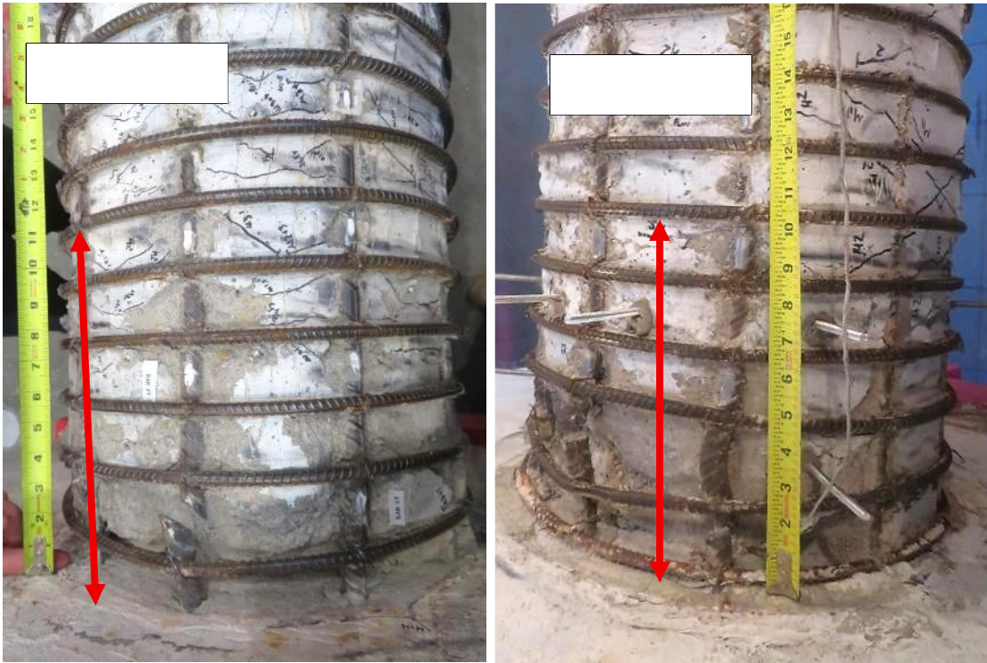
Figure 5-144 Concentration of concrete crushing at the base of the columns
