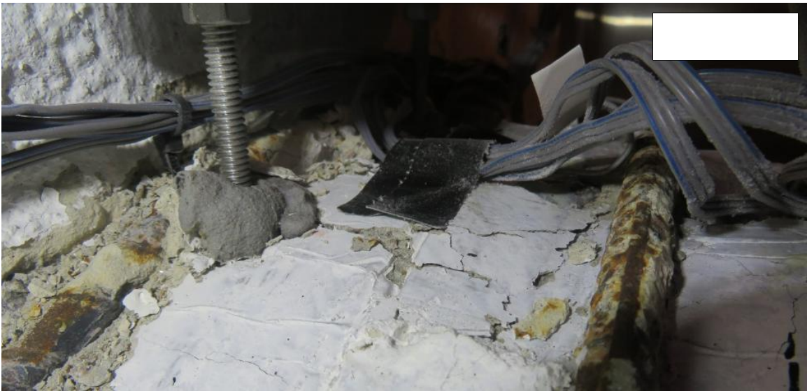
Figure 5-115 Third pulling cycle of \mu 3 : Concrete flaking near the base of the column.
