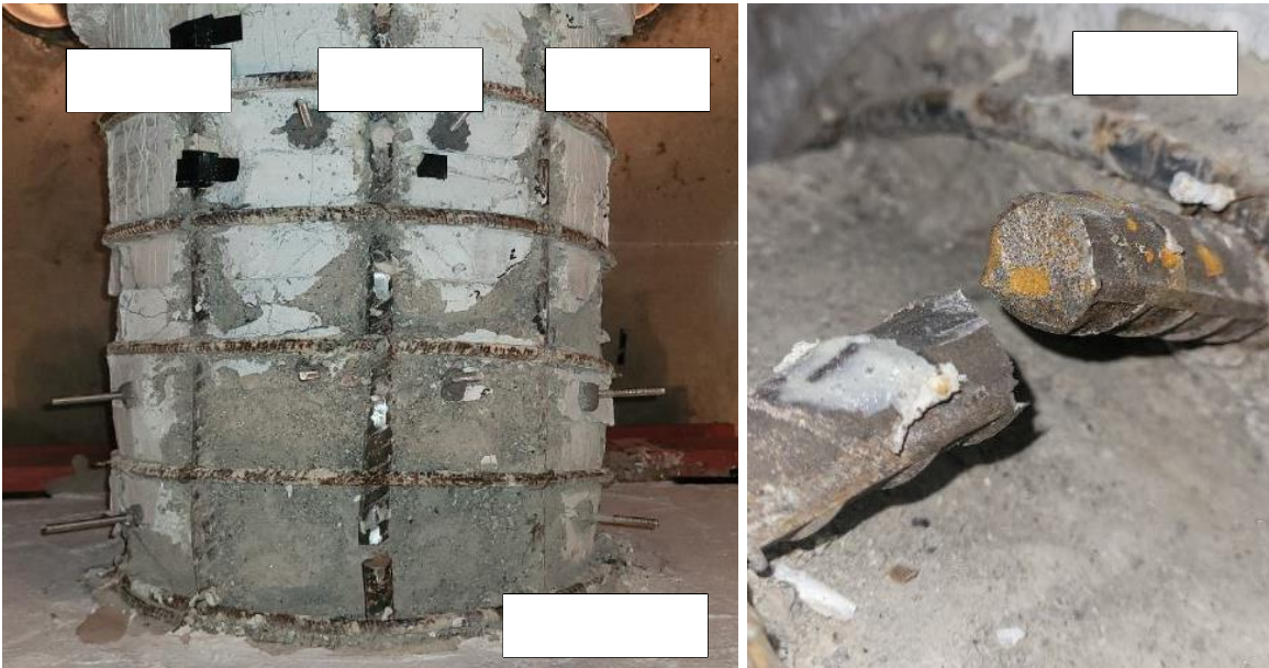
Figure 5-121 Damage at the top of the column along the plastic hinge: Fracture of bar 2T and concrete core crushing
