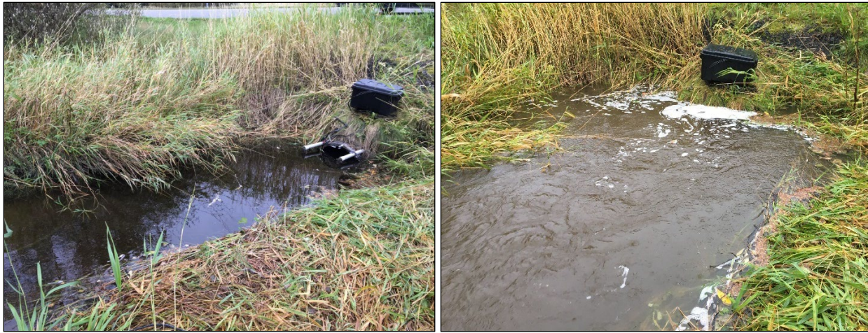
Figure 4.—Egan Drive Creek culvert outlet with PIT tag antenna installed; low flow 9/20/2023 (left), high flow 9/21/2023 (right).
