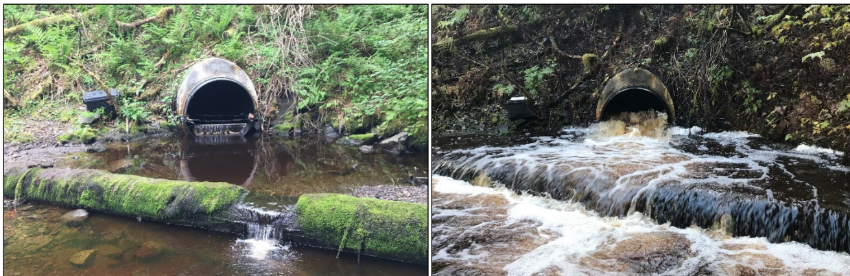
Figure 2.—Ninemile Creek culvert outlet with PIT tag antenna installed; low flow 5/28/2023 (left), high flow 10/19/2023 (right).
