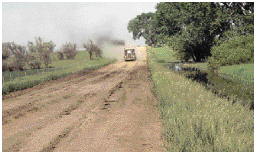
This road has been badly damaged from a heavy haul. It would be useless to begin hauling and placing fresh gravel until the entire roadway has been reshaped.
