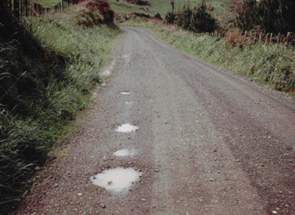
This road located in New Zealand does not have adequate crown to drain water to the roadside. Consequently, potholes form. (Courtesy of Ken Skorseth, SD LTAP)
