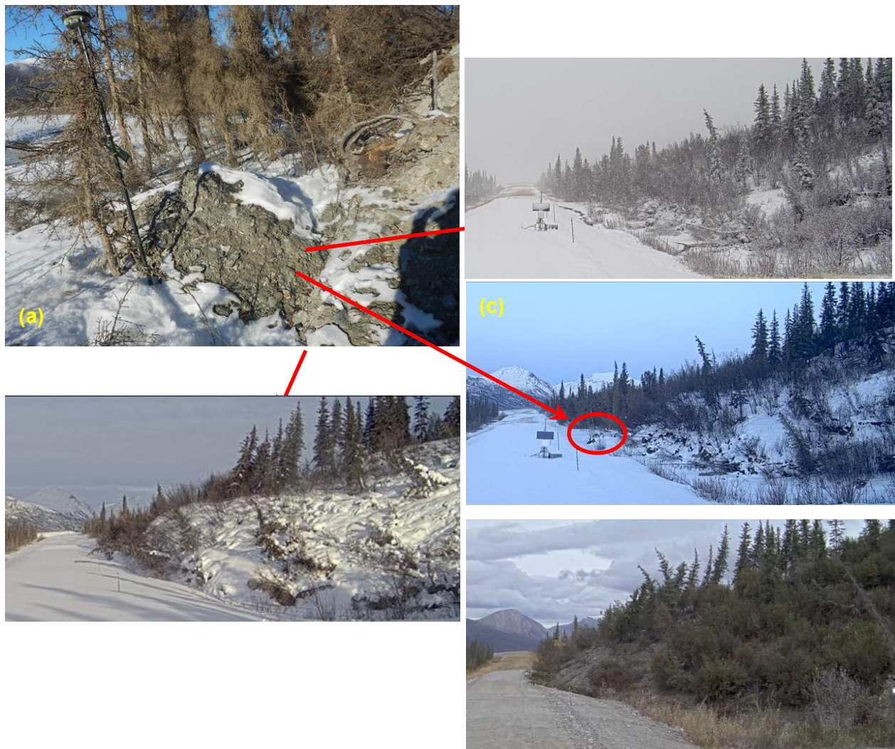
Figure 13. Sequence of deformation at the toe of FDL-A: (a) soil mound noted during a field visit on October 2, 2021; location (red ellipses) of the soil mound in (a) on (b) September 19, 2021 and (c) November 30, 2021; (d) back-tilted trees (red arrow) along toe on March 1, 2023; (e) slumping of previous back-tilted trees (red arrow) on September 9, 2023.
