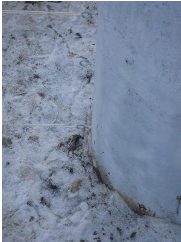
Figure 2.26: Soil crack at 150 kips, January test.
