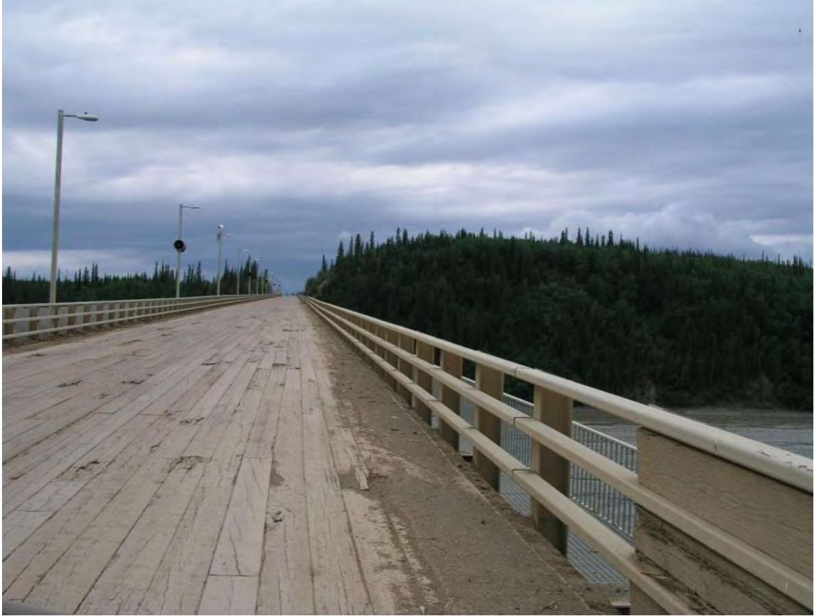
Figure 1.2 Timber deck at the end of its service life.
