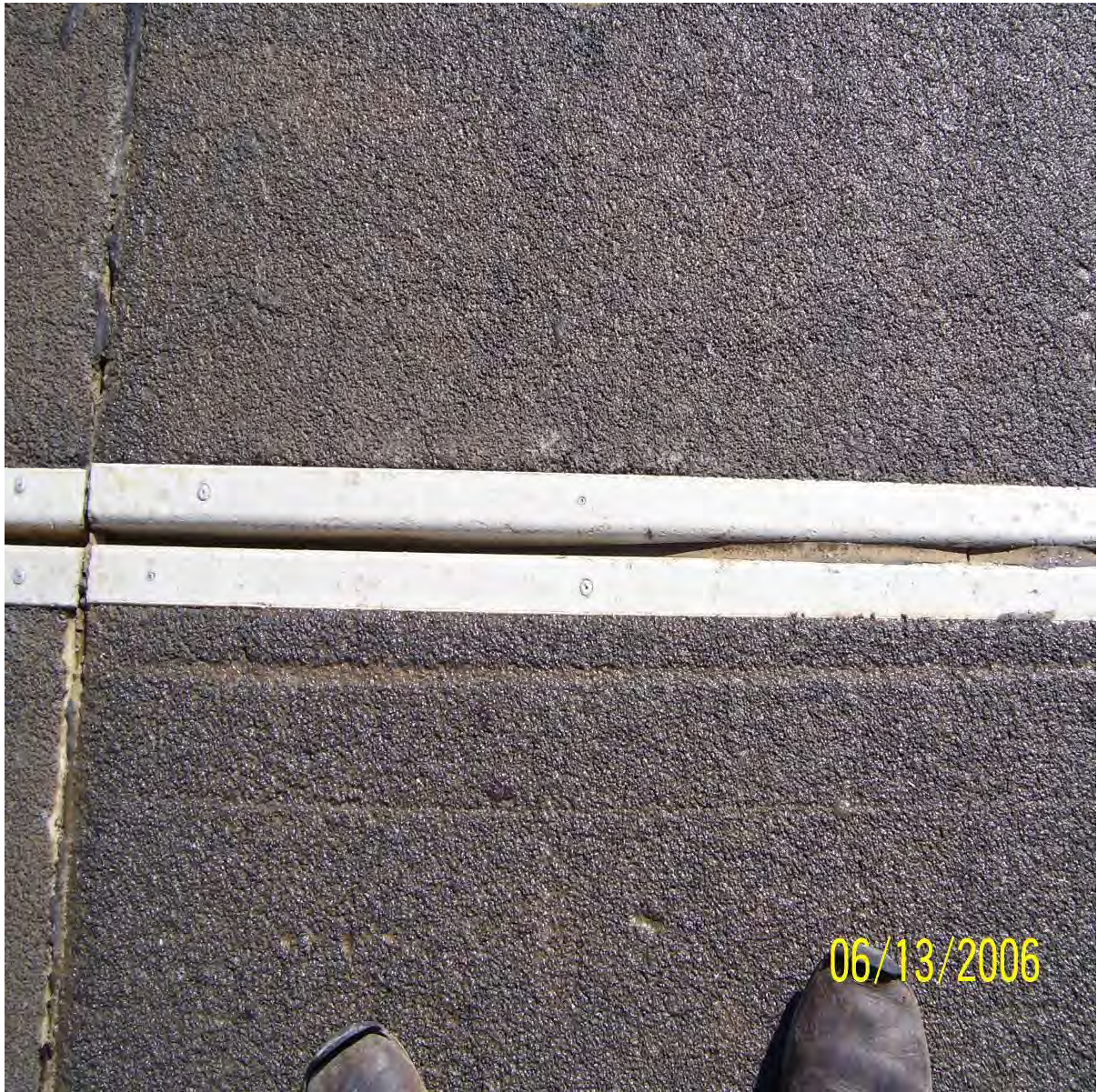
Figure B.13 Transonite edge strip with missing pop rivets.
