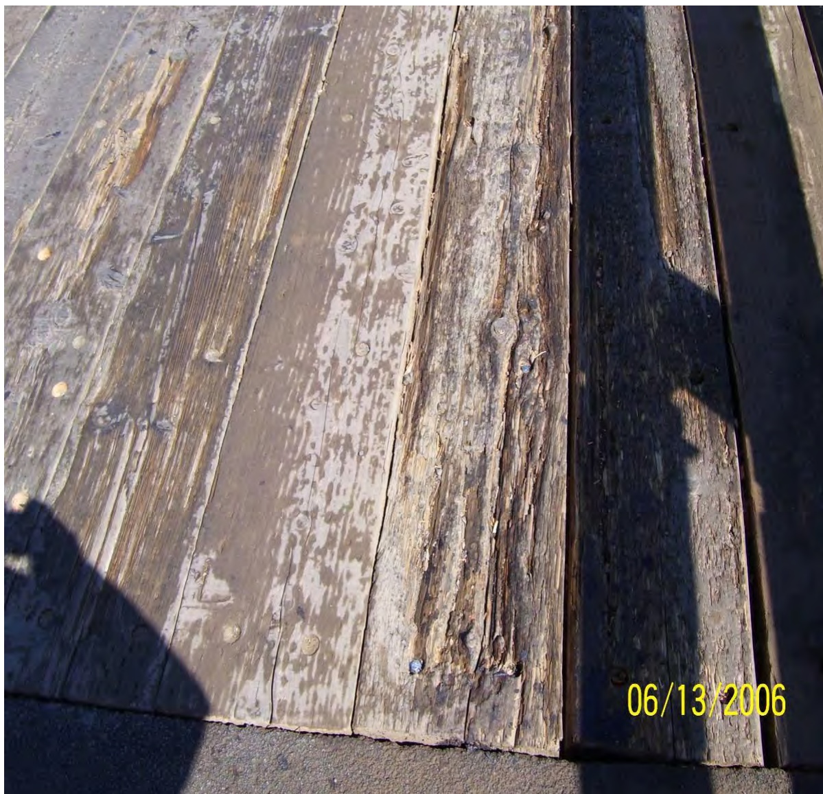
Figure B.3 Decay in the top of the wearing surface.
