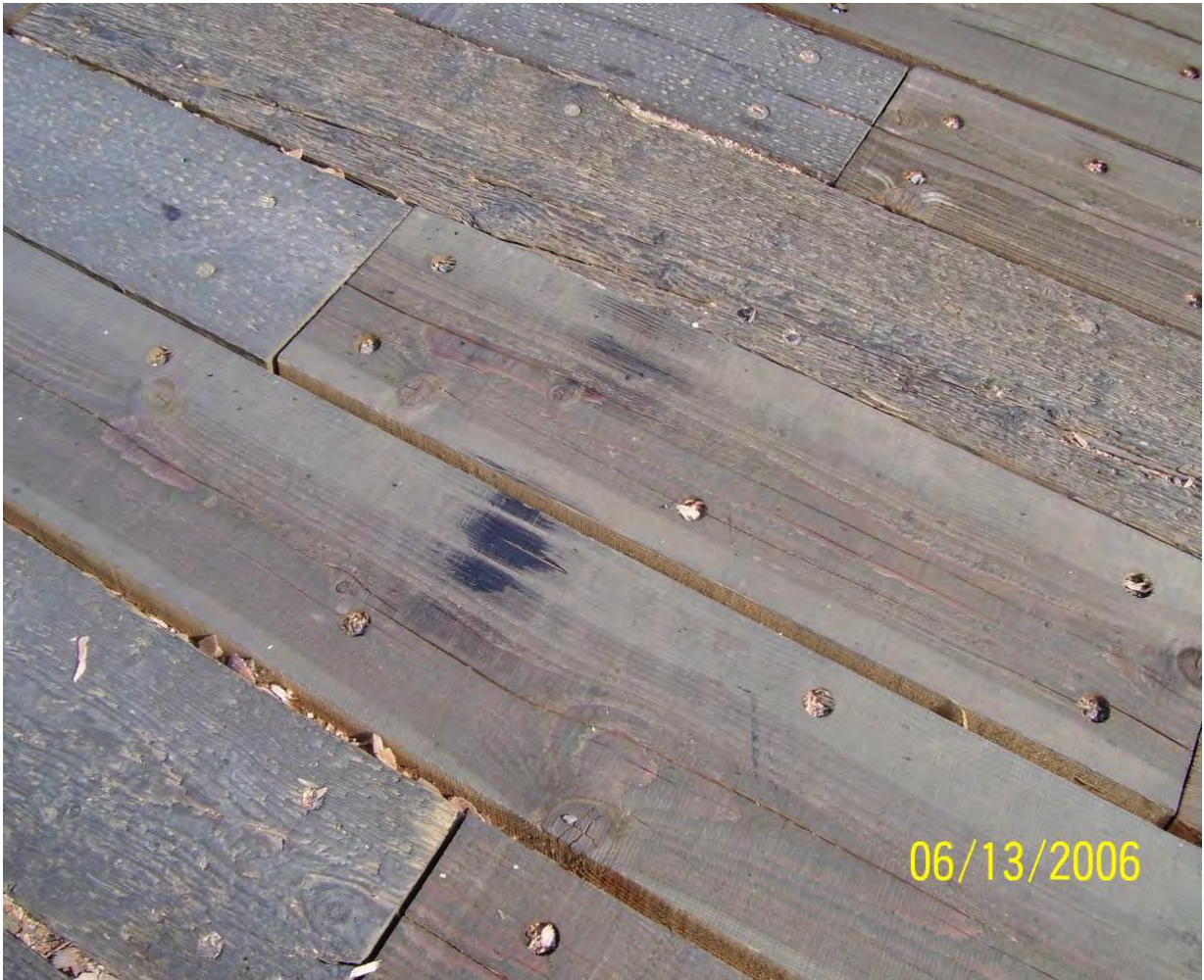
Figure B.4 Rubber tire marks caused by loss of traction.
