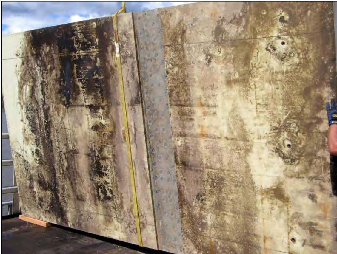
Figure C.5 Transonite panel, bottom side inspection.
