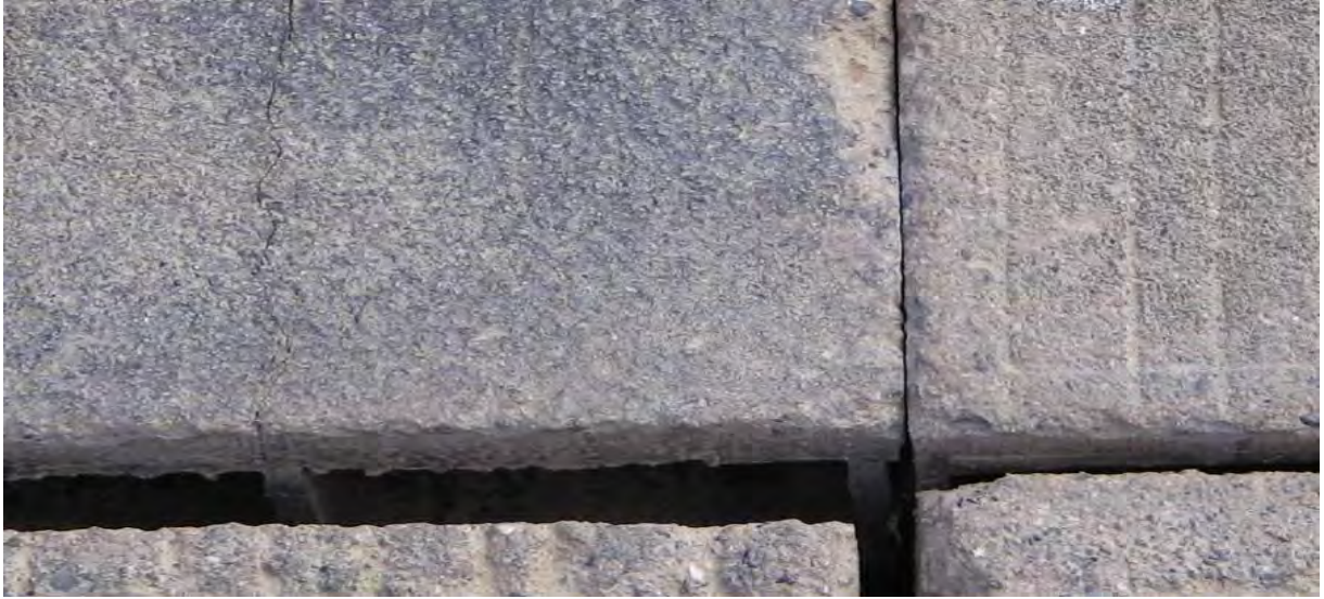
Figure B.23 Prodeck 4 test panel: Cracks propagated from the fiberglass.
