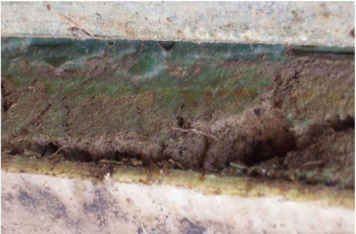
Figure B.15 Cracked sealer and foam on the Transonite panel.
