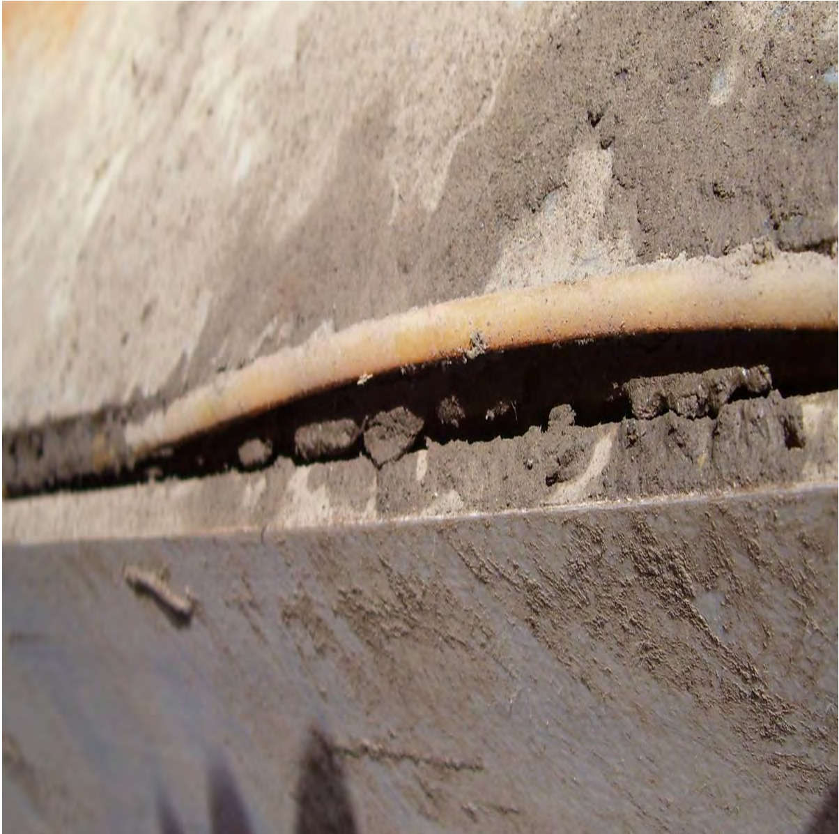
Figure B.14 Leaky seal under the Transonite panel.
