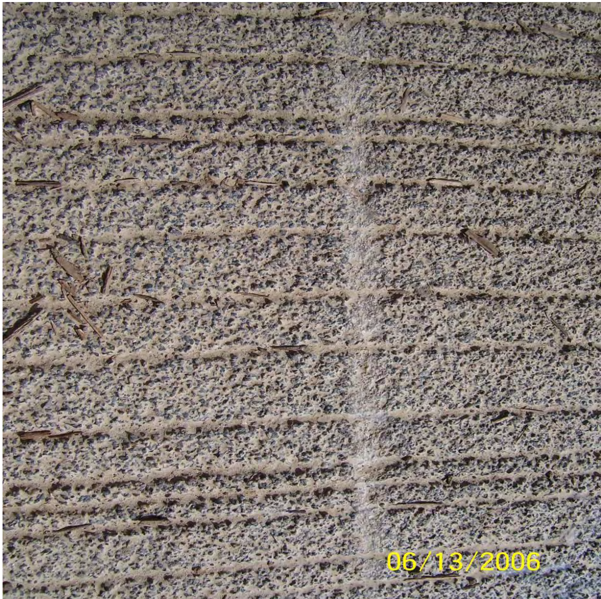
Figure B.22 Grader scratch to the wearing surface on the Prodeck test panel.
