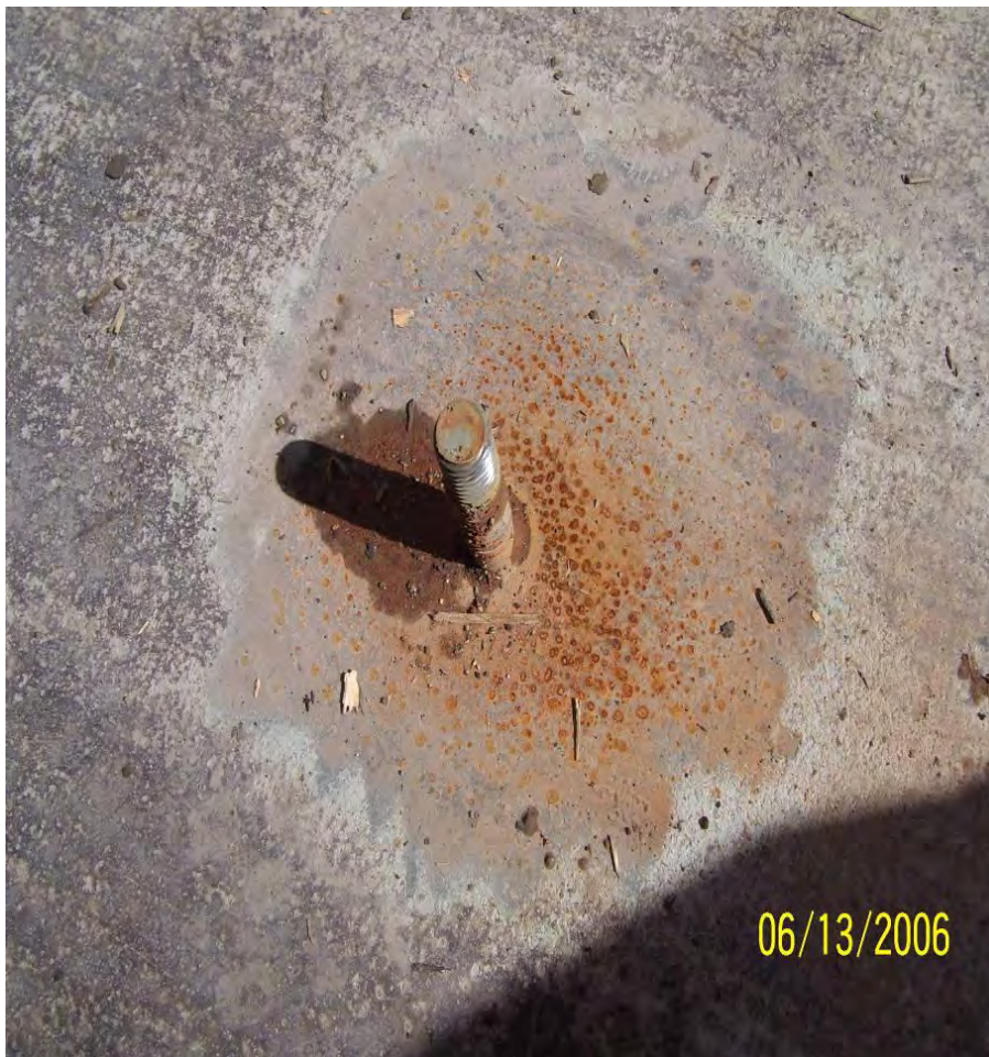
Figure B.21 Deck rust at a welded stud; loss of anticorrosion coating.
