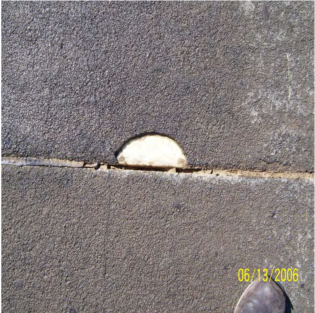
Figure B.12 Possible delamination caused by a bolt in the splice plate.
