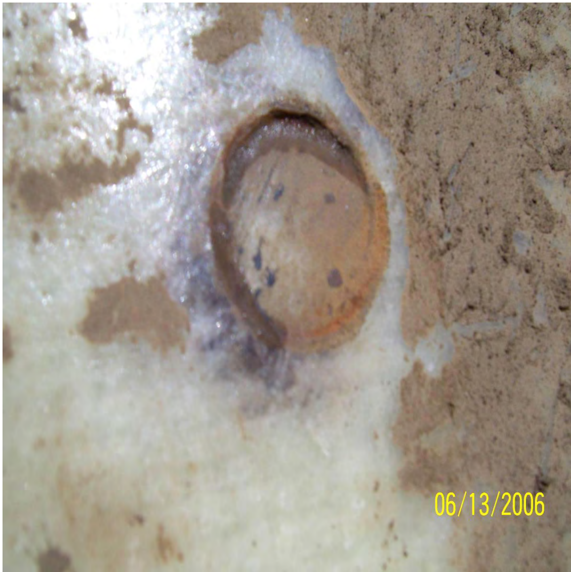
Figure B.20 Punctured bottom surface of the Transonite test panel.
