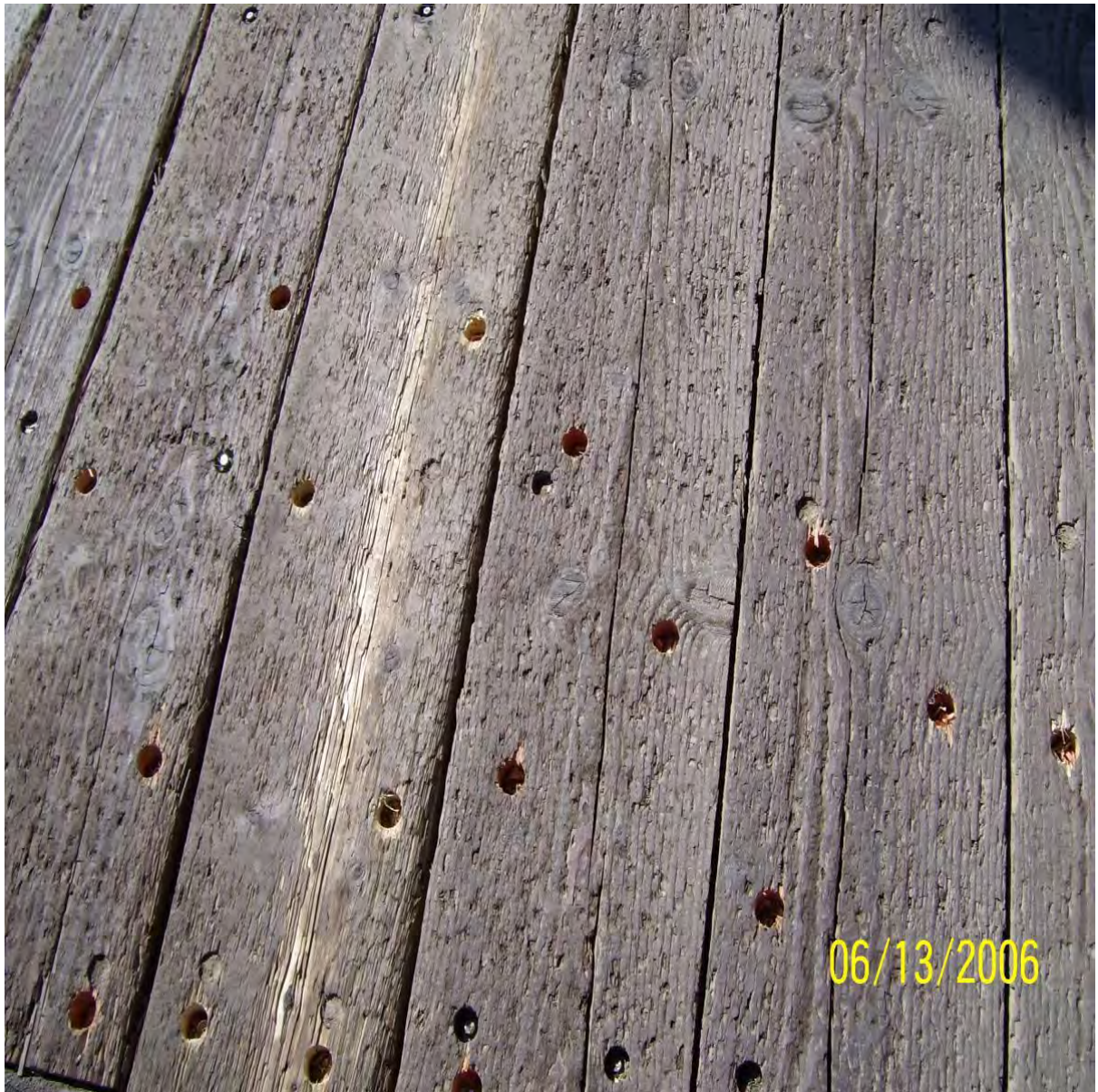
Figure B.2 Surface wear damage caused by tire chains.
