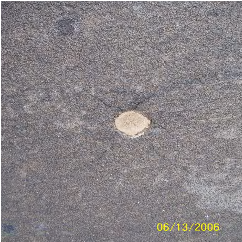
Figure B.11 Cracks around attachment hole: Transonite wearing surface.
