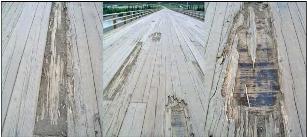
Figure C.1 Timber wearing surface, months before it was replaced.
