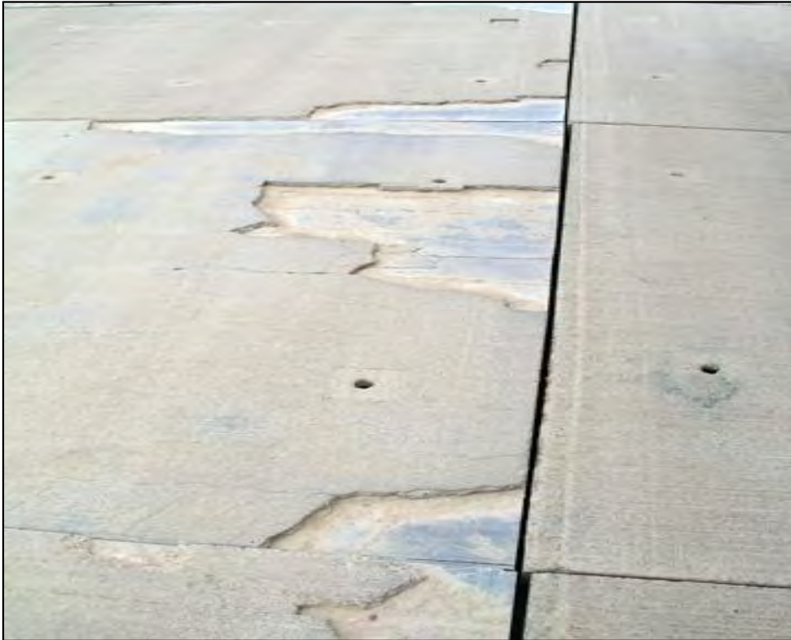
Figure C.4 Prodeck 4, surface delaminating.
