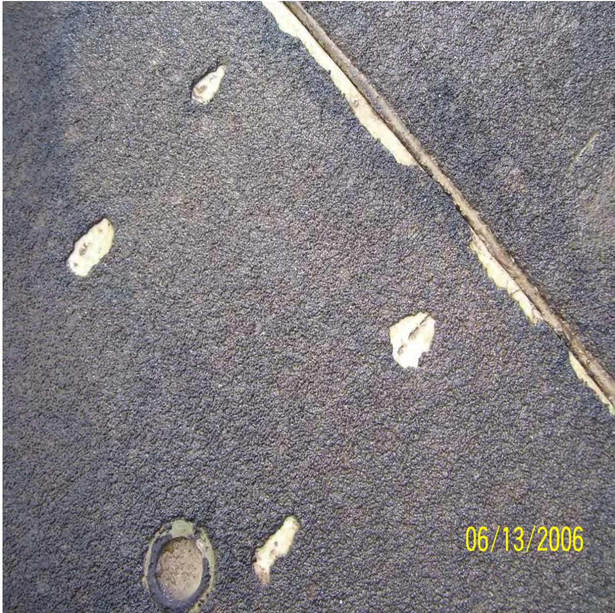
Figure B.10 Early delamination of the Transonite wearing surface (1 year old).
