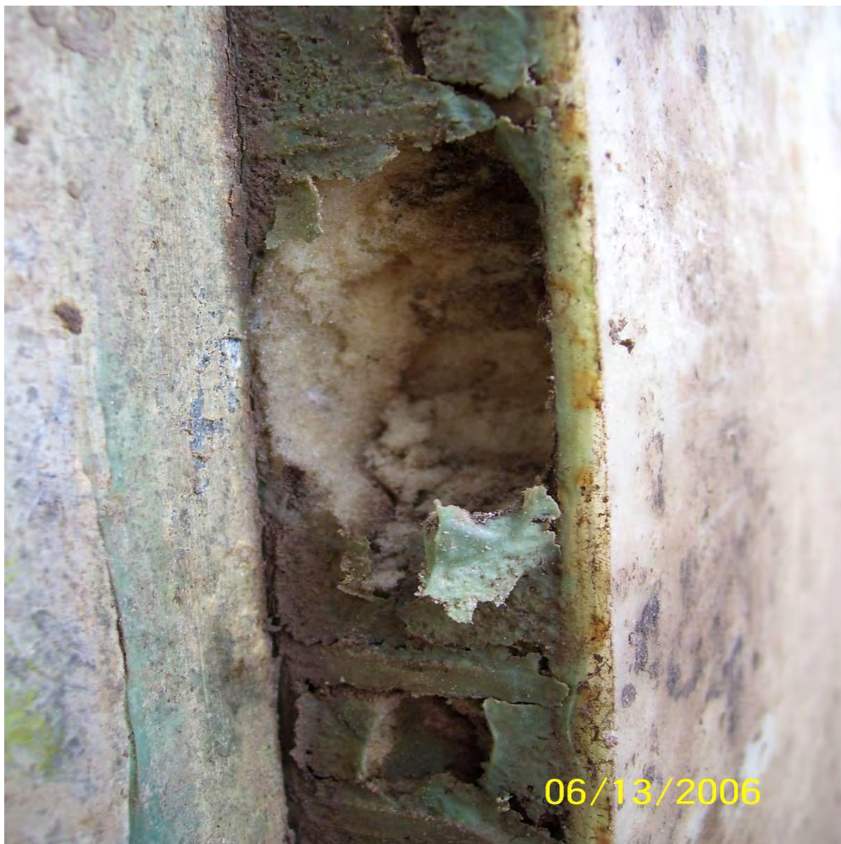
Figure B.16 Damaged fiberglass pillars and foam in the Transonite panel.
