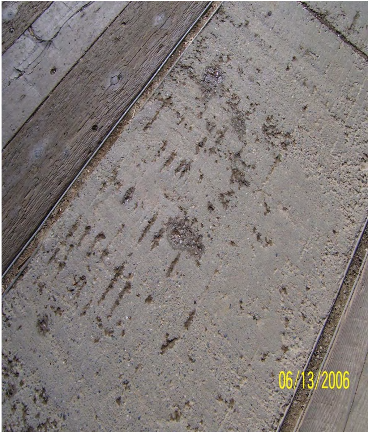
Figure B.8 Concrete-filled metal grid: Possible chain damage (age is 7 years).
