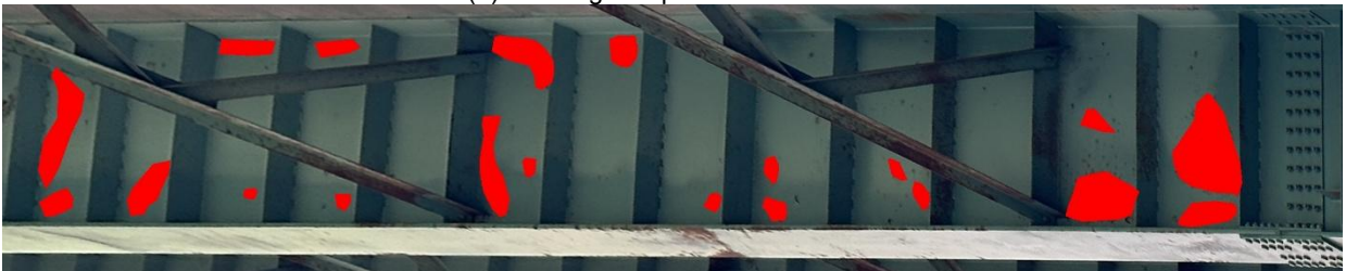
(e) Damaged Map Overlaid on Steel Girder (Damaged Regions Shown in Red)
