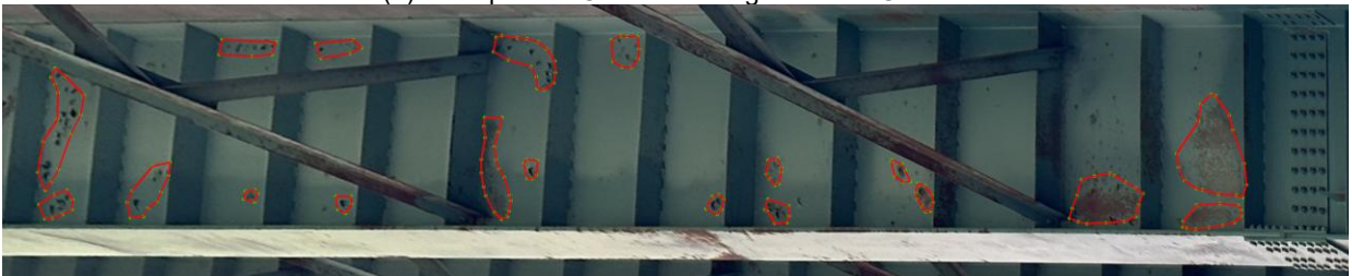
(c) Annotation of Damaged Regions
