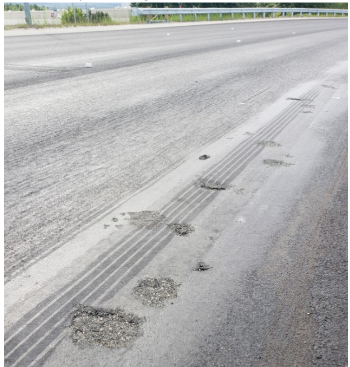
Photo 7 - Ramp 2 Flushing Distress
