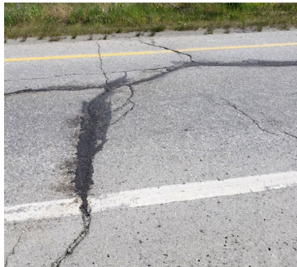
Photo 6 - Ramp 12 - Cracks after Surface Preparation
