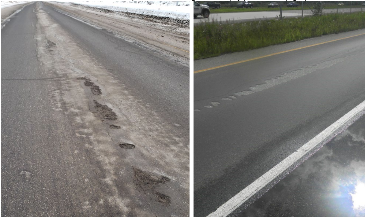
Photo 10 - Ramp 12 Plow Damage – 2021 (left) and 2022 (right)
