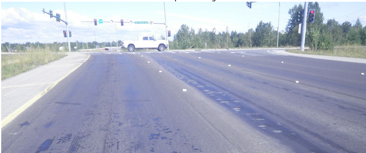
Photo 82 - Ramp 2 Flushing Distress
