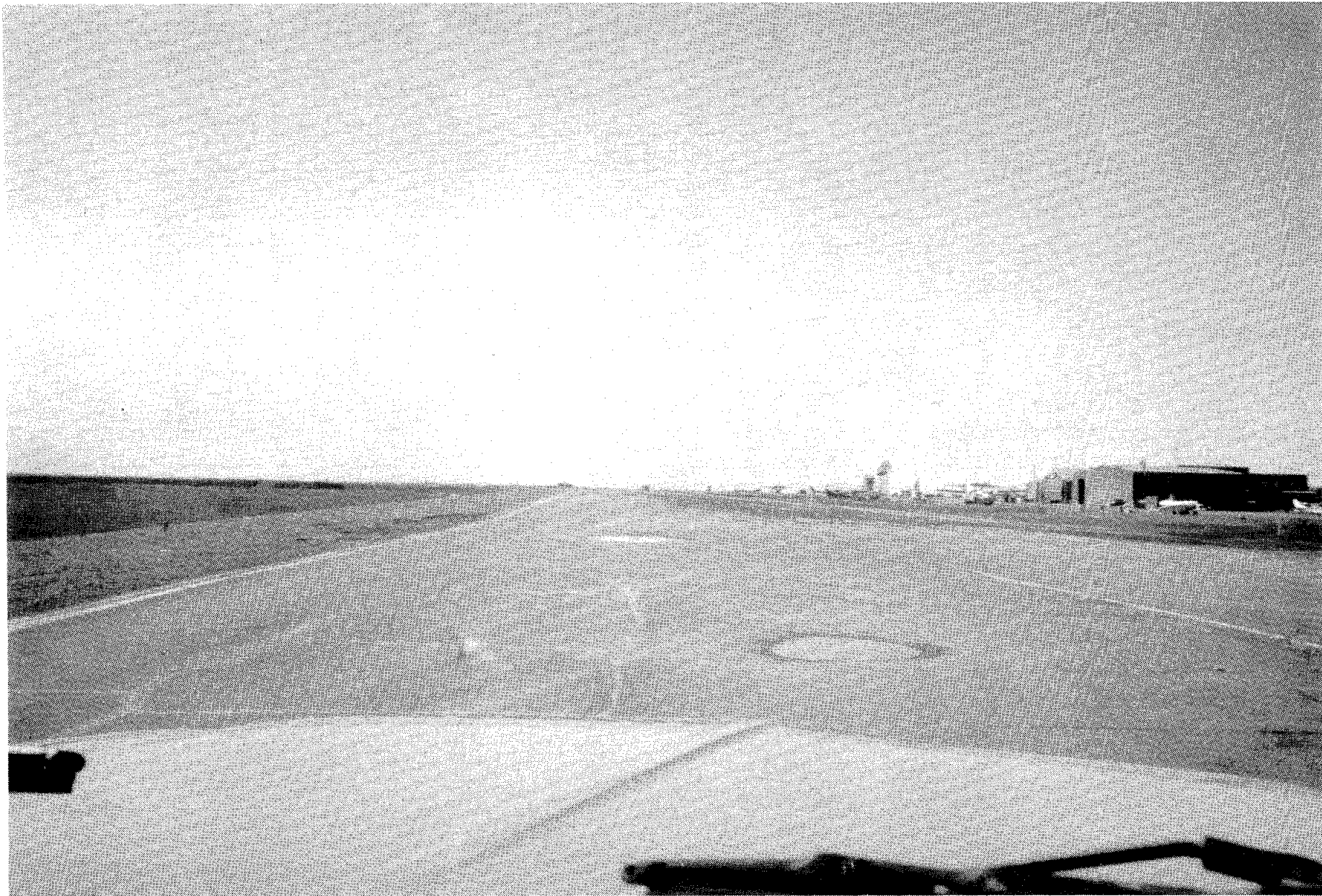
Figure 17: Pooled water on a ramp of the Deadhorse Airport which shows the areas subjected to settling due to the thawing of the underlying ice-rich permafrost.
