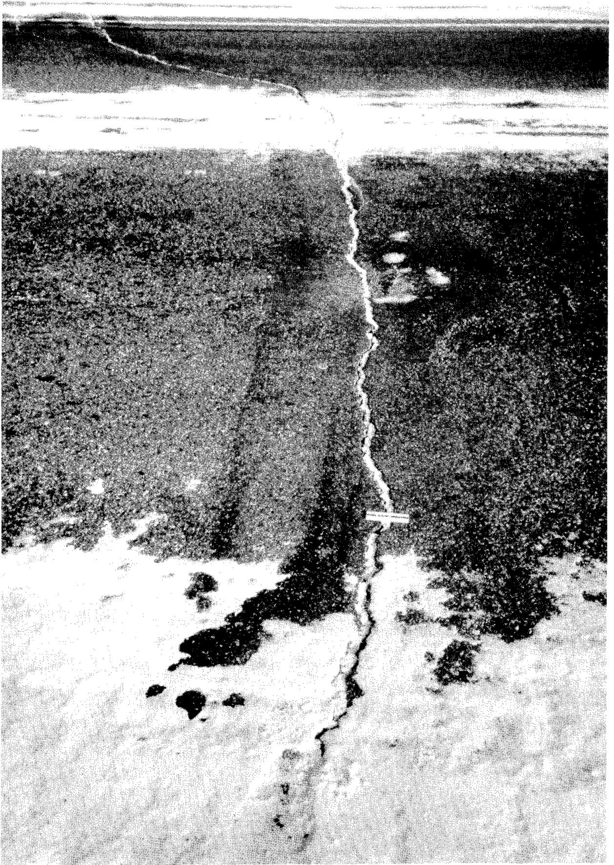
Figure 1: Transverse pavement crack on the Parks Highway (crack number 12, Table 1) during winter. The scale left of center is \approx 17 cm in length.
