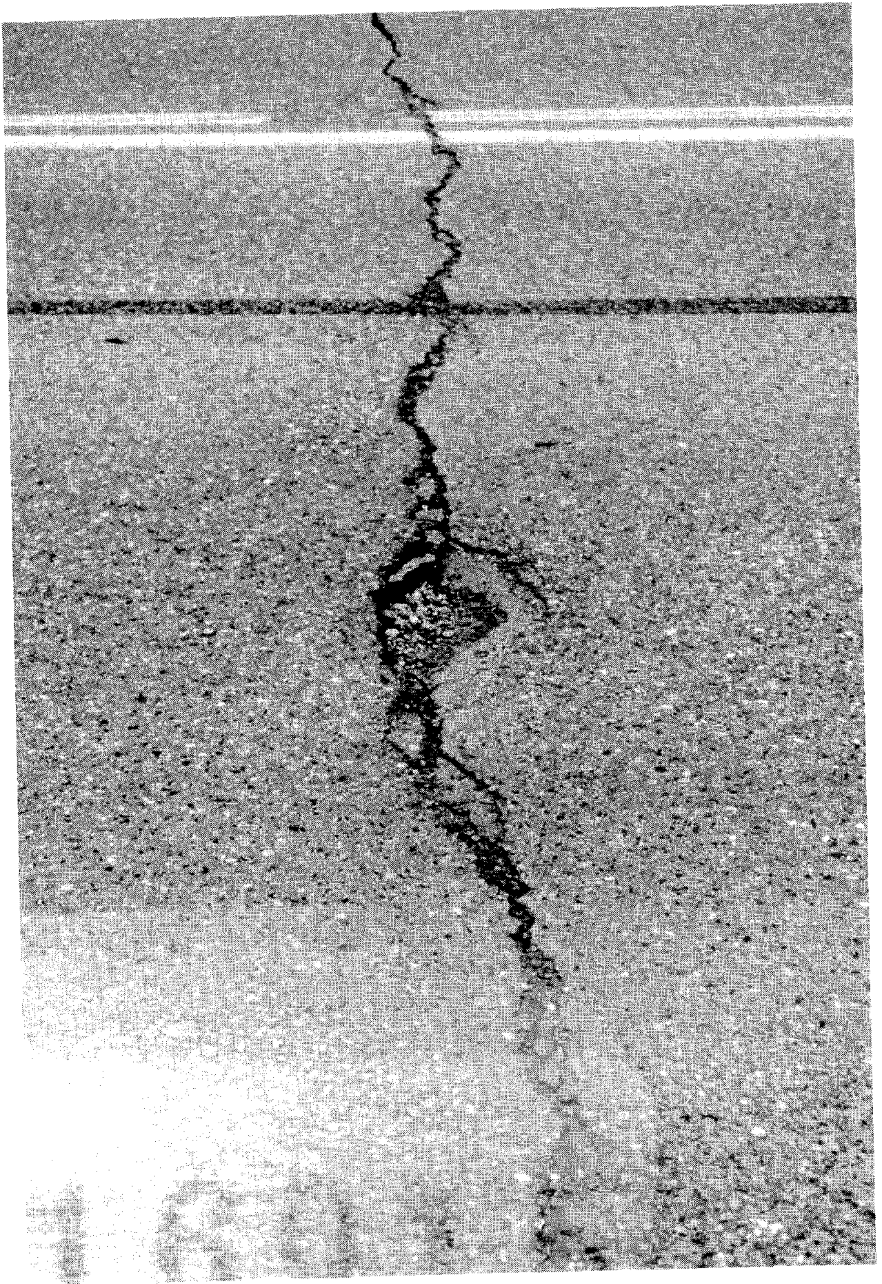
Figure 6: Pothole beginning to form in a crack.
