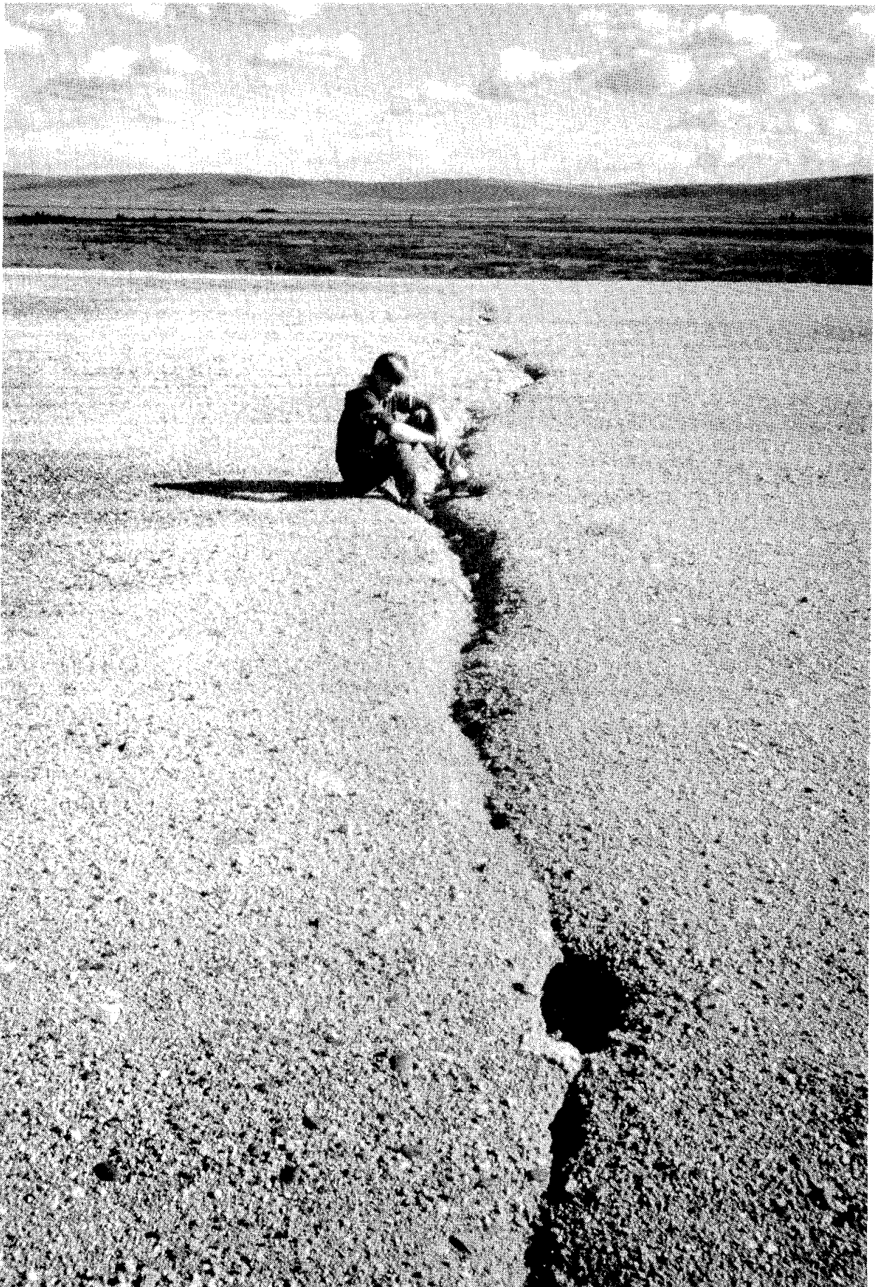
Figure 16: A major transverse crack in the gravel runway of Old Man Airport.
