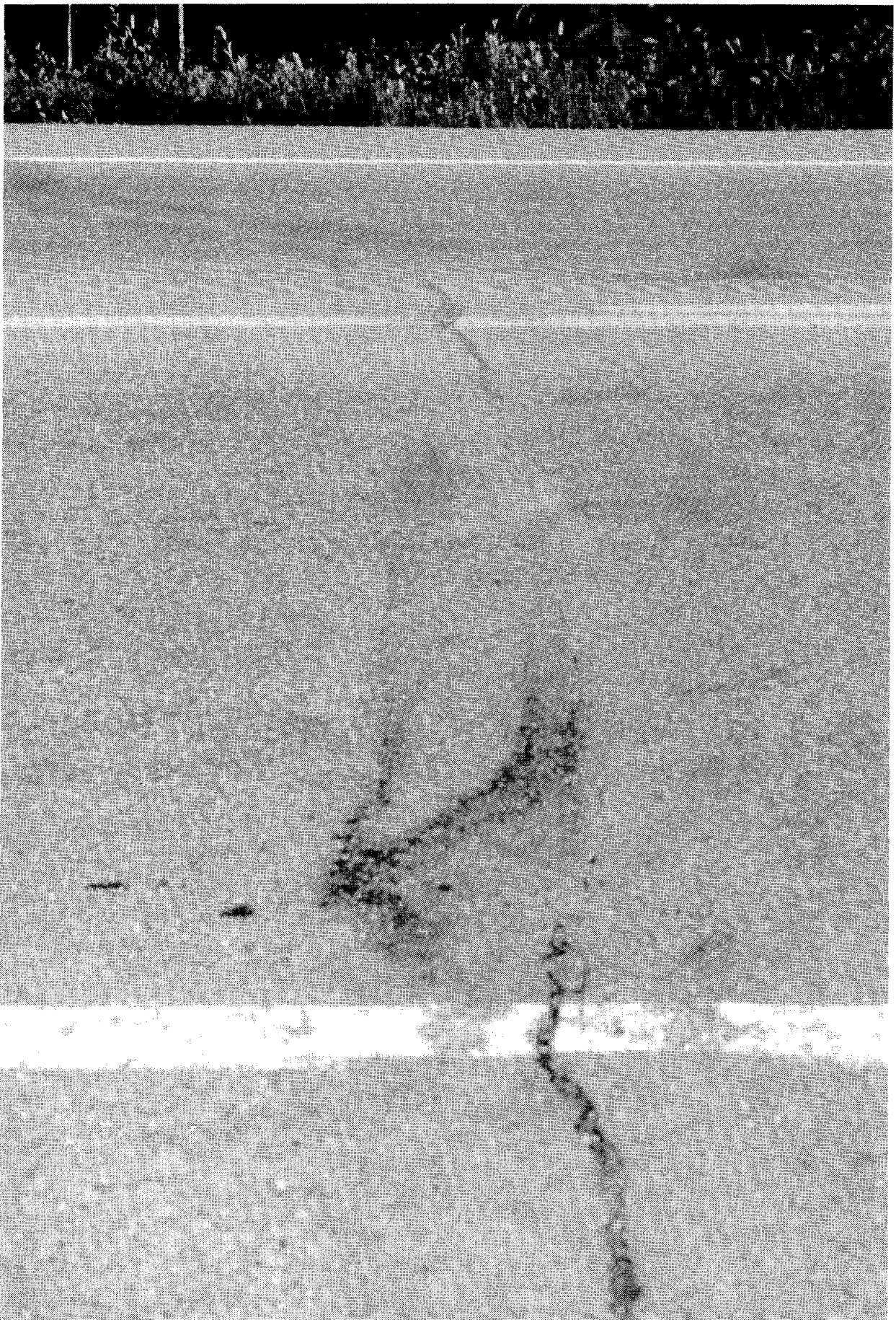
Figure 2: Transverse pavement crack on the Parks Highway during summer.
