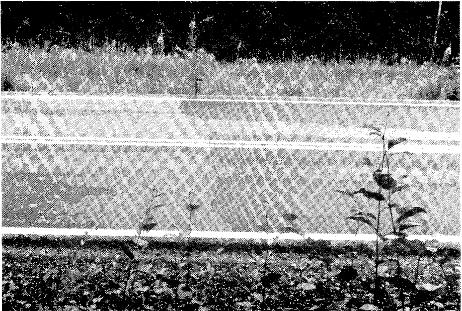
Figure 3: Transverse pavement crack after a shower showing the wet pavement on the uphill (right side) of the crack and the dry pavement on the downhill side.
