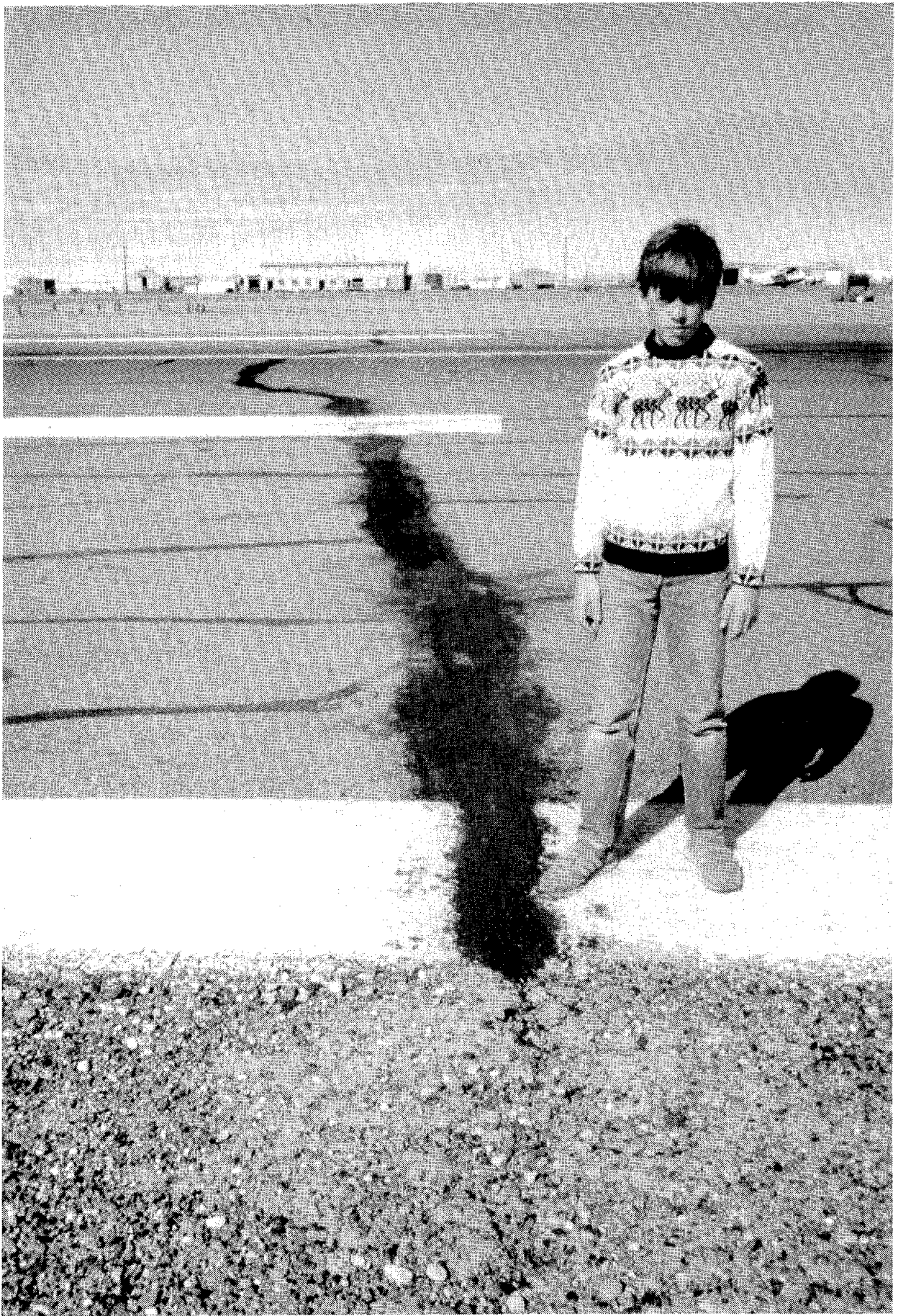
Figure 20: Major transverse crack in the pavement on the northeast end of the Deadhorse Airport Runway which has been patched recently. The cracks in this end of the runway were much more prominent than in the southwest end (Figures 18 and 19).
