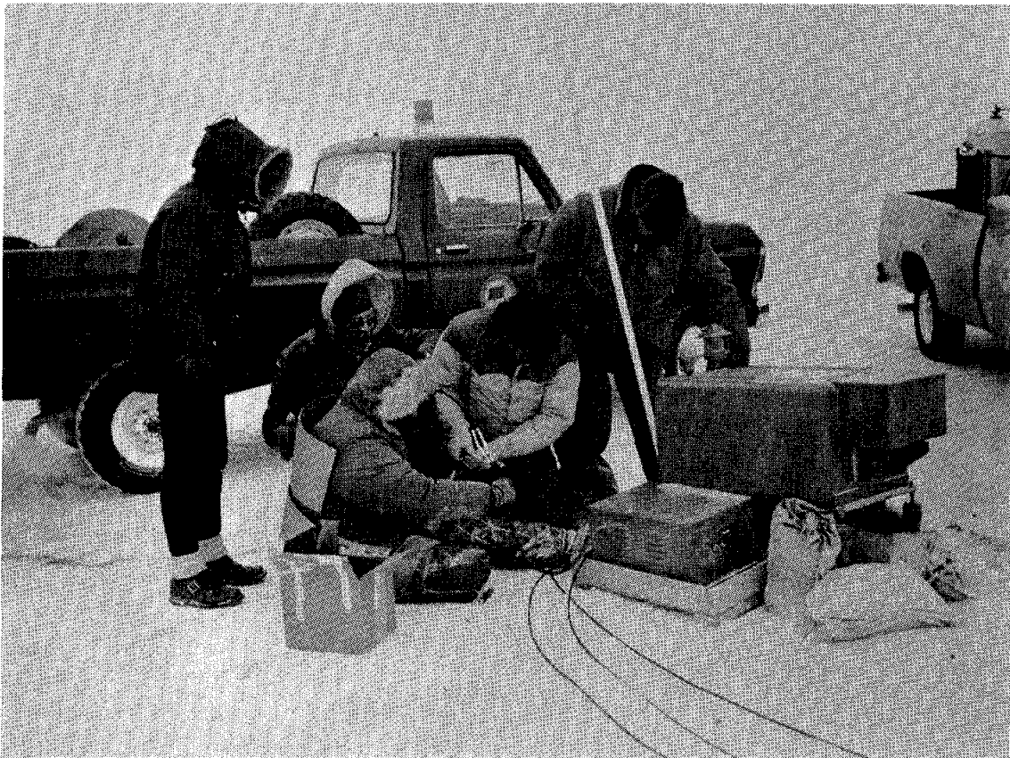
Photo No. 6: Left to right: Frank McHugh, John Scott, Chuck Landers, Mike Gavin, and Jed Atkins splice the power supply cables for the Bethel installation in windy -20°F weather. Vehicles were parked to deflect wind, and pieces of cardboard at Landers' back were also used to minimize discomfort.
