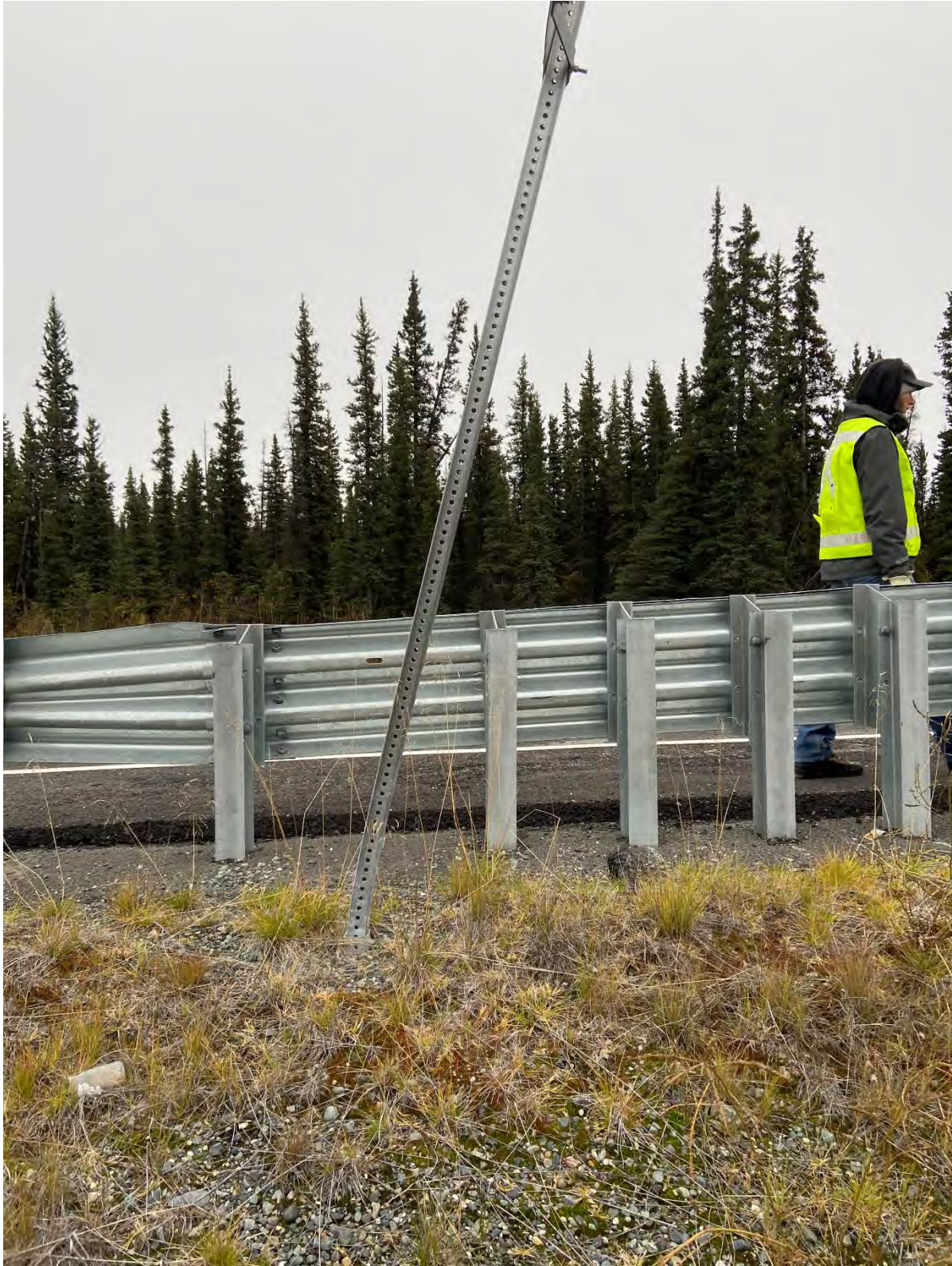
Tok Cutoff MP 17.5 site. Telespar sign post bent likely from snowplow-thrown snow.
