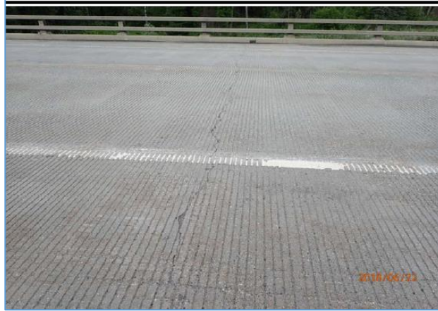
Figure 2.3 Cracks on silica fume deck at Troublesome Creek Bridge (Alaska DOT&PF Bridge Section, 2018)
