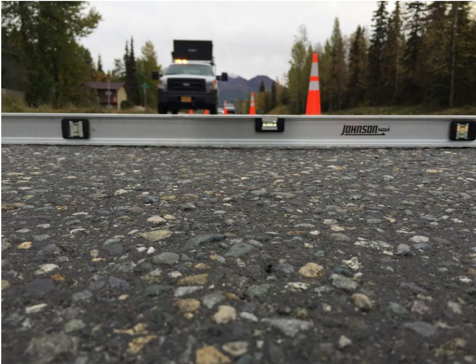
Figure 16: HMA rut on Abbott Road (Abaza, 2018).
