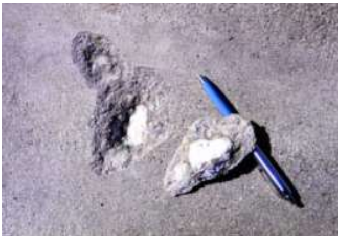
Figure E6: Example of a pop-out on concrete surface (PCA 0113).
