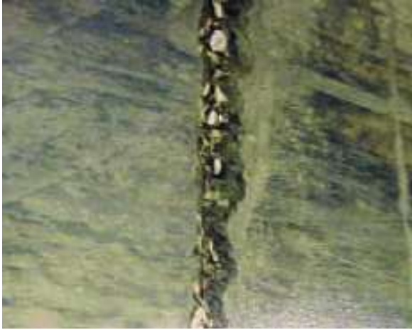
Figure E3: Typical overload crack (PCA 70151).
