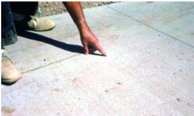
Figure E8: Typical crazing cracks on a concrete surface.
