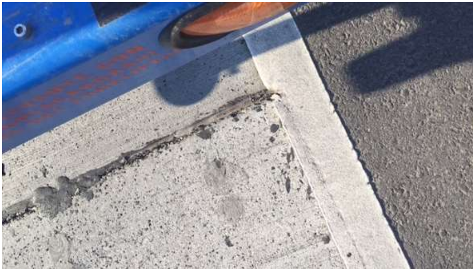
Figure 8: Typical view of crack filling, edge striping, and the slab shoulder joint (Abaza, 2018).
