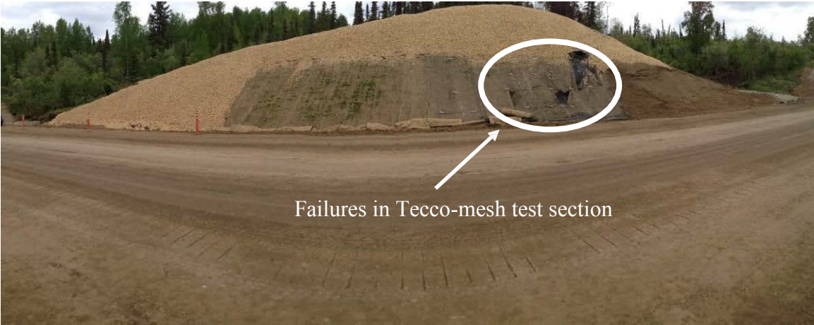
Figure 6.1 Panorama view of Experimental Feature showing failure in Tecco-mesh section
