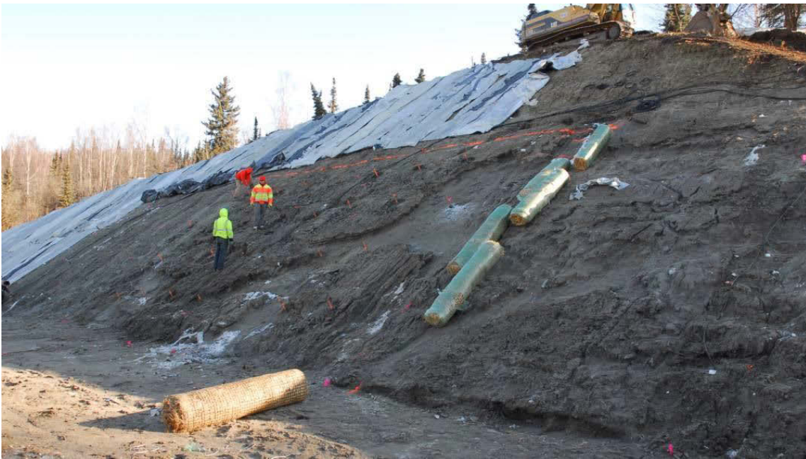
Figure 4.7 Cut slope erosion during construction
