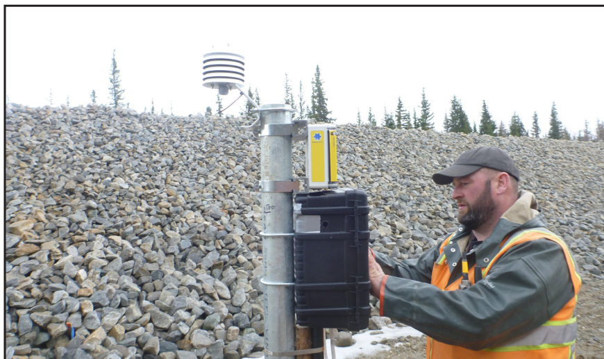
Matt Billings, Alaska DOT&PF Geotechnical Engineer, installs data logger hardware in weather proof case as part of the Alaska Highway ACE experimental feature.
