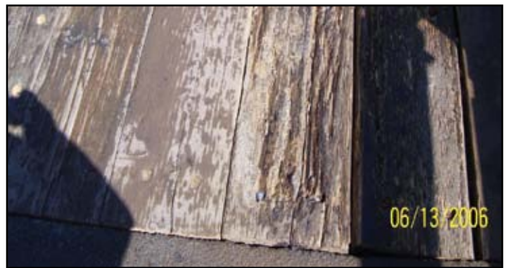
Decay in the top of the wearing surface.
