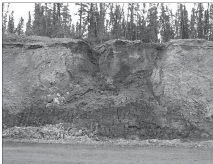
Dalton Highway unstable slope
