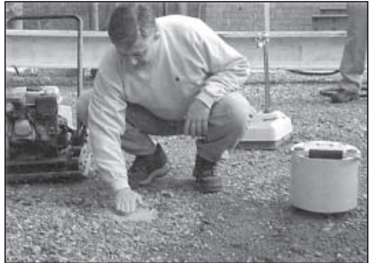
Melvin Main, who helped develop the device on the right known as the SSG, prepares the ground with a thin layer of sand to perform a soil stiffness test.
