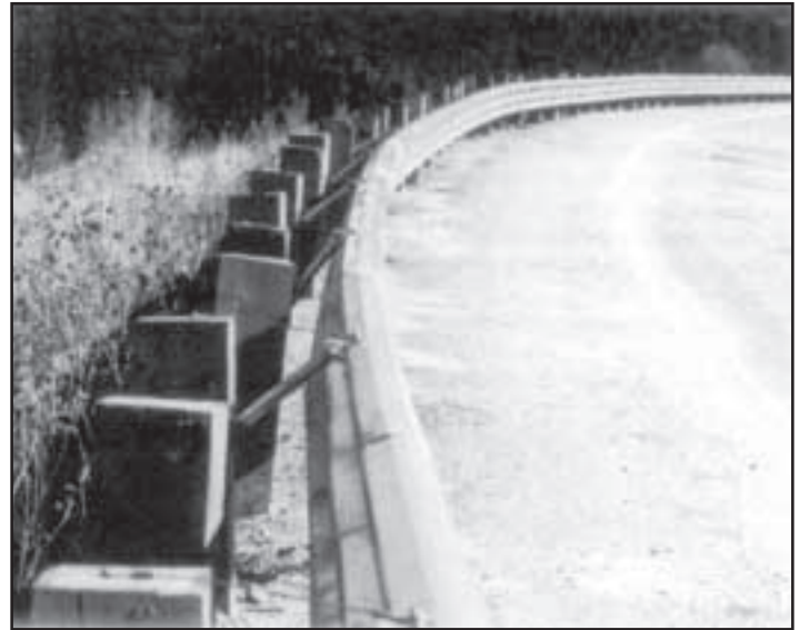
Installing, repairing, upgrading, and replacing roadside hardware such as this guardrail requires hundreds of millions of dollars annually.
