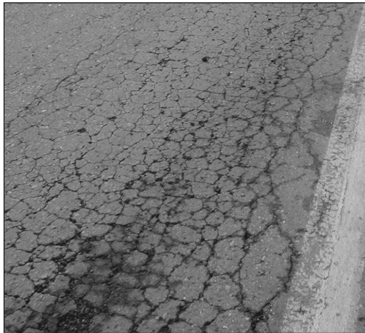
Figure 4-5. Advanced Fatigue Cracking of Highway Pavement
