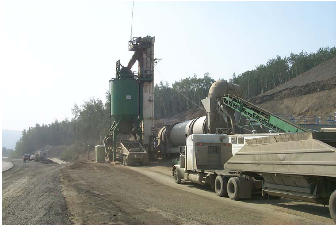
Figure 4-2 Asphalt Batch Plant
