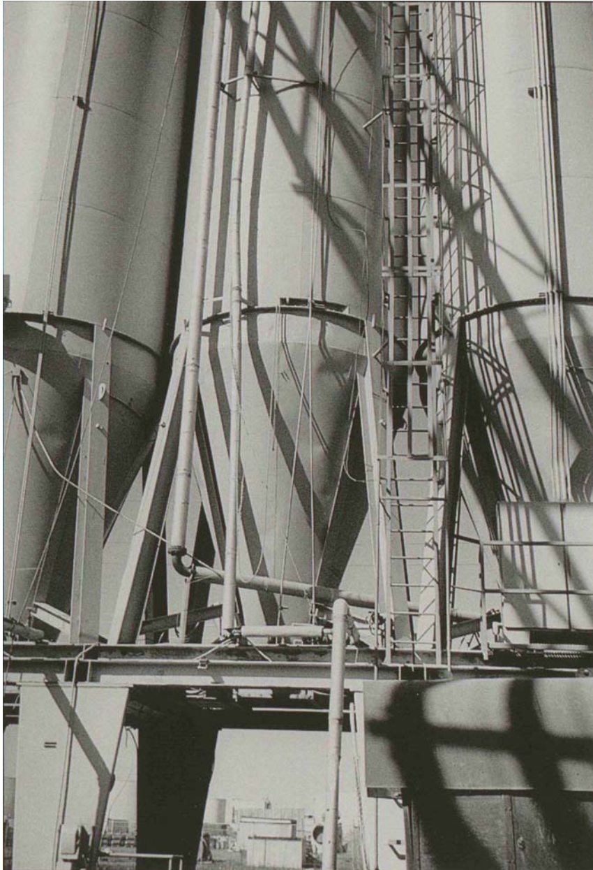
Figure 4-8 Hot Asphalt Storage Silos
