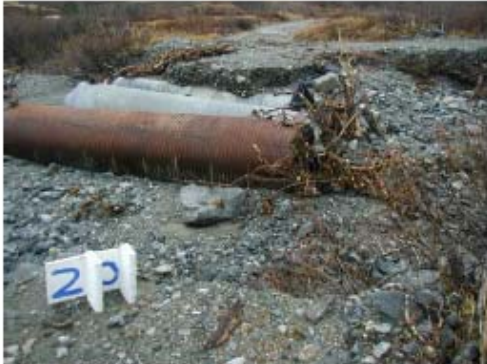
Photo 3: Williamsport Road washed out from 2003 Flooding.
