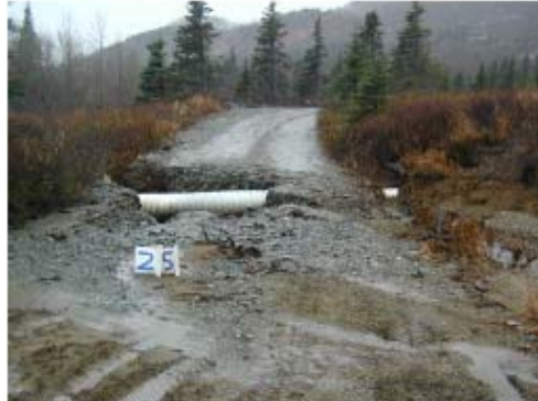
Photo 4: Williamsport Road washed out from 2003 Flooding.
