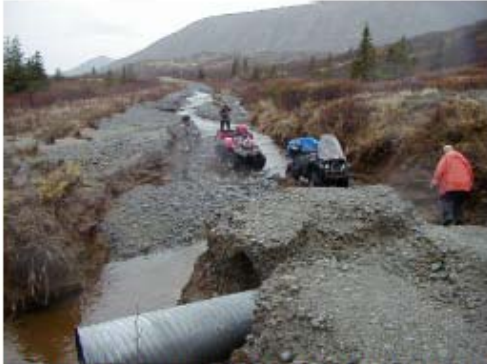
Photo 1: Williamsport Road washed out from 2003 Flooding.
