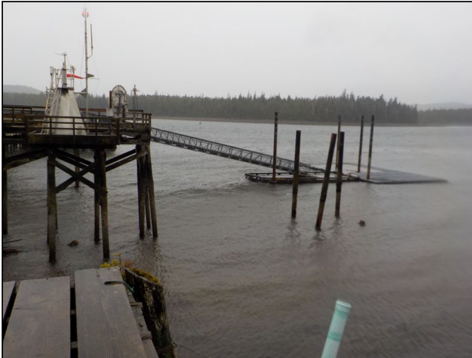
Hydaburg seaplane facility looking north west from the adjacent city dock. One pile collar at the gangway landing float has detached and the associated pile is no longer anchoring the float into position.
