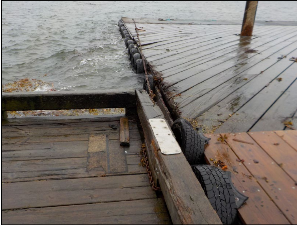
Gangway float and main float held together with chain (in lieu of piling) after storm damage. Several deck boards on the main float are no longer attached to the underlying stringers and pop up when there is wave action at the float.
