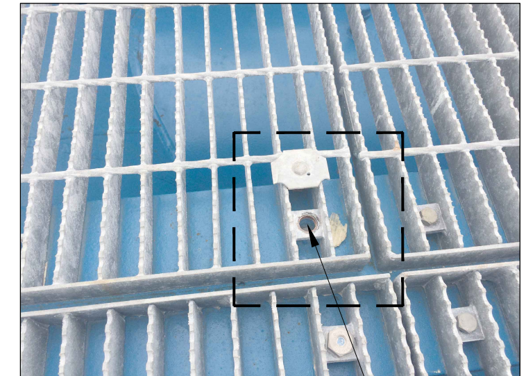
PROVIDE NEW DECK CLIP (SHOWN ABOVE) TO SECURE GRATING TO THE DECK BEAM FLANGE AT LOCATIONS WHERE THE ANCHOR BOLTS ARE DAMAGED/MISSING.
