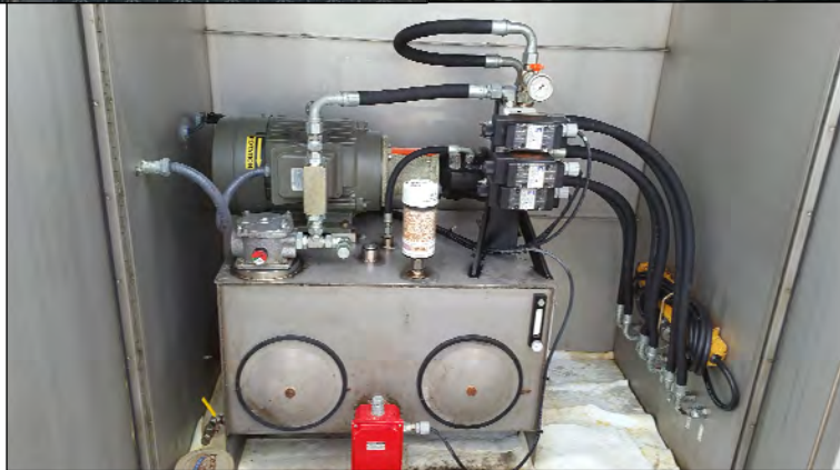
6 HYDRAULIC POWER UNIT & CONTROLS SALVAGE 704 705
