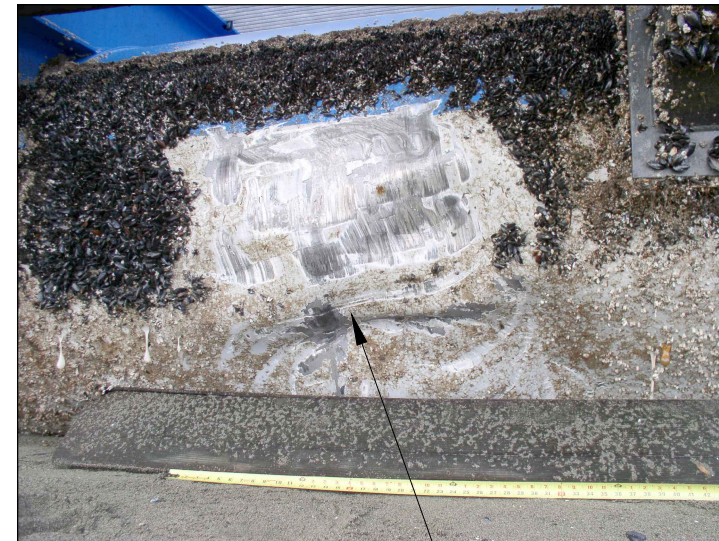
REPAIR DAMAGED ZINC-PAINT BOTTOM COAT ON STEEL FLOAT PONTOONS.
