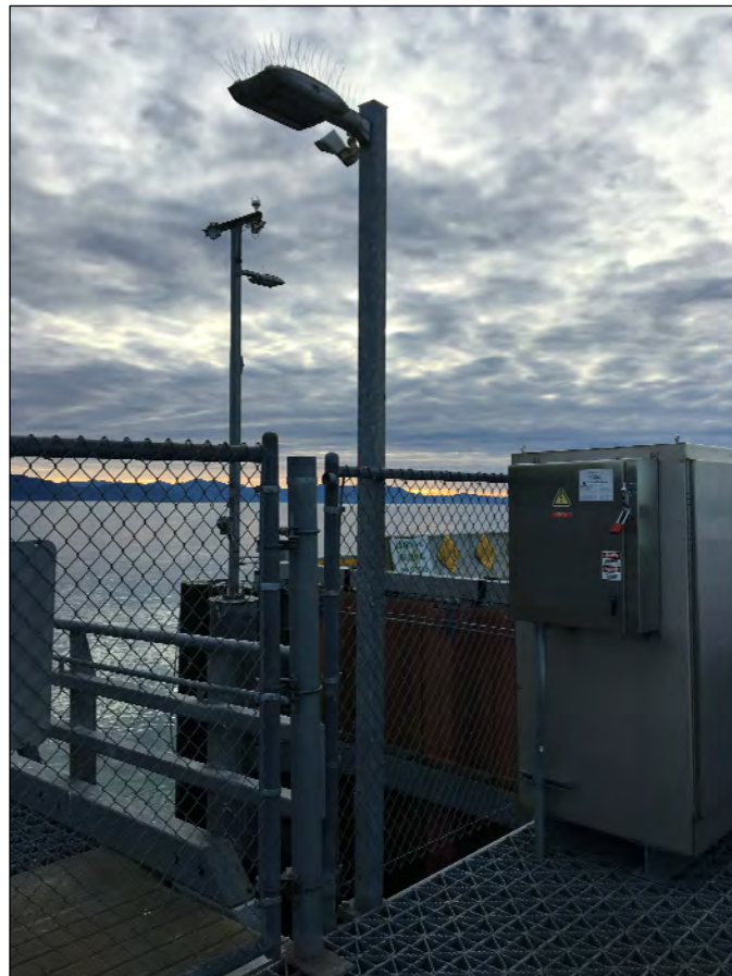
5 LIGHT POLES & CAMERAS SALVAGE 704 705
