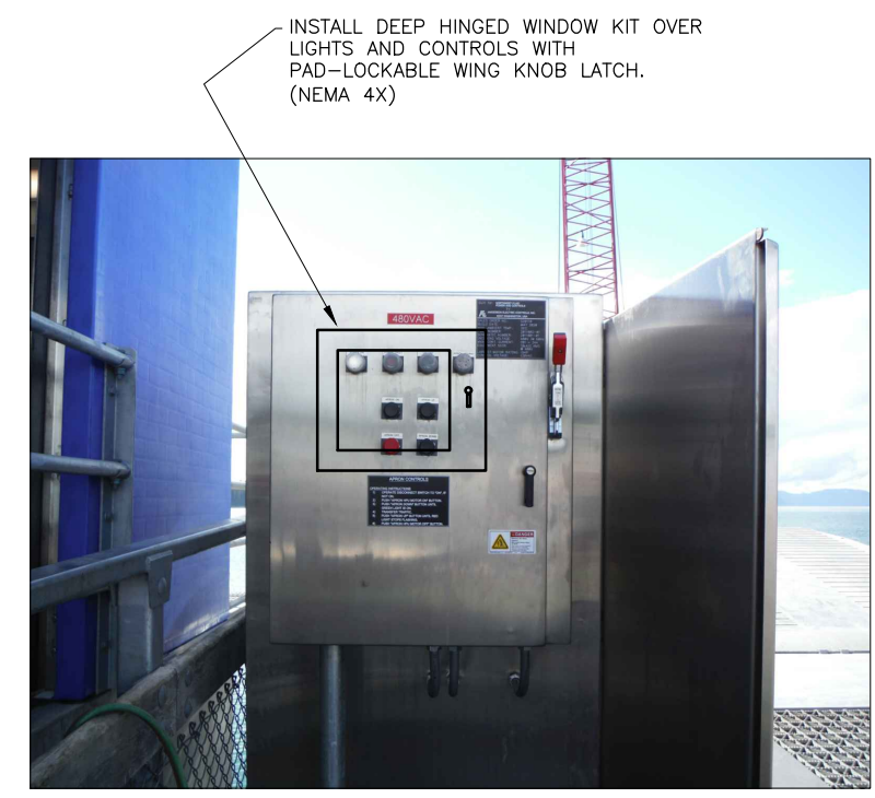
CONTROL PANEL MOD APRON HYDRAULIC ELECTRICAL PANEL
