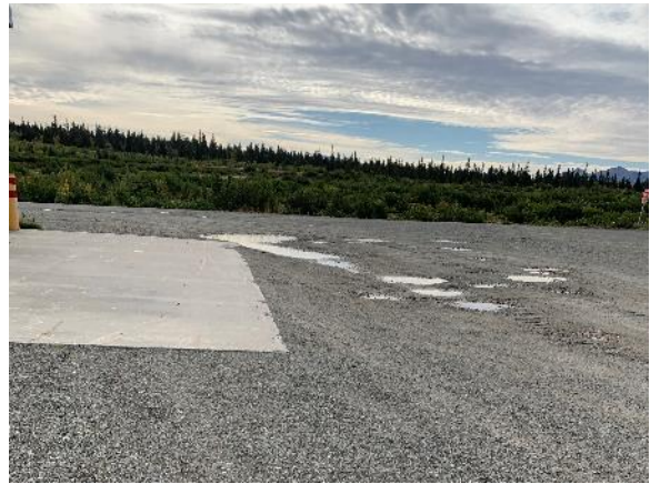
Figure 11: Potholes Near SREB, Looking South
