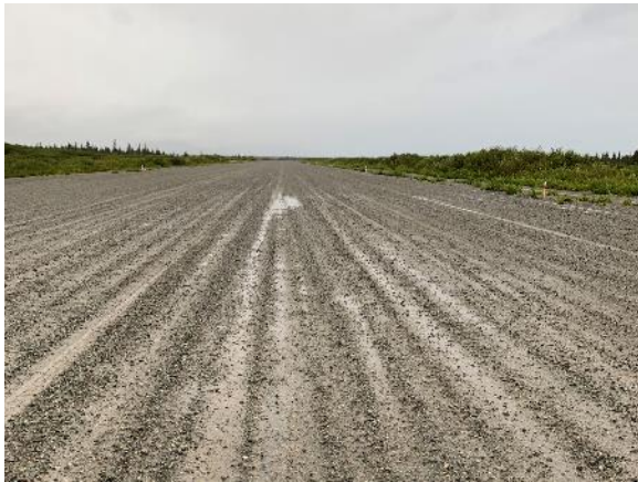
Figure 12: Runway Rutting and Soft Areas When Wet, Looking West
