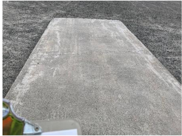
Figure 3: Crack in Apron Hard Stand, Looking South
