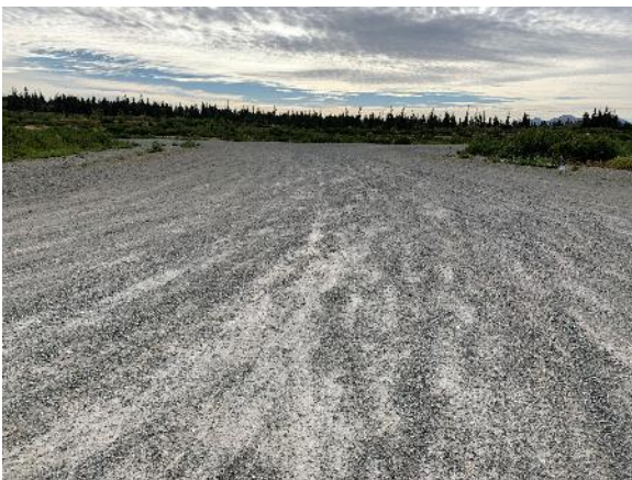
Figure 6: Ruts and Thin Surfacing on Taxiway, Looking South
