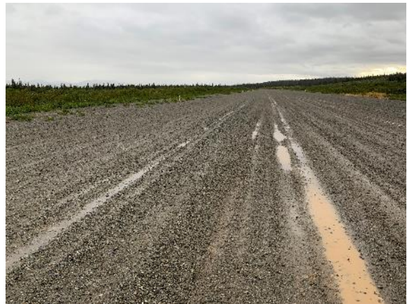
Figure 5: Ruts on Runway, Looking East
