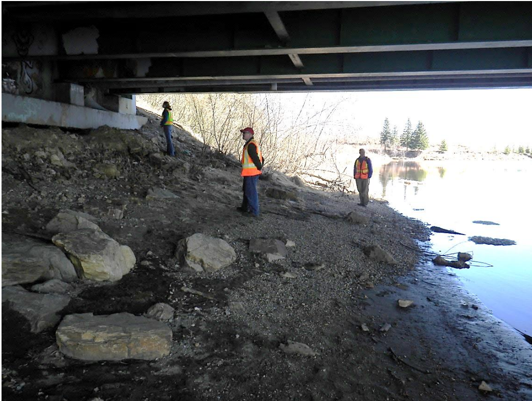
Photo 2 Minor erosion and scattered riprap observed at the north abutment, looking east; May 20, 2013
