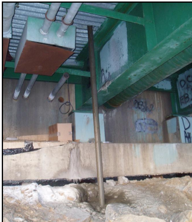
Photo 4. North abutment. Conduits overhead. Erosion under cap.
