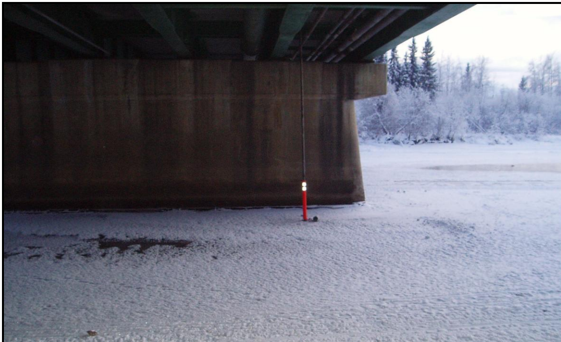
Photo 2. Pier 3 Pen test in progress. Suspended conduits visible. Chena River flow is to the right.
