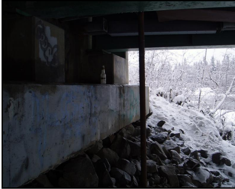
Photo 3. South abutment, looking west. Erosion under cap.
