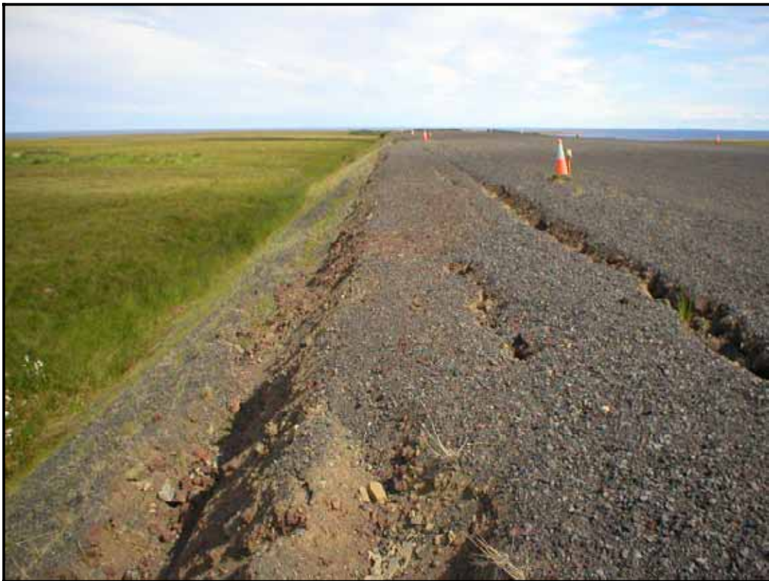
Photograph A-1: Longitudinal Cracks on Runway Embankment caused by Permafrost Degradation
