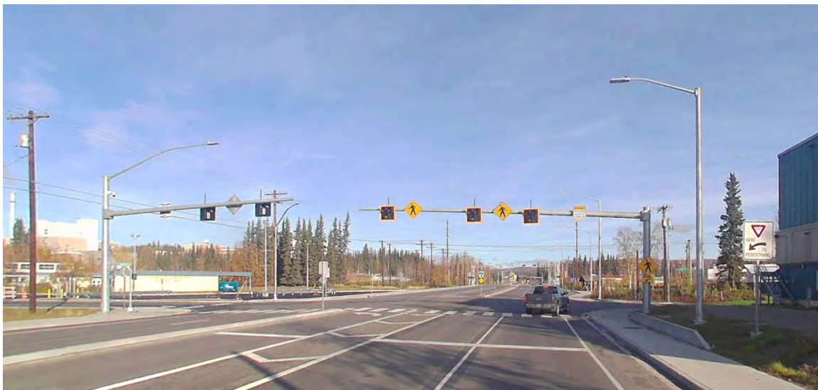
Figure 40. Pedestrian Hybrid Beacon example (on University Avenue at Sandvik Street)
