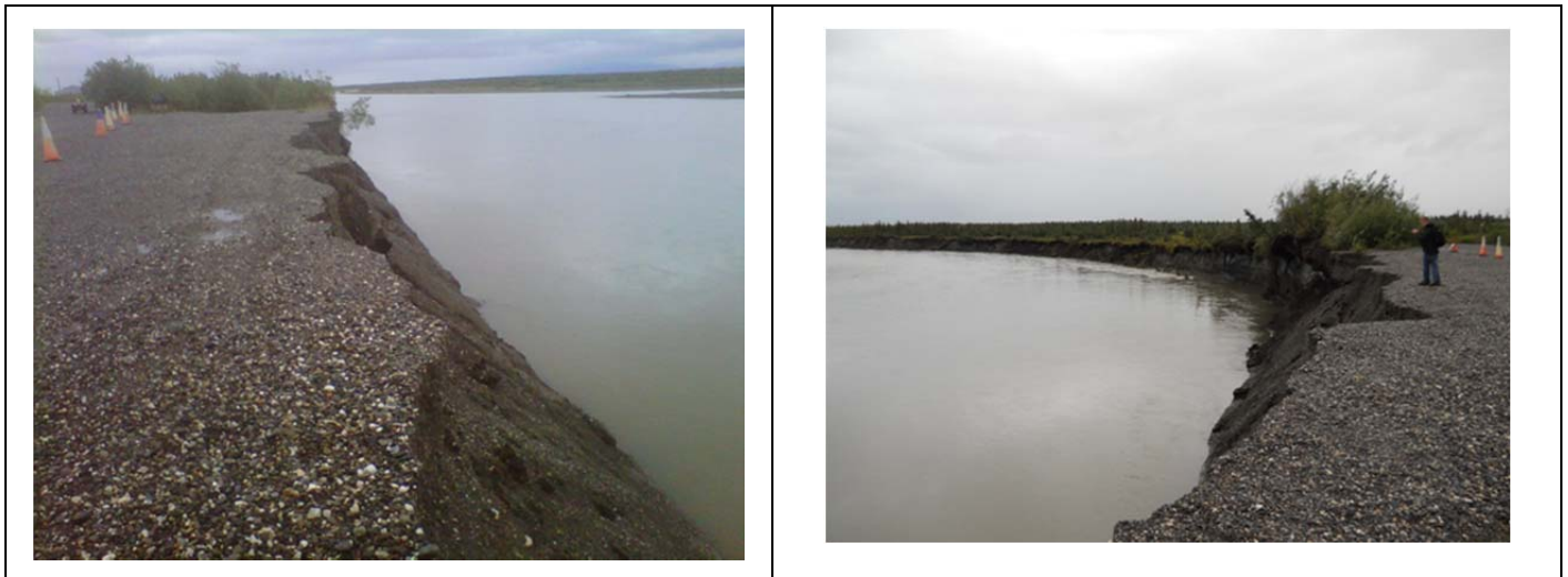
Figure 5: Bank Erosion August 2012 Orange cones set along east side of Pit Road. (Left) looking upriver from Point C (Right) looking downriver from Point B
