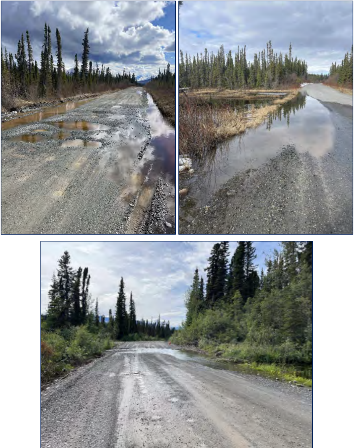
Figure 1-7. Examples of Drainage Issues and Lack of Ditches
