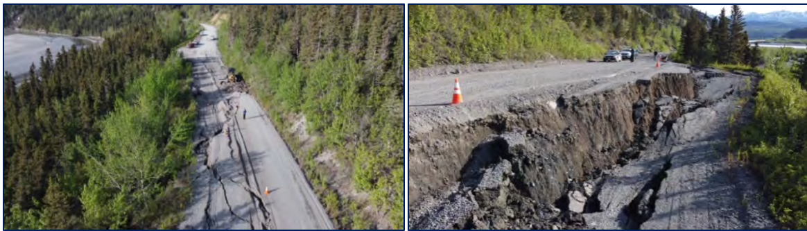
Figure 4-3. Road Settlement Issues near MP 0.5
