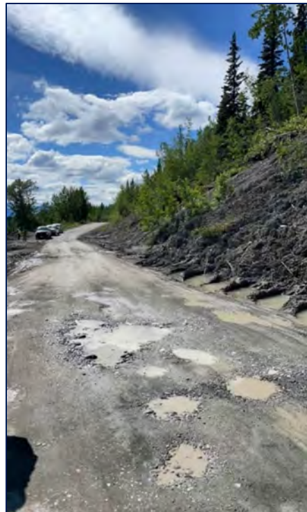
Figure 4-12. McCarthy Road Conditions near MP 58
