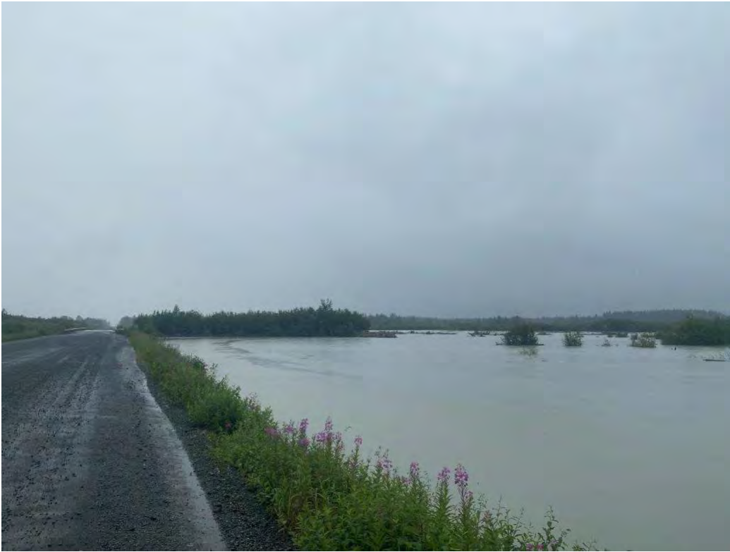
Image 4: Approach to the east side of the bridge, water being impounded on the north side with no drainage points.
