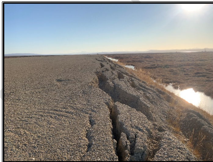
Figure 1: RW 11-29 RSA degradation present during October 14, 2020 Site Visit (View southeast)
