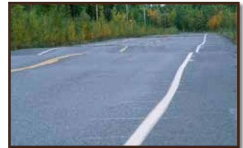
Frost heaves on the Richardson Highway.
