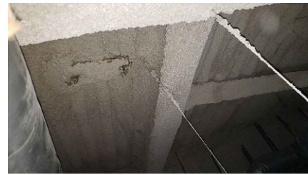
LOCATION 12: RUSTING AROUND BRACKETS. ACM FIREPROOFING NOT STAINED.
