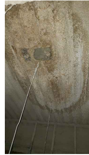
LOCATION 7: WATER STAINED/DAMAGED SPRAY-ON ACM FIREPROOFING.
