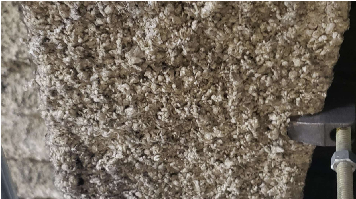
Photo 20: Tannish-gray spray on fireproofing located on the sixth floor in part of the mechanical areas. This fireproofing was non-detect for asbestos.
