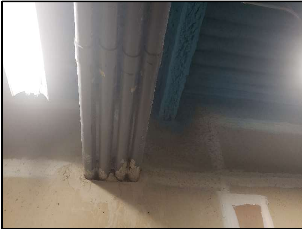
Photo 18: Typical Mechanical space present on Floors 5-7 depicting blue colored fireproofing on pan decking (non-asbestos containing) with gray fireproofing overspray on walls and piping (Chrysotile asbestos containing).
