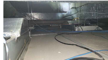
LOCATION 9: OVERSPRAY OF ACM FIREPROOFING ON TOP OF CEILING TILES. ACM FIREPROOFING ON PANDECKING IN GOOD CONDITION.
