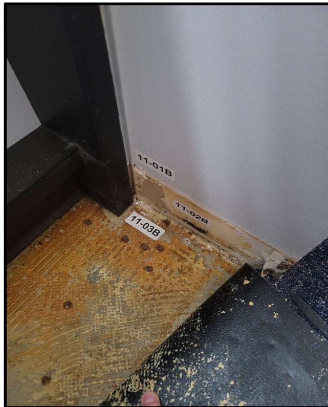
Photo 14: Joint compound (6% Chrysotile) and cove base mastic (1.25% Anthophyllite) contain asbestos. Old carpet mastic and existing carpet adhesive do not contain asbestos.
