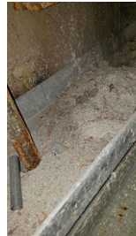
LOCATION 22: OVERSPRAY OF ACM FIREPROOFING IN CHANNEL IRON. ACM FIREPROOFING ON PANDECKING IN GOOD CONDITION.
