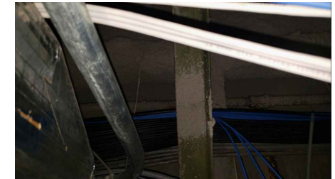
LOCATION 24: OVERSPRAY OF ACM FIREPROOFING IN CHANNEL IRON AND ON TOP OF CEILING TILES. CABLE BUNDLES STRUNG OVER SUPPORTS HAVE ACM FIREPROOFING ON THEM, DAMAGING THE ACM.
