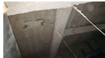
LOCATION 12: RUSTING AROUND BRACKETS. ACM FIREPROOFING NOT STAINED.
