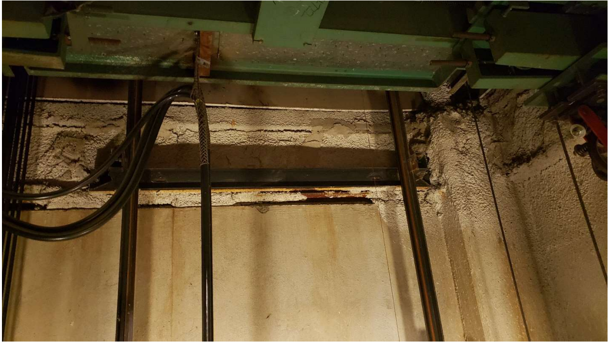
Photo 21: Damaged ACM containing fireproofing within an elevator shaft. Note the cracks and missing pieces.
