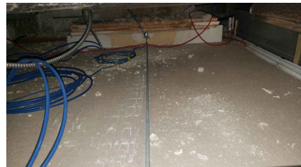
LOCATION 23: OVERSPRAY OF ACM FIREPROOFING IN CHANNEL IRON AND ON TOP OF CEILING TILES. ASSOCIATED ACM FIREPROOFING ON PANDECKING IN GOOD CONDITION.
