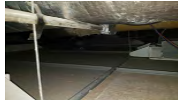
LOCATION 10: OVERSPRAY OF ACM FIREPROOFING ON TOP OF CEILING TILES. ACM FIREPROOFING ON PANDECKING IN GOOD CONDITION.
