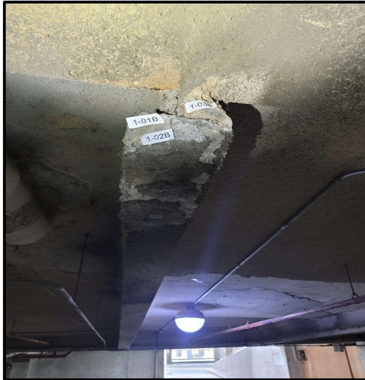
Photo 1: 1 st floor garage showing 3 different materials of fireproofing overlapped, non-homogenous, and damaged.
