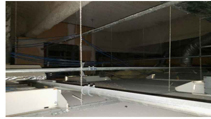
LOCATION 6: OVERSPRAY OF ACM FIREPROOFING ON TOP OF CEILING TILES. ACM FIREPROOFING ON PANDECKING IN GOOD CONDITION.
