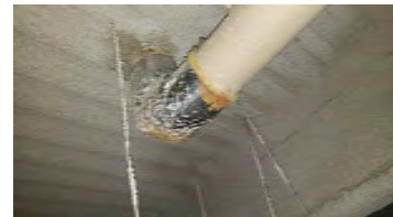
LOCATION 14: WATER STAINING NEAR PIPE PENETRATIONS IN PANDECKING.
