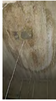
LOCATION 7: WATER STAINED/DAMAGED SPRAY-ON ACM FIREPROOFING.
