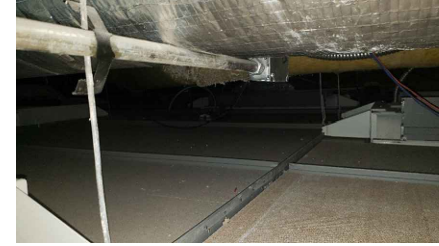
LOCATION 10: OVERSPRAY OF ACM FIREPROOFING ON TOP OF CEILING TILES. ACM FIREPROOFING ON PANDECKING IN GOOD CONDITION.
