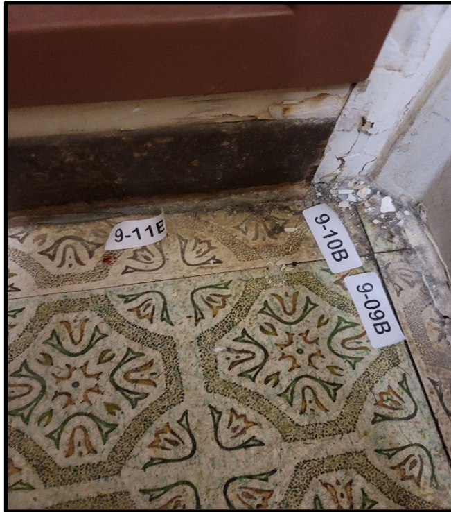
Photo 9: Brown mastic on cove base inside Storage room in front of Mechanical room contains 2.75% Anthophyllite asbestos. Cove base mastic containing asbestos not differentiable from non-asbestos containing cove base mastic throughout Floor 9-11.
