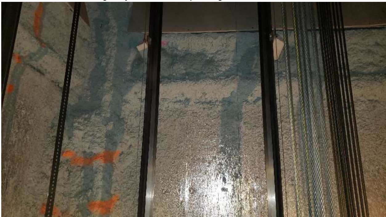
Photo 18: Blue, non-asbestos fireproofing within Elevator 3 shaft. Note the color is less intense than in other areas, again likely due to inconstant amounts of dye mixed with the fireproofing.
