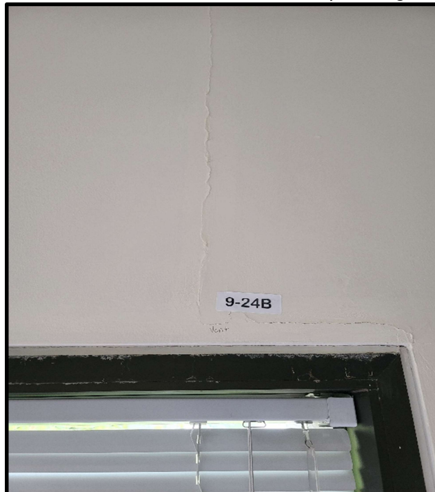
Photo 12: 9 th floor exterior wall above window joint compound contains 5.25% Chrysotile asbestos. Exterior walls, structural columns, and interior spaces surrounding Atrium constructed with asbestos containing joint compound.
