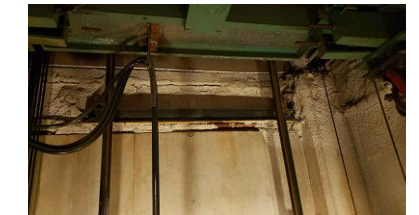
ELEVATOR 4/5: CRACKING AND MISSING PIECES OF ACM FIREPROOFING THROUGHOUT ELEVATOR SHAFT.
