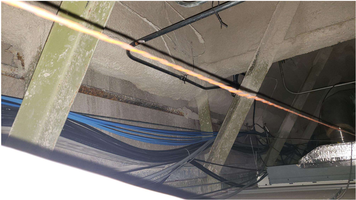
Photo 29: Cable bundles on top of ACM spray on fireproofing.
