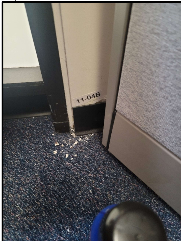
Photo 16: Joint compound sample at corner wall adjoining Atrium window wall contains 6% Chrysotile asbestos.
