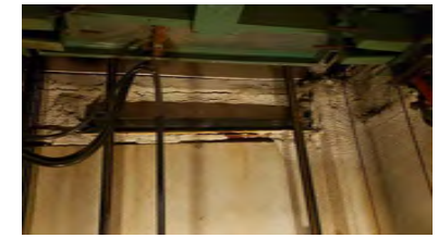
ELEVATOR 4/5: CRACKING AND MISSING PIECES OF ACM FIREPROOFING THROUGHOUT ELEVATOR SHAFT.
