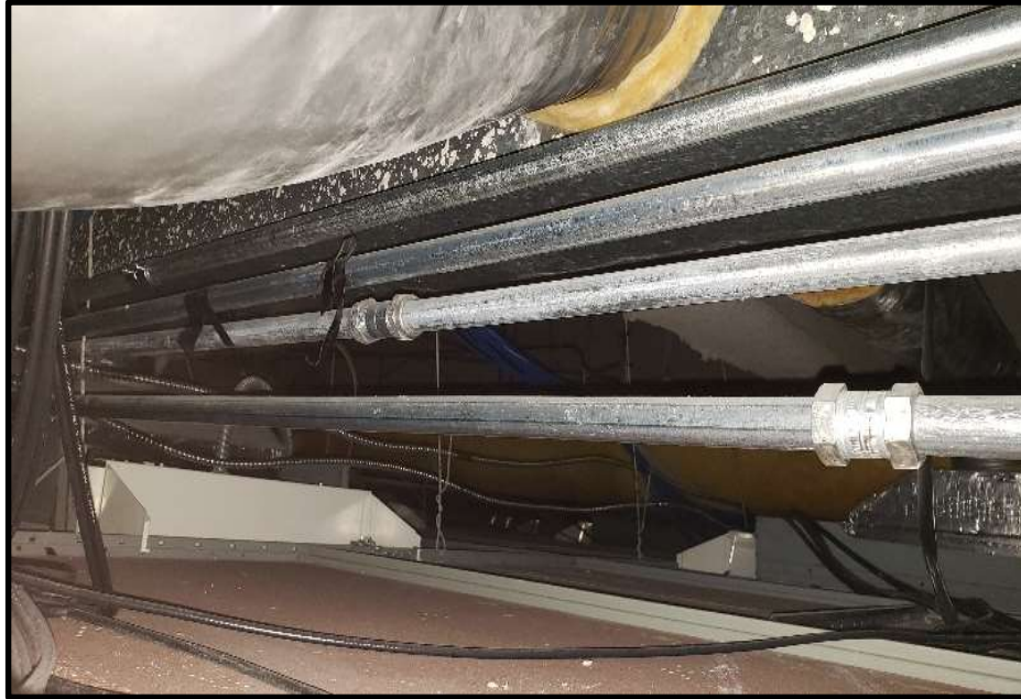
Photo 13: Space between drop ceiling and pan decking on 9 th floor. White spots shown are overspray from spray-on fireproofing. White spots on ceiling tile in bottom of photo are fireproofing that has deteriorated and fallen. Fireproofing contains 10-15% Chrysotile asbestos.
