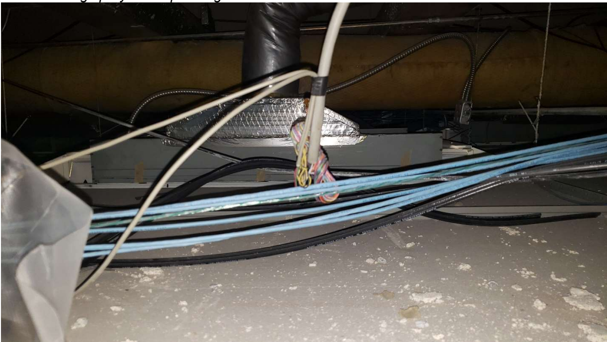
Photo 24: ACM spray on fireproofing on top of ceiling tiles.
