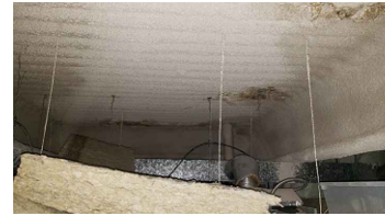
LOCATION 8: WATER STAINED/DAMAGED SPRAY-ON ACM FIREPROOFING.
