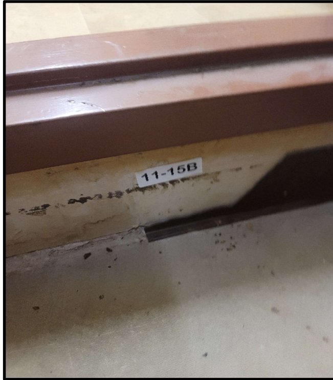
Photo 17: Brown/Yellow mastic containing 2% Anthophyllite asbestos present on brown cove base at step separating Storage room and Mechanical room on 11 th floor.
