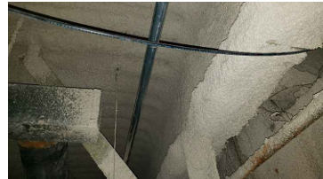
LOCATION 1: ACM FIREPROOFING ON PAN DECKING.
