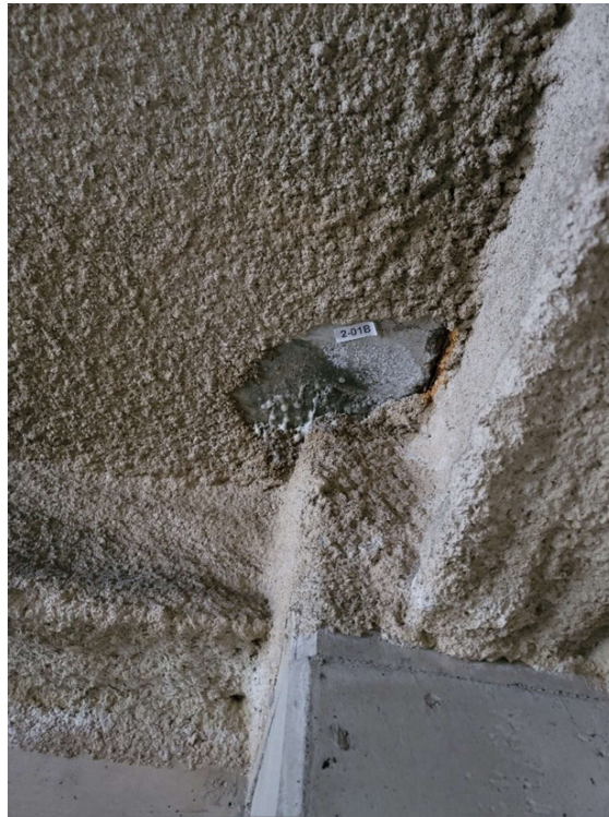
Photo 1: Light tan fireproofing – standard spray pattern
