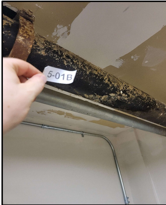
Photo 5: Gray fireproofing overspray on pipe at ceiling inside 5 th floor Maintenance room. Ceiling appears to have been previously abated or hard lid installed encapsulating fireproofing above. Overspray fireproofing contains 25% Chrysotile asbestos.
