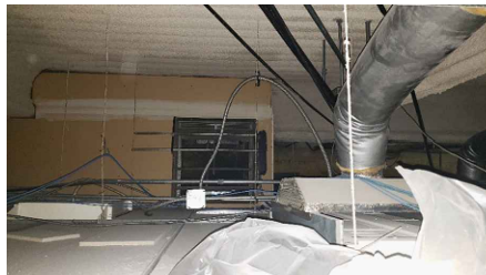
LOCATION 3: OVERSPRAY OF ACM FIREPROOFING ON TOP OF CEILING TILES. ACM FIREPROOFING IN GOOD CONDITION.
