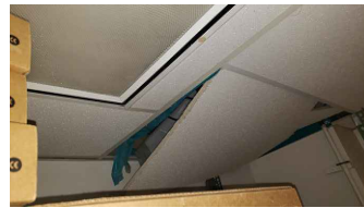
LOCATION 19: PLASTIC COVER OVER/AROUND FIRE SUPPRESSION GLOBE. ACM NOT VISIBLE. ASSUMED WATER DAMAGED.
