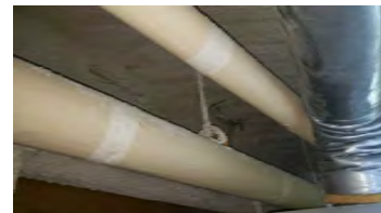
LOCATION 11: CRACKING/STAINING IN DAMAGED ACM FIREPROOFING ON PANDECKING.
