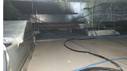
LOCATION 9: OVERSPRAY OF ACM FIREPROOFING ON TOP OF CEILING TILES. ACM FIREPROOFING ON PANDECKING IN GOOD CONDITION.
