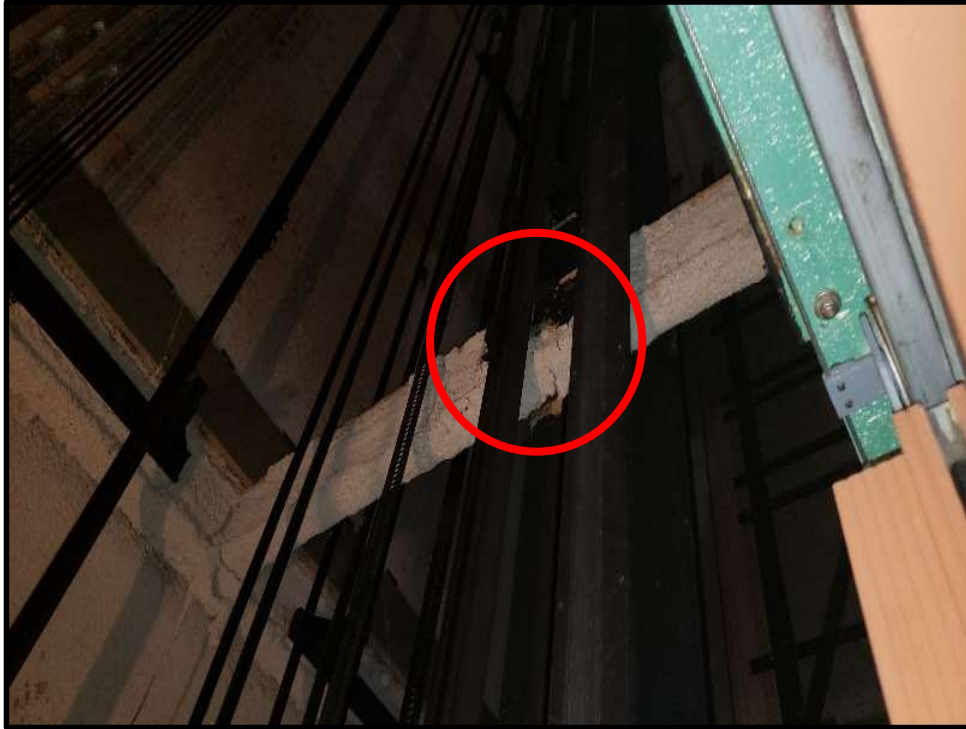
Photo 19: Elevator shaft 6/7, southern 2 elevators in center of building connecting Floors 5-11, showing asbestos containing gray fireproofing. Damage to fireproofing on central beam outlined in red.
