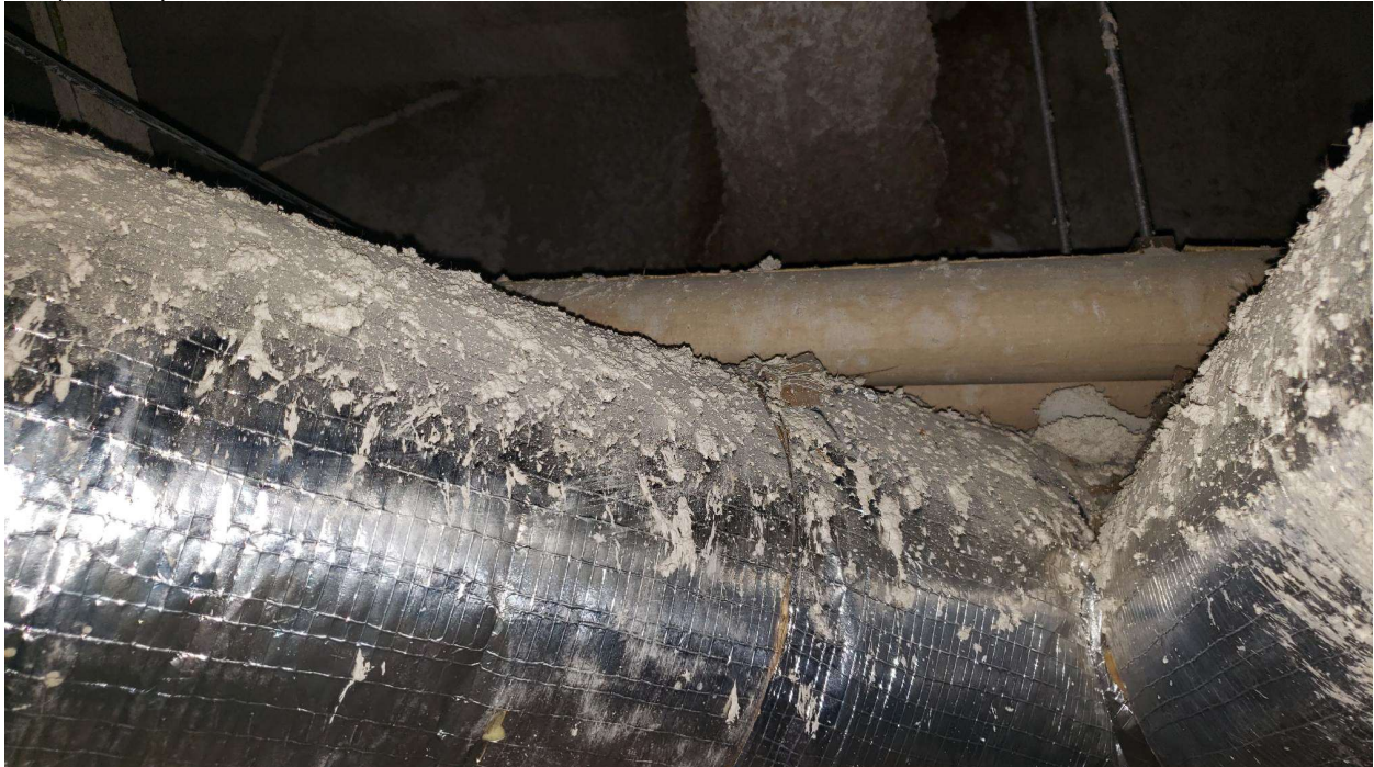
Photo 28: ACM spray on fireproofing overspray on ducting and pipe insulation.
