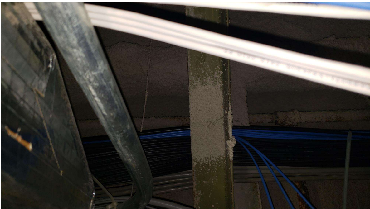
Photo 30: Cable bundles on top of ACM spray on fireproofing overspray.
