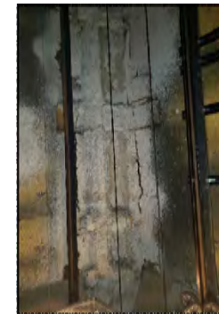
ELEVATOR 1/2: EXTENSIVE CRACKING OF ACM FIREPROOFING THROUGHOUT SHAFT
