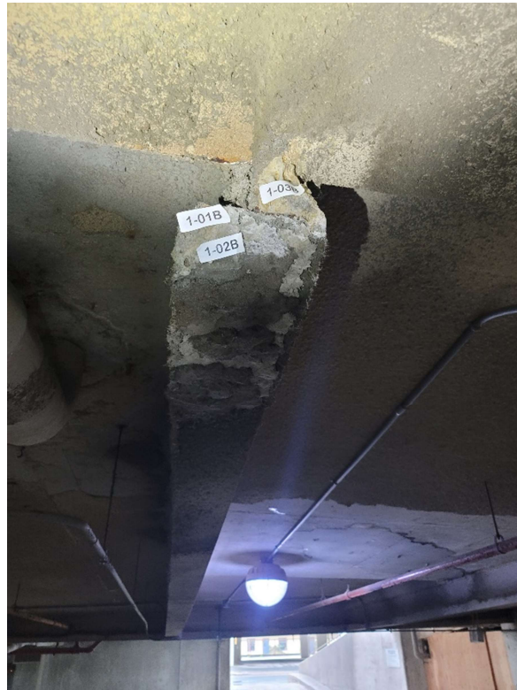
Photo 9: New fireproofing from 2 nd floor are 1-01B (white – standard spray pattern) & 1-03B (dark tan – standard spray patter)
