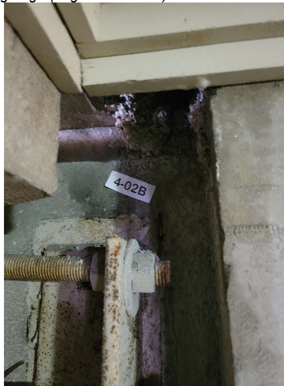
Photo 14: Gray fireproofing (above ceiling and at corner openings) – appears to be same spray as identified inside of the building on undersides of metal pan-decking (but is ND for asbestos)
