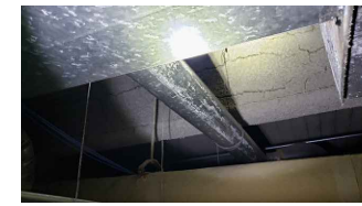
LOCATION 17: CRACKS IN ACM FIREPROOFING ALONG I-BEAM.
