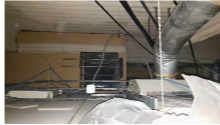
LOCATION 3: OVERSPRAY OF ACM FIREPROOFING ON TOP OF CEILING TILES. ACM FIREPROOFING IN GOOD CONDITION.
