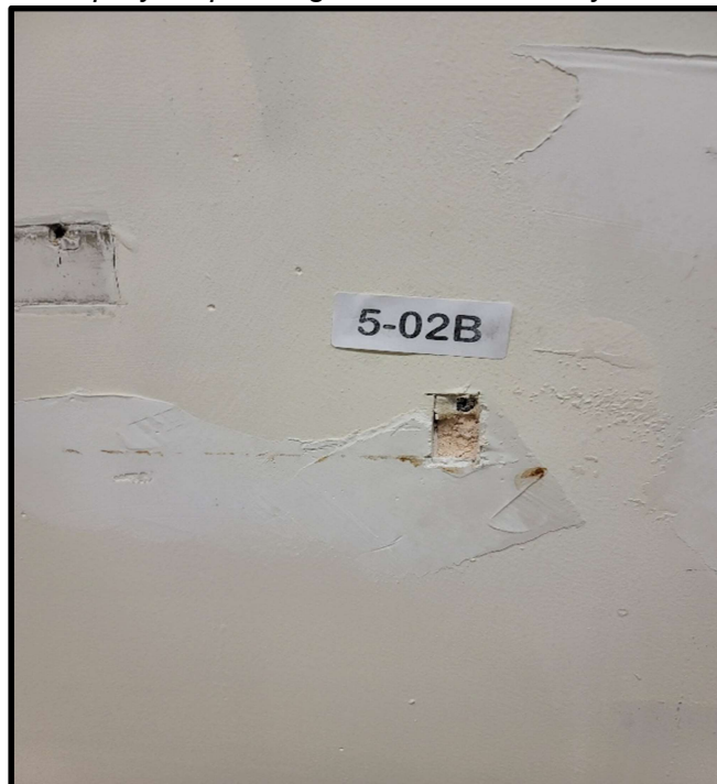
Photo 6: Asbestos containing joint compound patching applied to walls in 5 th floor Maintenance room. Joint compound patching applied to interior walls throughout building assumed to contain asbestos.
