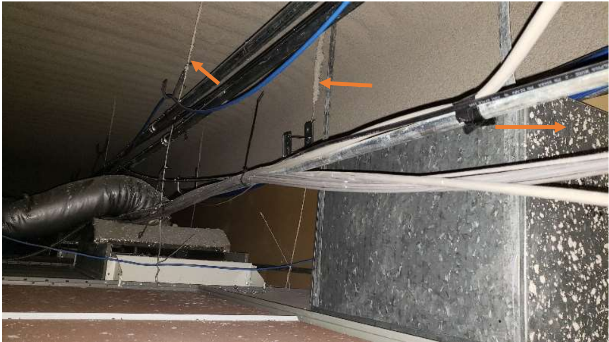
Photo 25: ACM spray on fireproofing on top of ceiling tiles. Note the spray on fireproofing on the pandecking above the tiles is in good condition. Note the overspray on the support wires and ducting (arrows).
