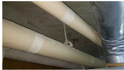
LOCATION 11: CRACKING/STAINING IN DAMAGED ACM FIREPROOFING ON PANDECKING.
