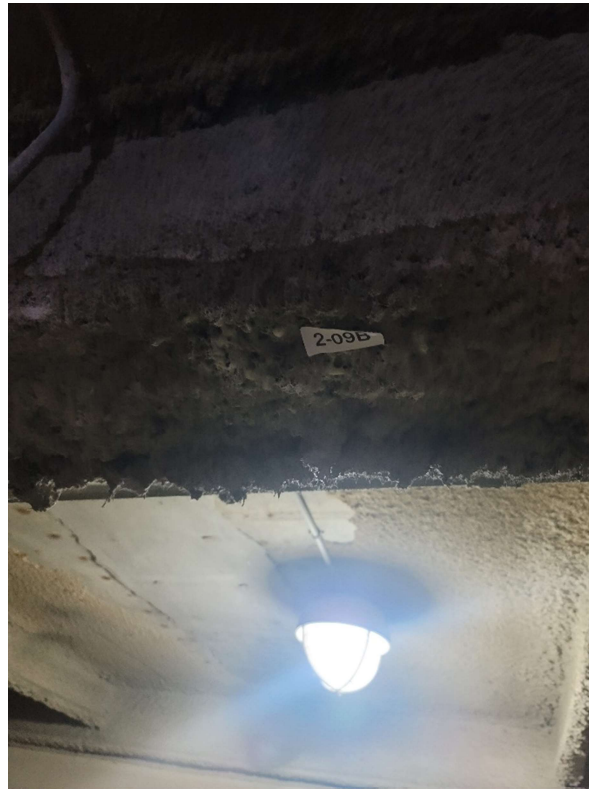
Photo 7: Dark gray fireproofing – fibrous – clumpy – semi-hardened
