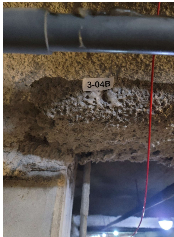
Photo 12: Off-white fireproofing (standard tan behind pipe) – standard spray pattern
