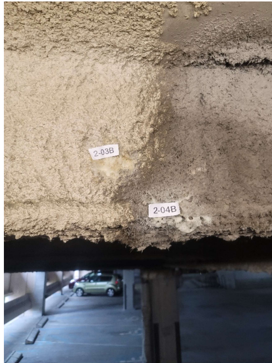
Photo 3: Off-white(left)/gray(right) fireproofing – standard spray pattern
