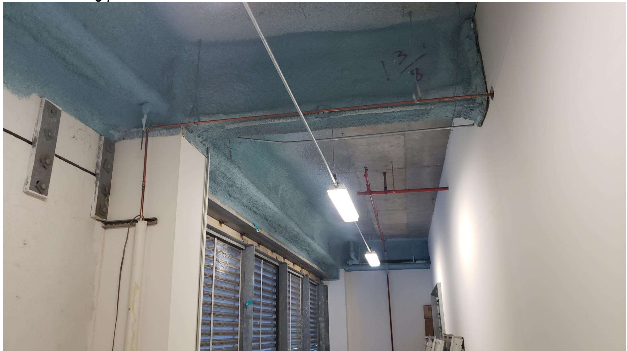
Photo 22: Air plenum and intake area. Note the spray on fireproofing has been abated and non-ACM fireproofing has been sprayed blue.
