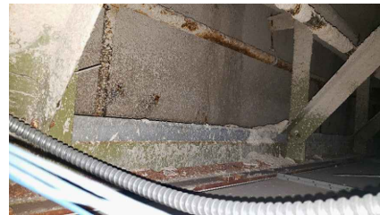
LOCATION 4: OVERSPRAY OF ACM FIREPROOFING ON TOP OF CEILING TILES. ACM FIREPROOFING IN GOOD CONDITION.
