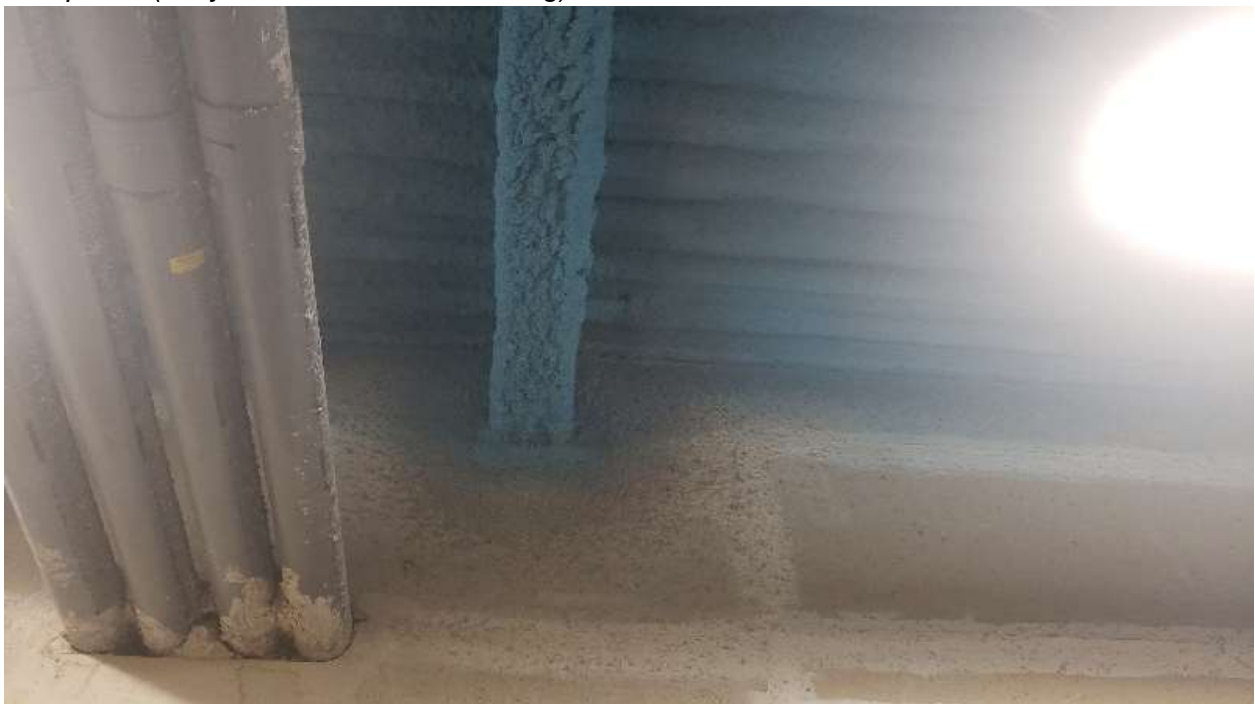
Photo 16: Typical Mechanical space present on Floors 5-7 depicting blue colored fireproofing on pan decking (non-asbestos containing) with gray fireproofing overspray on walls and piping (Chrysotile asbestos containing).
