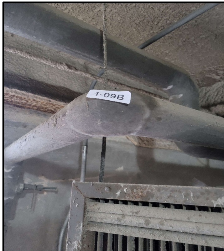
Photo 2: Pipe elbow containing 6% Amosite asbestos. Small diameter insulated piping sporadic throughout parking garages.
