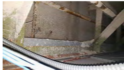
LOCATION 4: OVERSPRAY OF ACM FIREPROOFING ON TOP OF CEILING TILES. ACM FIREPROOFING IN GOOD CONDITION.
