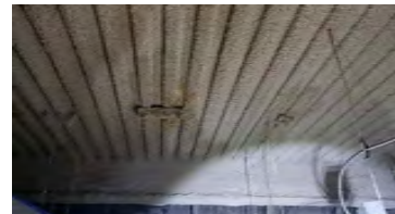
LOCATION 15: WATER STAINING AROUND ROOF PENETRATIONS.
