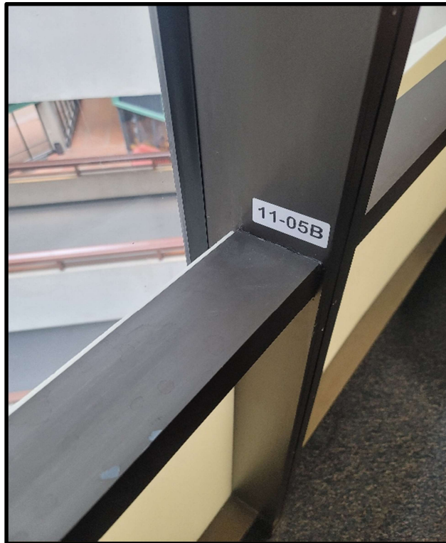
Photo 15: Black sealant at Atrium metal window supports contains 5.5% Chrysotile asbestos. Black sealant present at all visible seams for metal connections.
