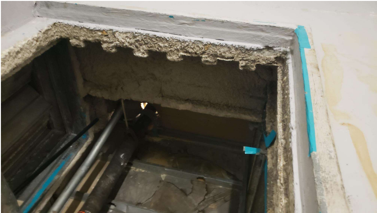
Photo 23: Opening in floor of sixth floor mechanical room, looking onto the pandecking above the fifth floor dropped ceiling. Although sixth floor mechanical areas have either been abated of ACM containing spray on fireproofing, or contain non-abated, but non-ACM spray on fireproofing, areas of the mechanical rooms may still be open to areas with ACM containing spray on fireproofing.
