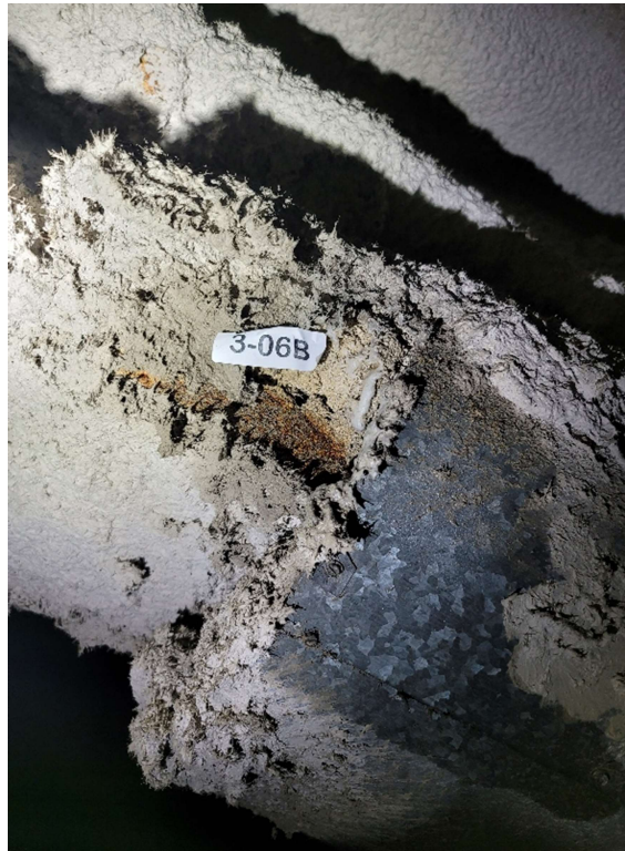
Photo 13: Beige fireproofing/insulation – visibly fibrous – inside metal clad cross brace members at edges of garage (large 3' diameter)
