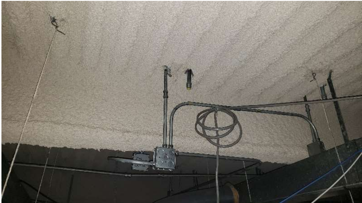
Photo 15: Typical light gray fireproofing on pandecking above dropped ceilings in office spaces (Chrysotile asbestos containing).
