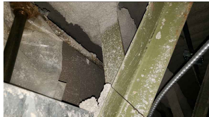
LOCATION 2: OVERSPRAY OF ACM FIREPROOFING IN CHANNEL IRON.
