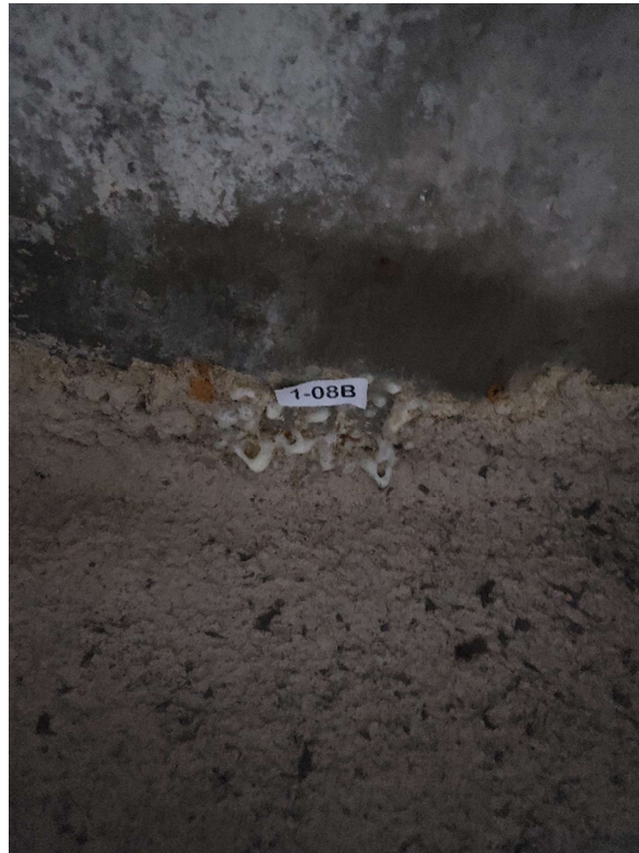
Photo 11: Slightly darker tan fireproofing – chunky/thick spray with white undercoat spray
