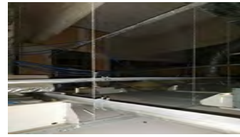
LOCATION 6: OVERSPRAY OF ACM FIREPROOFING ON TOP OF CEILING TILES. ACM FIREPROOFING ON PANDECKING IN GOOD CONDITION.
