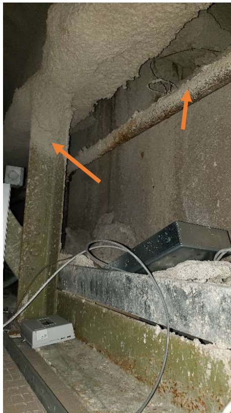
Photo 26: Fireproofing in channel iron on the concrete wall sill. Note the router placed on top of the ACM fireproofing and the overspray (arrows).
