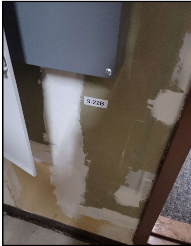
Photo 11: 9 th floor Mechanical room joint compound contains 3.5% Chrysotile asbestos. Joint compound present as wallboard seam sealant and patching.
