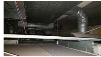
LOCATION 5: OVERSPRAY OF ACM FIREPROOFING ON TOP OF CEILING TILES. ACM FIREPROOFING ON PANDECKING IN GOOD CONDITION.
