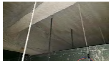
LOCATION 13: RUSTING AROUND BRACKETS. ACM FIREPROOFING NOT STAINED.
