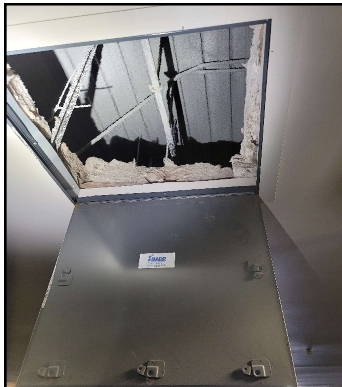
Photo 4: 4 th floor parking garage view above hard lid. Gray spray-on fireproofing present on pandecking consistent with rest of building. Assumed to contain chrysotile asbestos.
