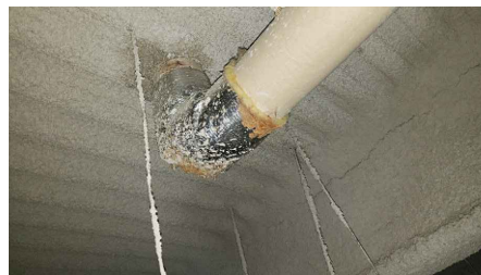
LOCATION 14: WATER STAINING NEAR PIPE PENETRATIONS IN PANDECKING.
