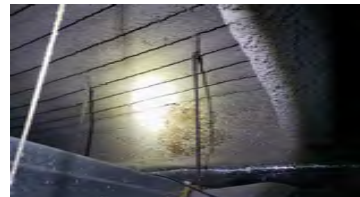
LOCATION 16: WATER STAINING ON I-BEAM WITH SUPERFICIAL CRACKS.
