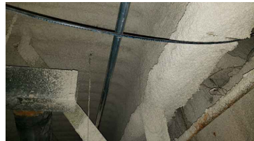
LOCATION 1: ACM FIREPROOFING ON PAN DECKING.
