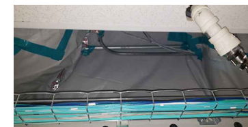
LOCATION 20: PLASTIC COVER OVER/AROUND FIRE SUPPRESSION GLOBE. ACM NOT VISIBLE. ASSUMED WATER DAMAGED.
