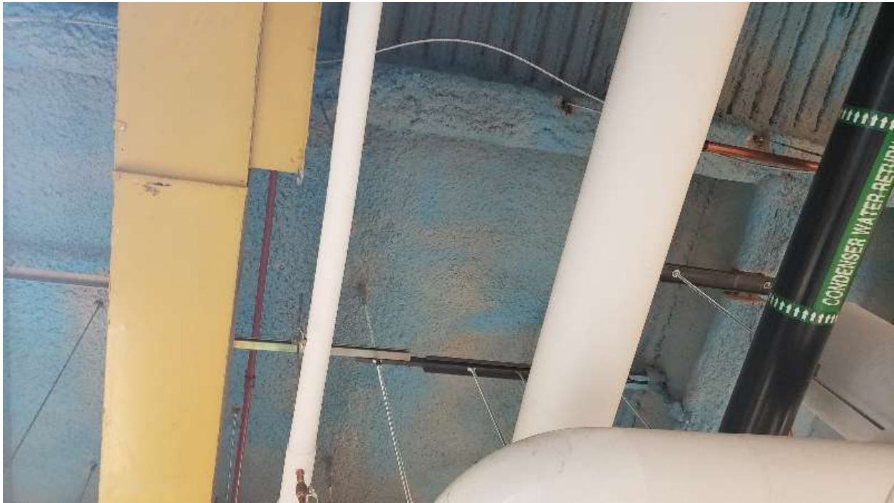
Photo 17: Blue, non-asbestos fireproofing. Note the inconsistent color, probably stemming from insufficient mixing of dye within the fireproofing batch.
