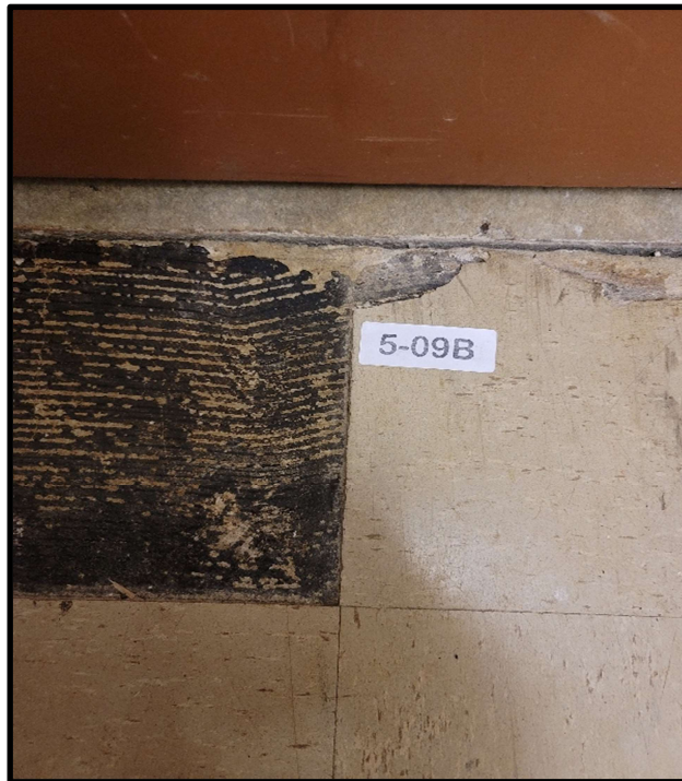
Photo 7: 5 th floor office building server room entry floor tiles and black mastic both contain Chrysotile asbestos. Floor tiles brittle and damaged.
