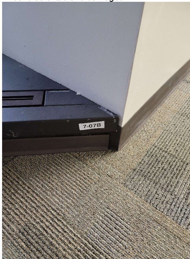
Photo 8: Light tan mastic behind brown cove base contains 2.5% Anthophyllite asbestos.
