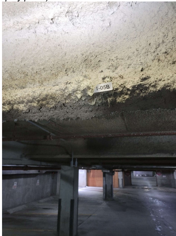
Photo 10: Gray fireproofing – visibly fibrous overspray pattern
