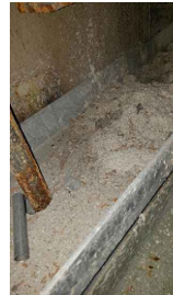
LOCATION 22: OVERSPRAY OF ACM FIREPROOFING IN CHANNEL IRON. ACM FIREPROOFING ON PANDECKING IN GOOD CONDITION.
