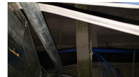
LOCATION 24: OVERSPRAY OF ACM FIREPROOFING IN CHANNEL IRON AND ON TOP OF CEILING TILES. CABLE BUNDLES STRUNG OVER SUPPORTS HAVE ACM FIREPROOFING ON THEM, DAMAGING THE ACM.
