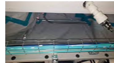
LOCATION 20: PLASTIC COVER OVER/AROUND FIRE SUPPRESSION GLOBE. ACM NOT VISIBLE. ASSUMED WATER DAMAGED.
