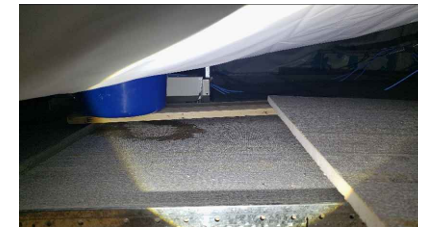
LOCATION 18: ASSUMED WATER DAMAGE. ACM FIREPROOFING NOT VISIBLE DUE TO PLASTIC CATCHMENT.
