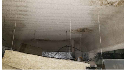
LOCATION 8: WATER STAINED/DAMAGED SPRAY-ON ACM FIREPROOFING.
