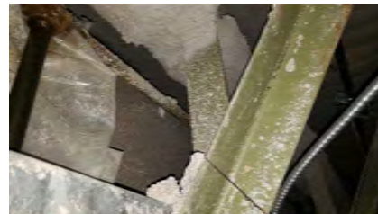
LOCATION 2: OVERSPRAY OF ACM FIREPROOFING IN CHANNEL IRON.
