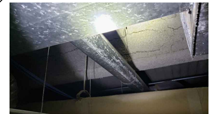
LOCATION 17: CRACKS IN ACM FIREPROOFING ALONG I-BEAM.
