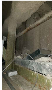
LOCATION 1: OVERSPRAY OF ACM FIREPROOFING IN CHANNEL IRON.
