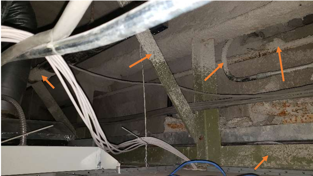
Photo 27: Fireproofing in channel iron on the concrete wall sill. Note the overspray areas (arrows)
