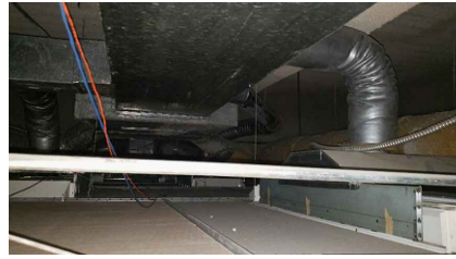
LOCATION 5: OVERSPRAY OF ACM FIREPROOFING ON TOP OF CEILING TILES. ACM FIREPROOFING ON PANDECKING IN GOOD CONDITION.
