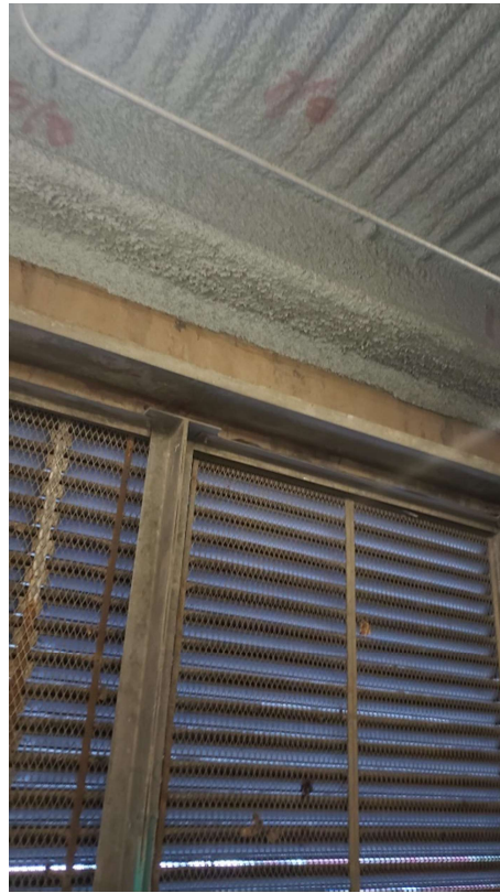
Photo 19: Blue, non-asbestos fireproofing in the air intake plenum. Note the blue color is consistent, but light colored.
