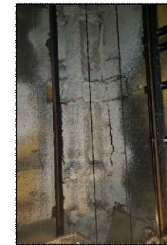
ELEVATOR 1/2: EXTENSIVE CRACKING OF ACM FIREPROOFING THROUGHOUT SHAFT
