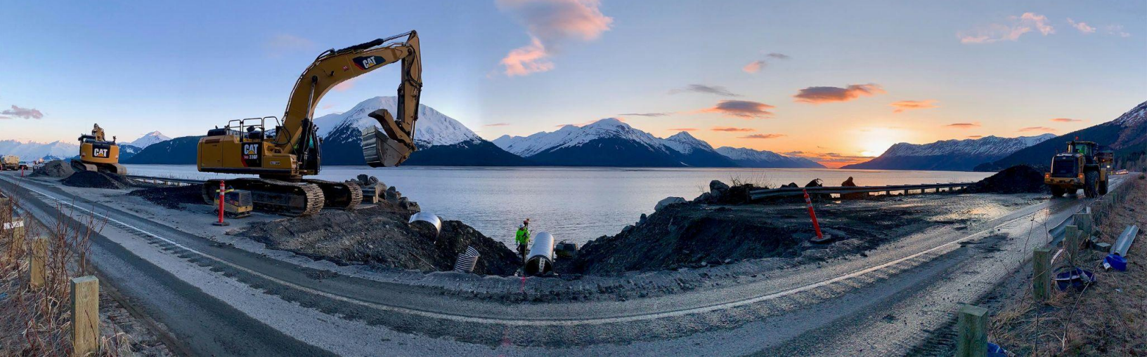
Seward Highway MP 75-90 Road and Bridge Rehabilitation project, April 2019. Ted Meyer, Alaska DOT&PF
