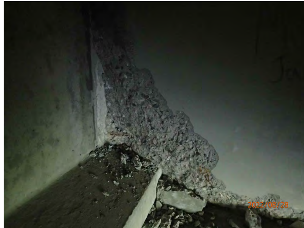
ABUTMENT I BAY 14 SPALL No Scale
