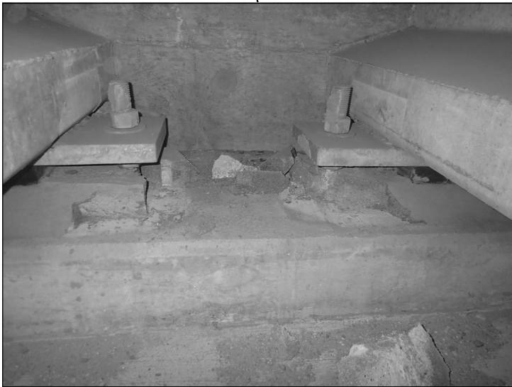
TYPICAL GROUT PAD SPALLING
