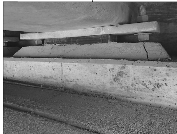
TYPICAL GROUT PAD SPALLING
