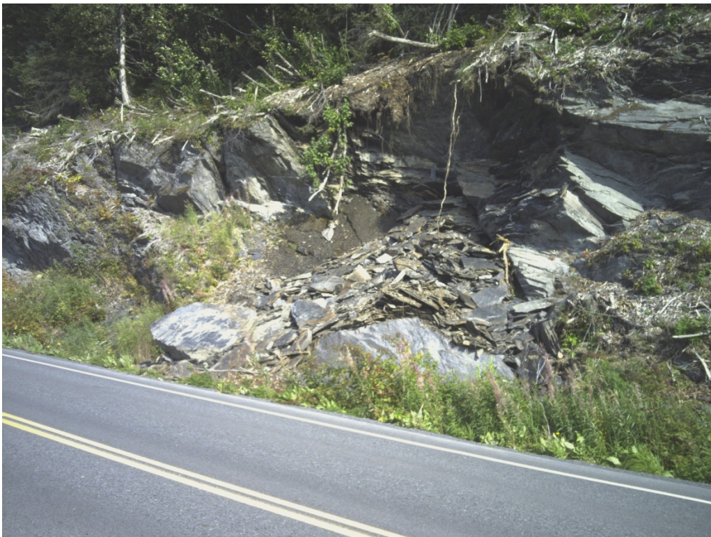
Rock fall at MP 18.5, September 2014
