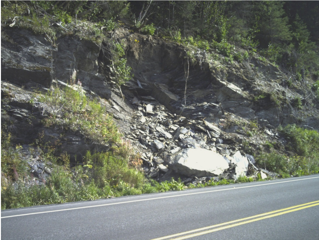
Recent rock fall September 2014 at MP18.5 Seward Highway, facing south
