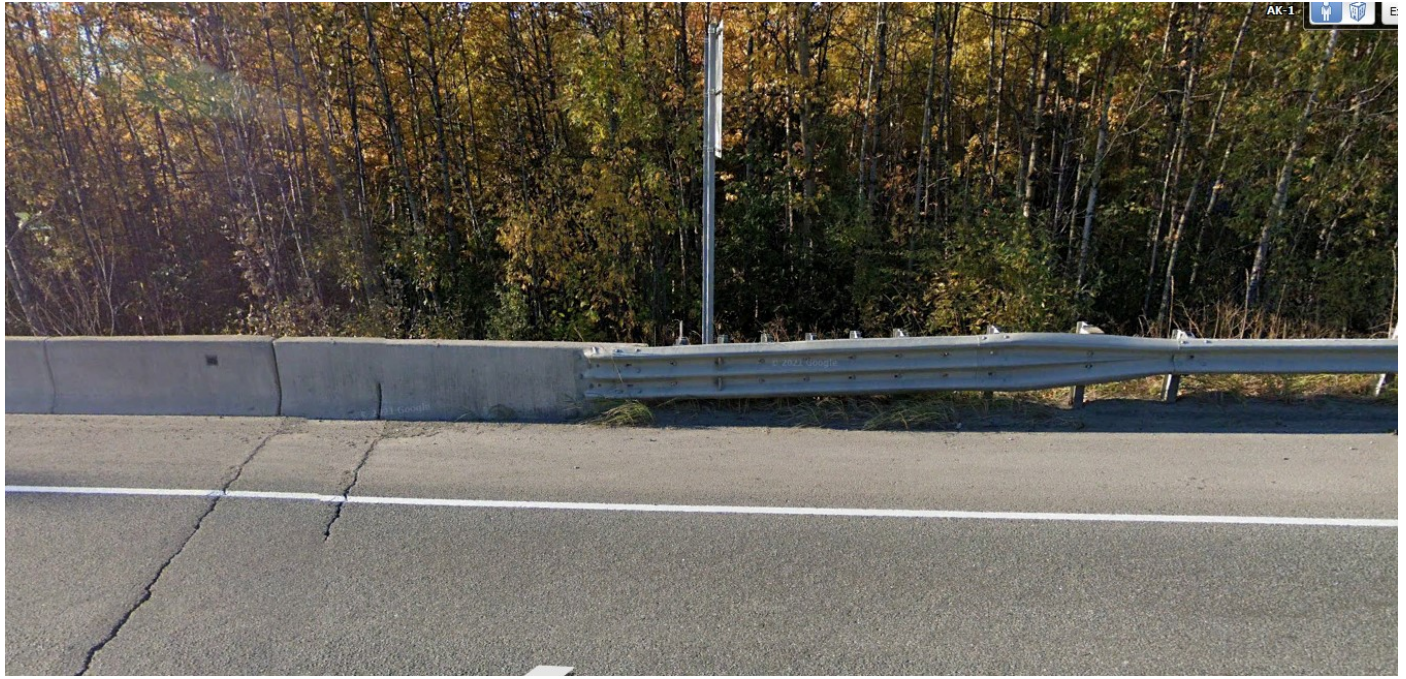
Modified Steel Post Thrie Beam Transition height difficulty to Concrete Barrier
