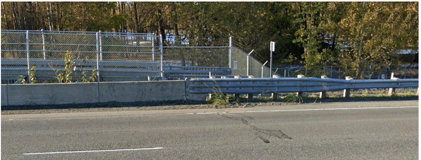
Older Wood Post Thrie Beam Transition to 32" concrete barrier
