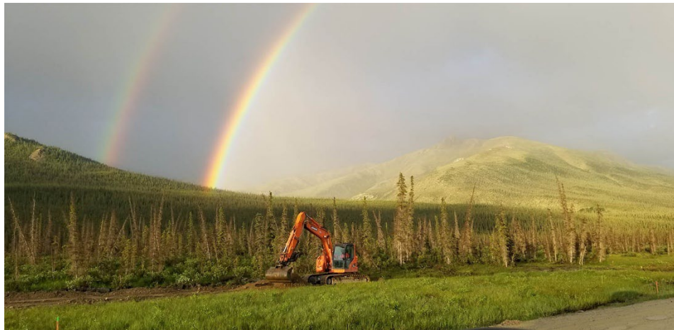
An excavator fills in the fiber optic trench along the Dalton Highway MP 210, Summer 2018. Photo By Henri Barnes, Alaska DOT & PF
