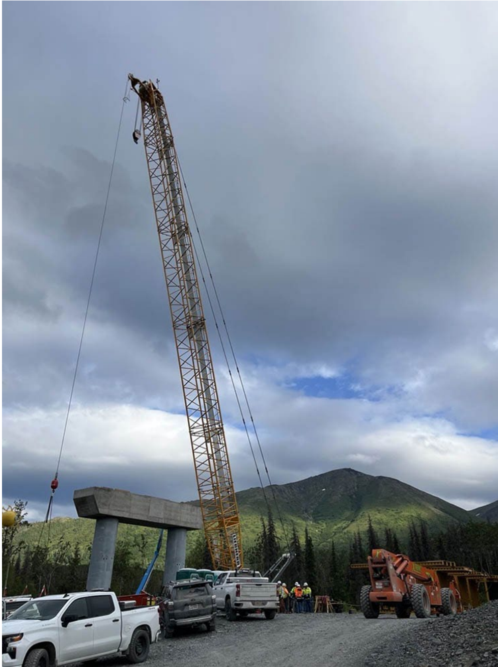
Project CFHWY01060: Sterling Highway MP 45-60 Juneau Creek Bridge Sage 2 CM/GC Photo by Zhenioa Peterson, Alaska DOT & PF
