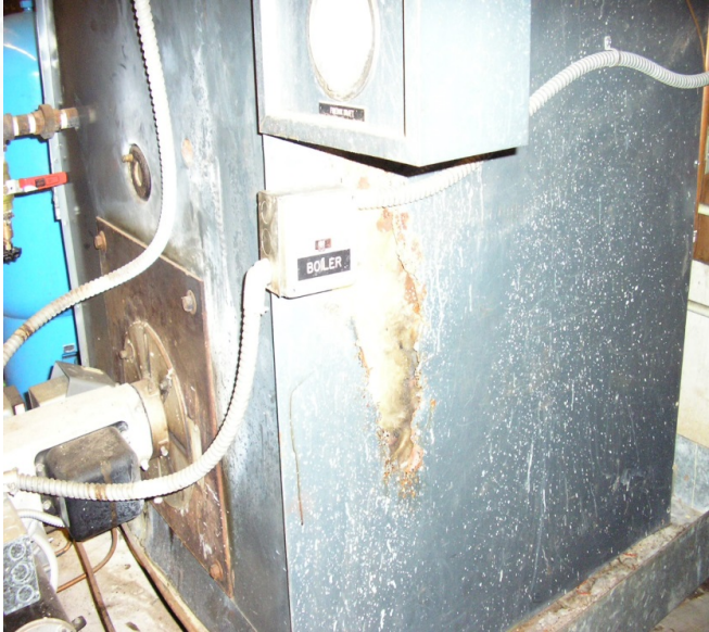
Wornout and rusting mechanical system
