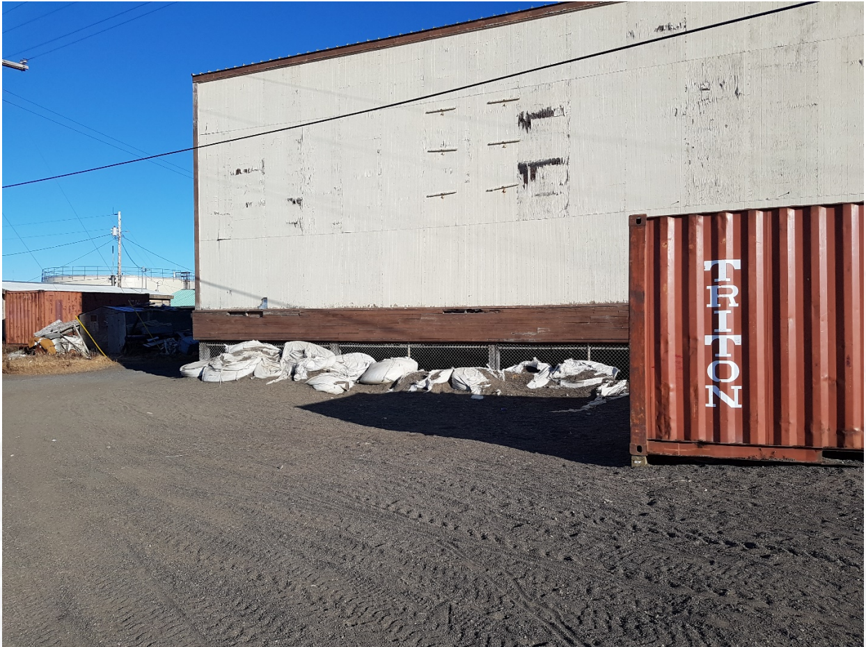
Failed siding and structural support. Note sand bags to prevent erosion of the foundation.
