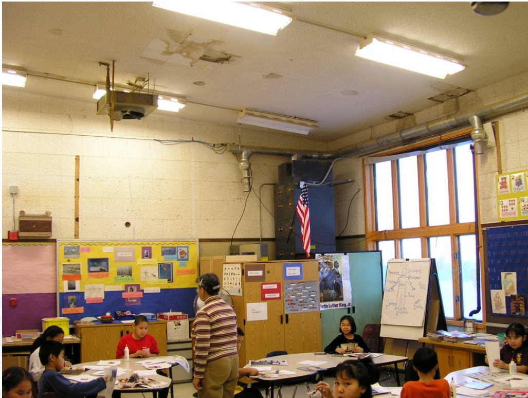
Former Voc Ed Classroom with ceiling unit heater, remnants of dust collector, water damaged ceiling, inadequate lighting, marginal electric and data support, flip chart for teaching wall.
