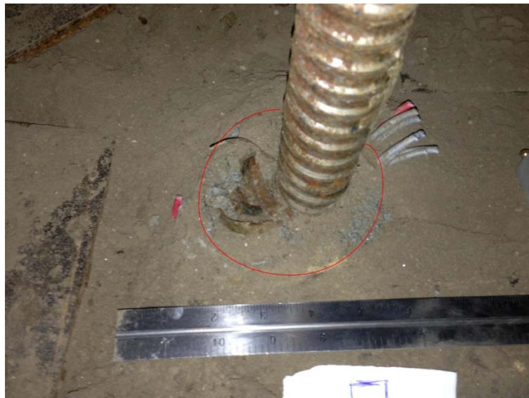
Figure 5.28 Anchor 4 After Failure
