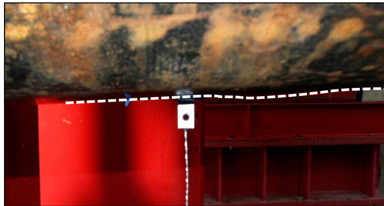
Figure 3-44: Buckling initiated under pile during the first pull of ductility three
