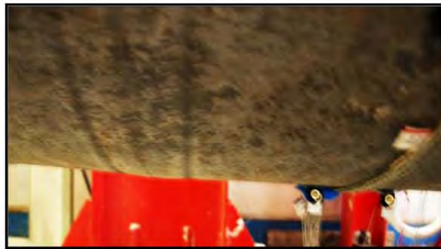
Figure 3-137: Tension cracks observed on the underside of the pile, ductility 4, \Delta=11.2 in
