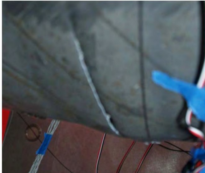
Figure 3-97: Rupture on underside of pile, \Delta = 8.98 in
