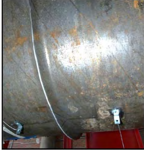
Figure 3-164: Crack on underside of the pile closing, first pull of ductility 5, \Delta=11.5 in
