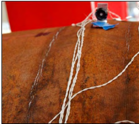
Figure 3-62: Tension cracking during the third pull, at 11 inches displacement, approaching the 13 inch displacement at ductility 4
