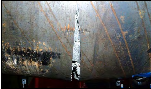
Figure 3-162: Concrete has not crushed under the buckle ductility 5, \Delta=11.5 in
