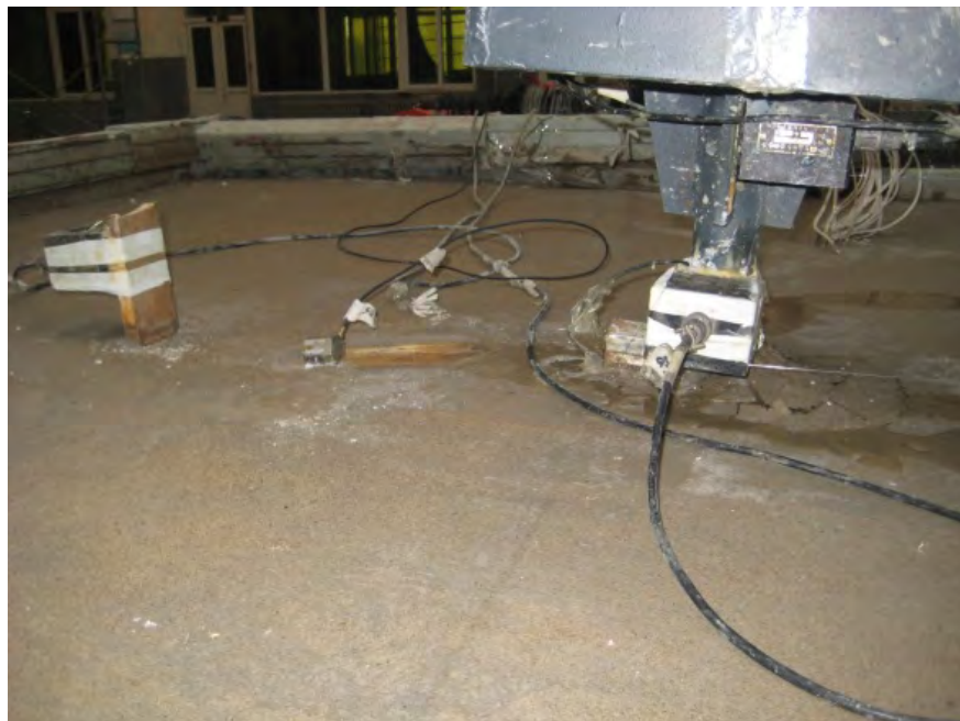
Figure 2.17. Tilted pile head
