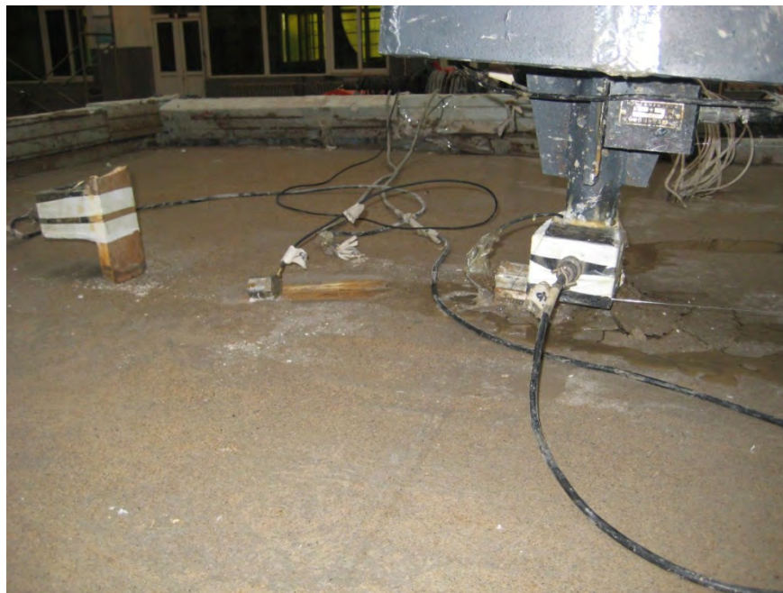
Figure 2.15. Cracks formed near the soil-pile interface
