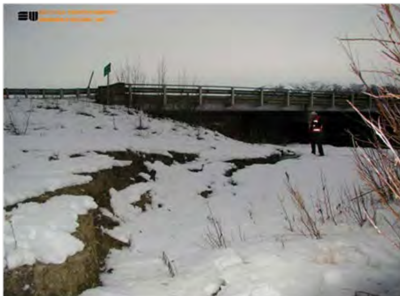
Figure 1.4. Lateral spreading observed in a bridge site after the 2002 Denali earthquake
