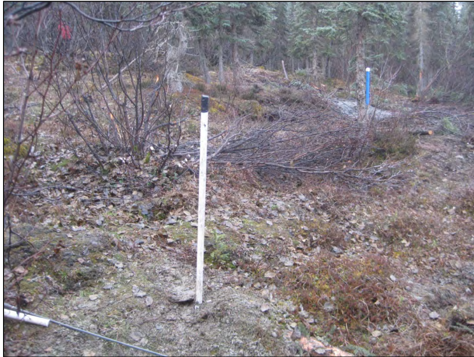
Figure B-3. Completed casing installations for TH12-9006 in the foreground and TH12-9000 in the background to the right. This photograph is taken to the south; the Dalton Highway is to the right of the photograph, and the toe of FDL-A is to the left. (Photograph by M. Darrow)
