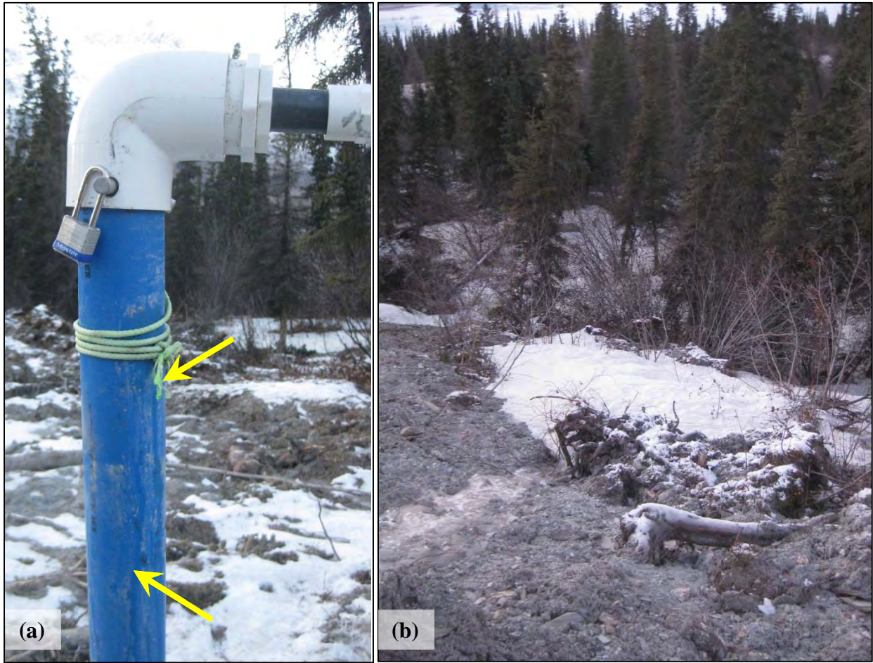
Figure 26. Evidence of groundwater flow at FDL-A. (a) Propylene glycol overflowing the top of the slotted casing in TH12-9004 drips from the M-IPI safety line and runs down the outside of the casing (indicated by arrows). (b) Ice formed along the toe of FDL-A; the Dalton Highway is visible near the top of the photograph. (Photographs by M. Darrow)
