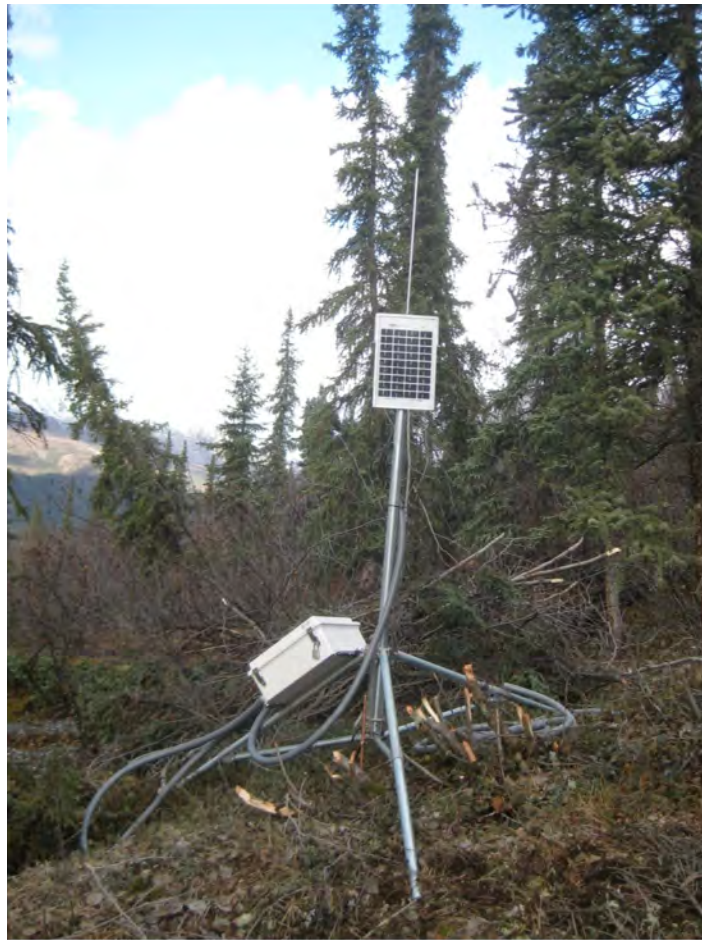
Figure B-11. Completed “lower” satellite ADAS installation. TH12-9005 is located beyond the brush behind the ADAS in the photograph. (Photograph by M. Darrow)
