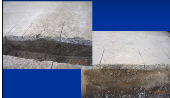
Parks Hwy MP 325-351 After foaming - Oct.2005 Blisters Cross-sectional view of affected area
